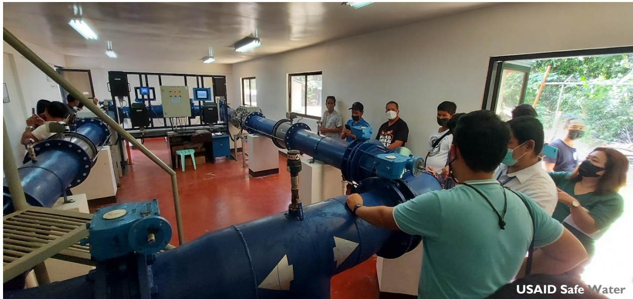
Inside the infiltration gallery of Puerto Princesa City Water District's Ultraviolet Hydro Optic Disinfection System in Barangay Irawan, Puerto Princesa City.
