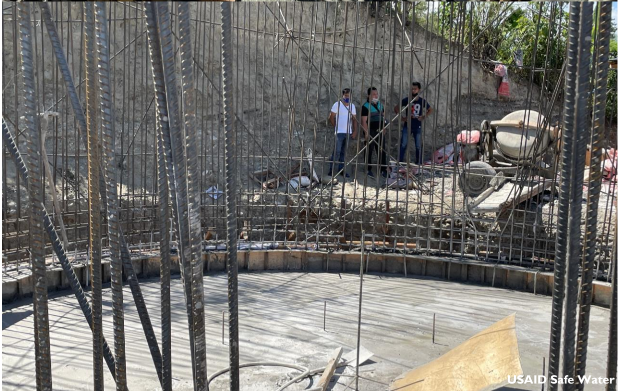
Following the Safe Water training on project proposal preparation, the Team is supporting the development of a small water impounding structure in Malapatan for funding from the grant program of the National Task Force to End Local Communist Armed Conflict.
