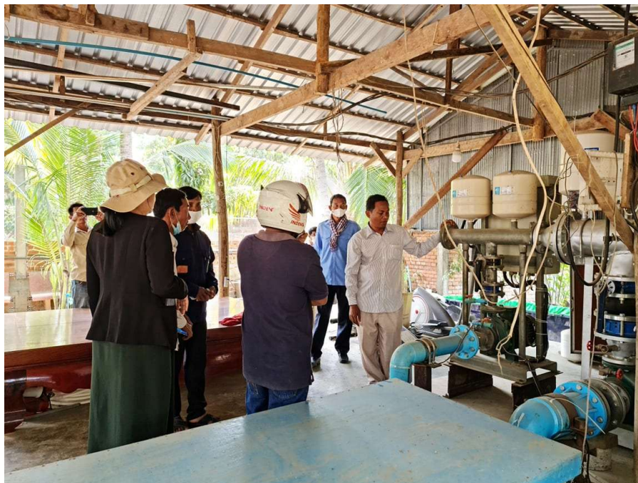
Photo 1. WASH-FIN organized a community water tour of the Svay Romeit water company facility
