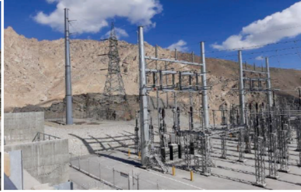
Photo #6: A-006_General overview Salang Tunnel Substation, Parwan Province. SS, 2020-10-14.
