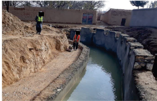
Photo #7: A-007_Backfilling behind canal lining at station 0+370 to 0+390 RS, Kohna Aybak Canal, Samangan Province. MHM, 2020-11-27.
