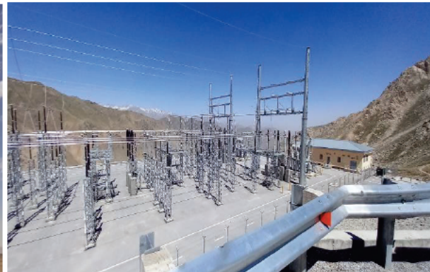
Photo #4: A-006_General overview, Salang Tunnel Substation, Parwan Province. MJR, 2021-06-15.
