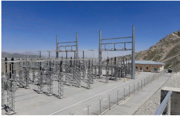
Photo #5: A-006_General overview, Slang Tunnel Substation, Parwan Province. MM,2021-06-16.
