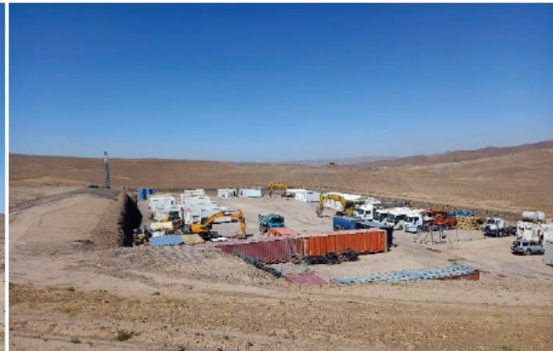
Photo #24: A-017_Live support area and turbine foundation excavation, Robate Sangi District, Herat Province, NAA, 2021-09-12.
