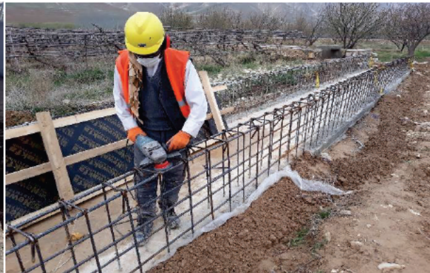
Photo #8: A-007_RCC lining rebar rust cleaning station 0+580 to 0+600, Asya Abad Canal, Samangan Province. MY,2021-03-15.
