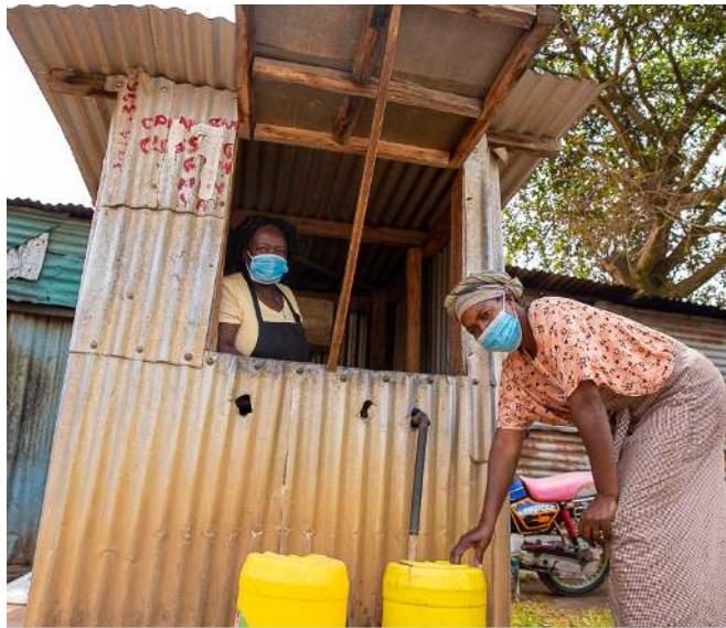
The installation of solar panels has ensured reliable water services to the community and reduced operational costs.
