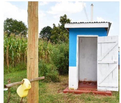
A SAFI latrine constructed at a health facility to arouse community's interest.
