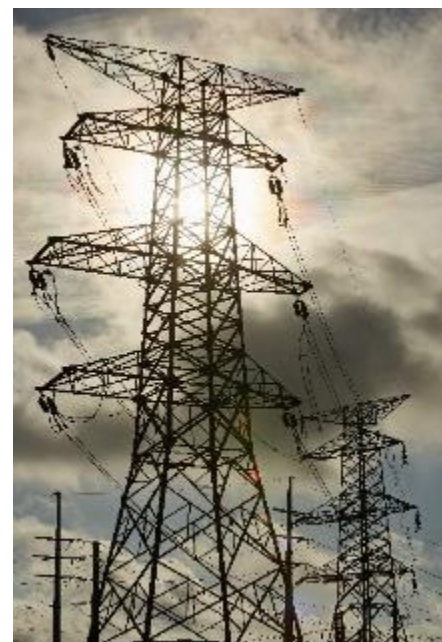
Figure 4: Camama Substation and in Luanda, Angola. Photo Credit: USAID SAEP
