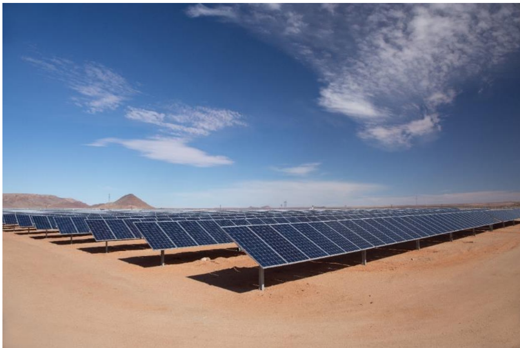
Figure 15: PV panels at the Aggenys solar plant in the Northern Cape. South Africa plans to solve the country’s power crisis by generating electricity through a mix of sources, with renewable energy accounting for a large portion of it. Photo Credit: USAID SAEP
