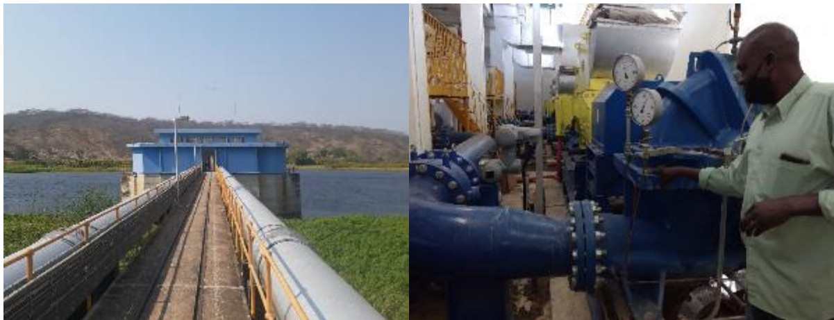
Figure 17: The LWSC Iolanda water treatment plant on the Kafue River supplies Lusaka with water. Photo Credit: USAID SAEP.
