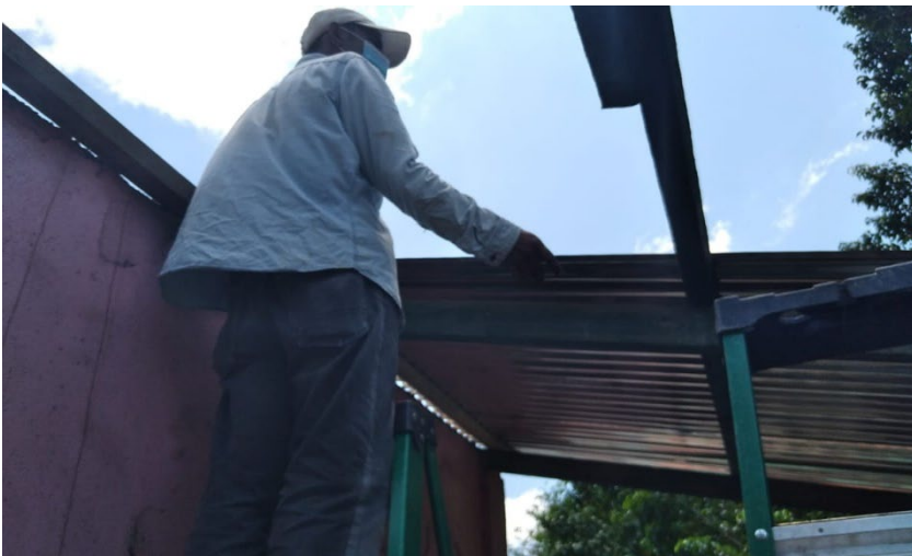
Figure 1. Shelter repairs in Brisas del Milagro community in the municipality of Villanueva.
