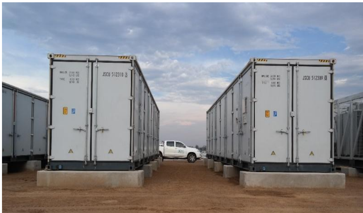
The 20 MW Golomoti Solar PV and Battery Energy Storage Project will pioneer utility-scale battery energy storage. Photo credit: JCM Power
