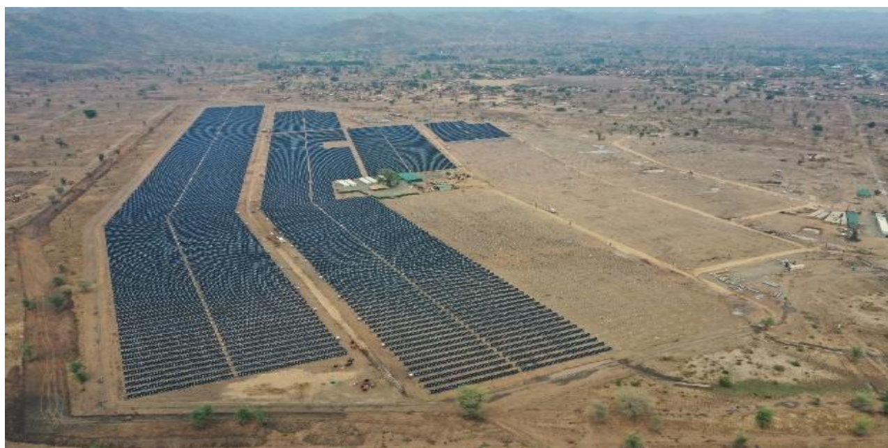
The 20 MW Golomoti Solar PV and Battery Energy Storage Project site is located in Dedza, about 100 kilometers southeast of Lilongwe. Photo credit: JCM Power
