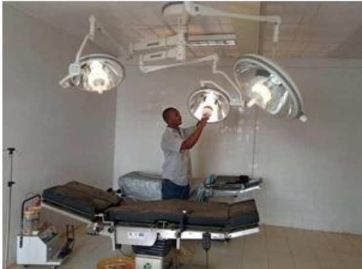
Photo: Project driver installing an operation room light, Laska PHL, Basketo Special Woreda
