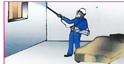
STEP 5: Windows and doors will be closed, and the operator will be alone in the structure during the spray
