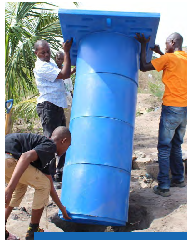
In Ghana, a family works together to install their new Digni-Loo. The entire installation process only takes about 10 minutes. Photo credit: Melissa Burnes, USAID/WASH for Health
