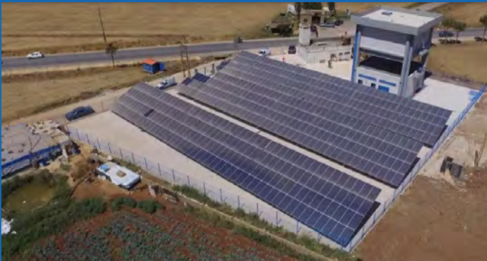
Aerial photo of the Ghazzeah Pumping Station with the 174 Kwp solar farm. Photo Credit: USAID/Lebanon Water Project
