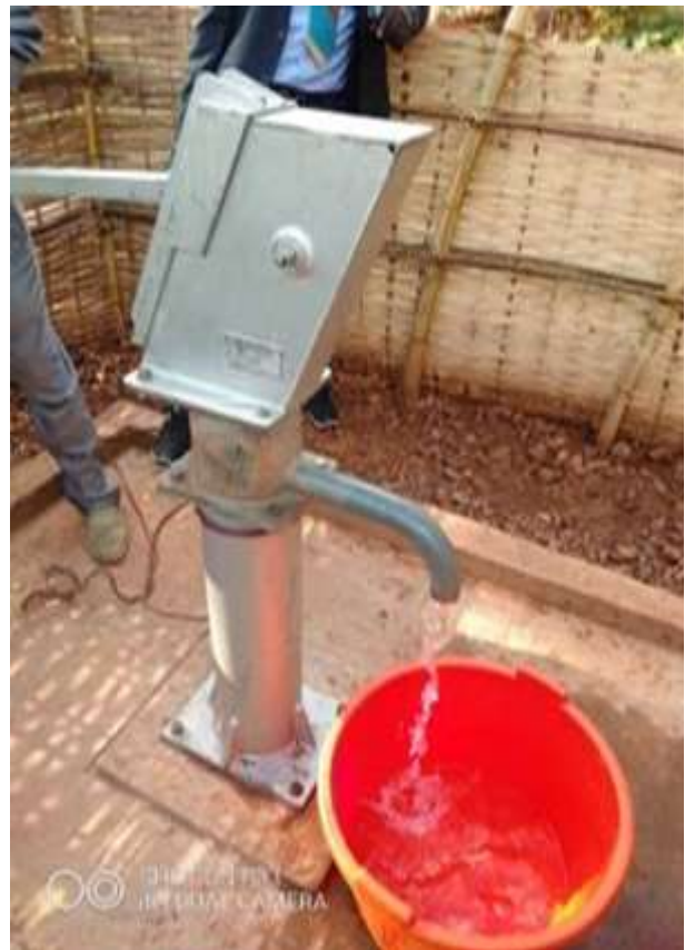
HYDRO INDIA 60 pump in Tshitshimu
