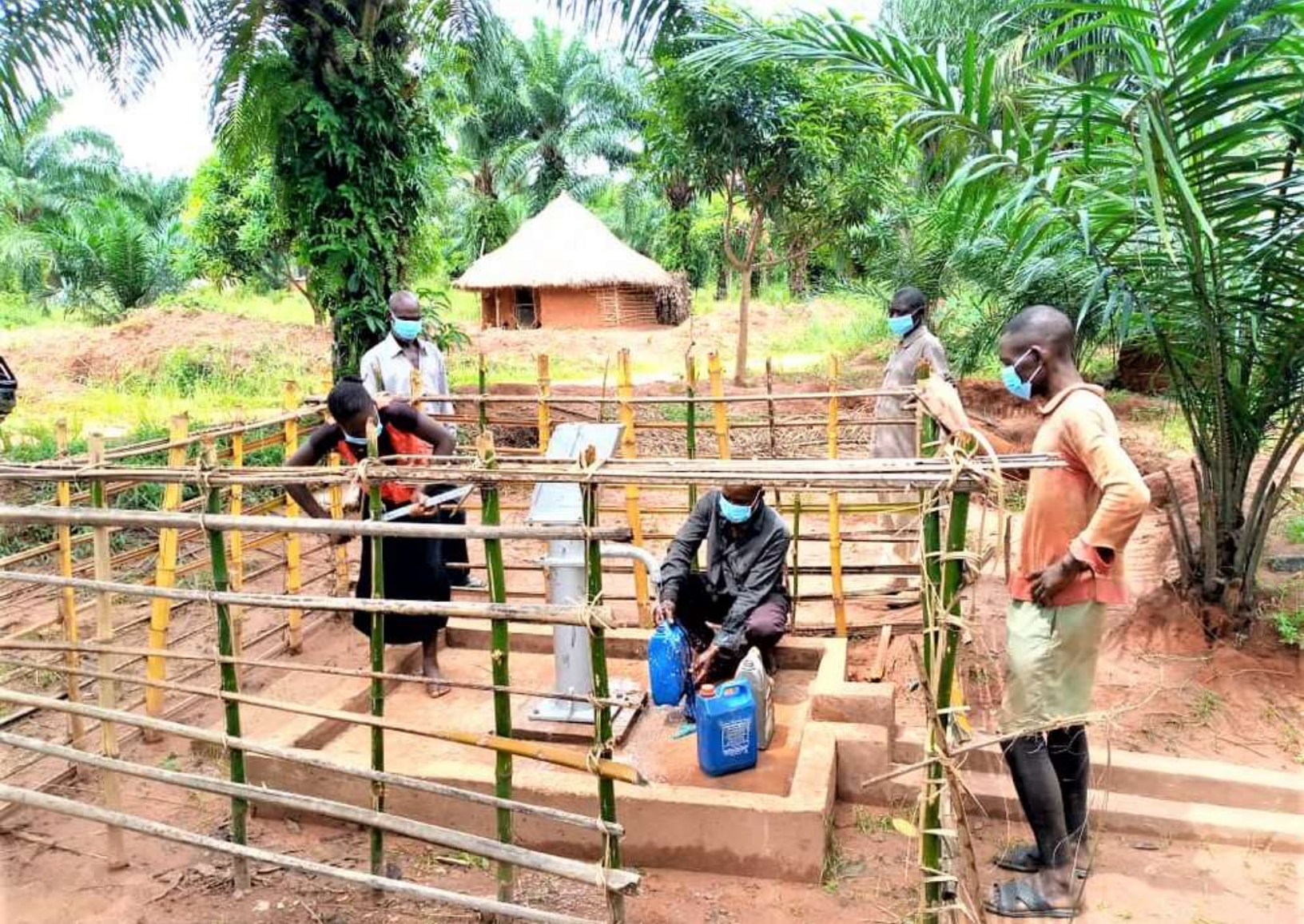
Installation of a standpipe in Kasansa ZS, Kasai-Oriental. Photo by Michel Dibwe, Abt Associates for USAID IHP.
