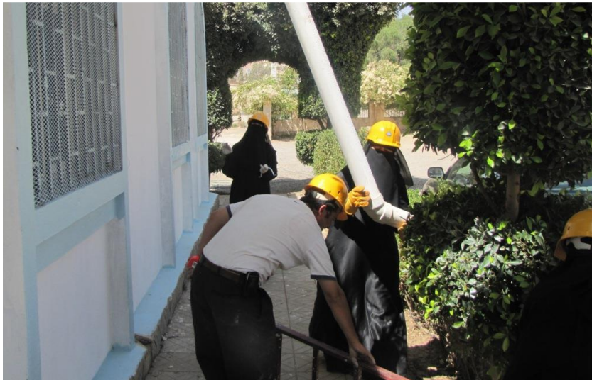
Peer Network members develop rooftop rainwater harvesting installations to direct rainwater to gardens at the only operational female MoYS club, Bilquis Club in Sana’a.
