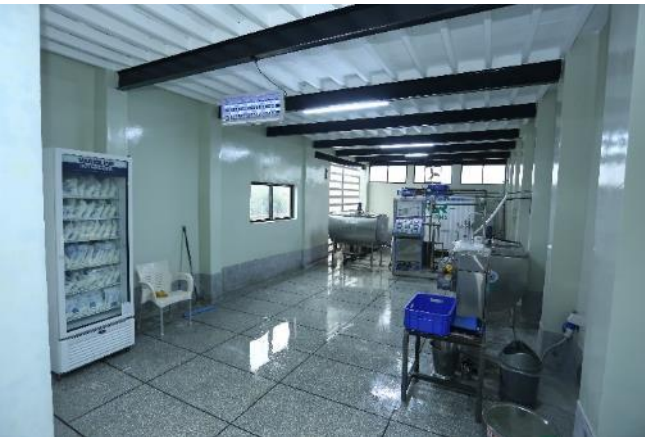
After – Neat and clean milk pasteurization facility at GR Farms after complete construction of the shed and installation of the PEEP-supported milk pasteurizing equipment – Photo by USAID PEEP
