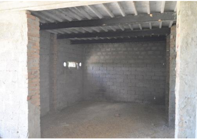
Before – Unfinished shed as part of matching grant contribution by GR Farms for PEEP-supported milk pasteurization facility before installation of the equipment – Photo by USAID PEEP
