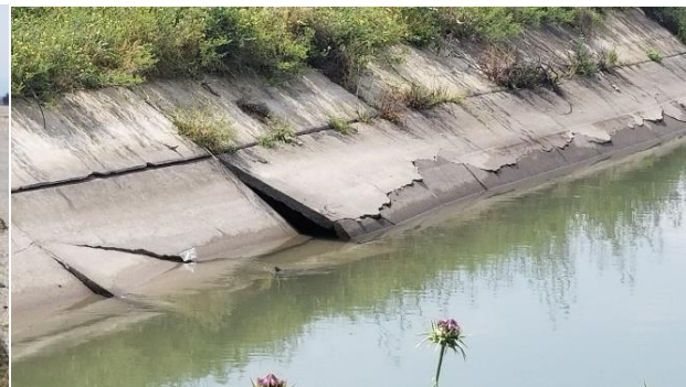
Figure 5: Damage to KAC Lining
