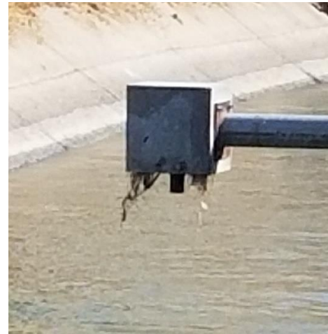
Figure 26: A KAC SCADA Stage Sensor Contaminated with Debris
