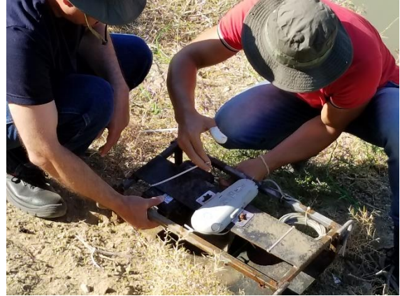
Figure 13: Preparing the SonTek IQ for Deployment in its Custom-Designed Frame, October 2017
