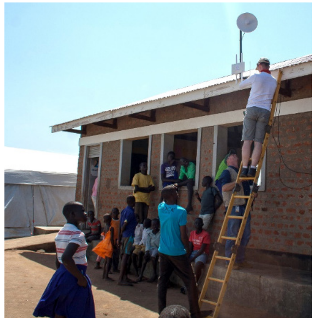
Network technicians installing broadband hardware at a field office of a USAID implementing partner in Uganda.
