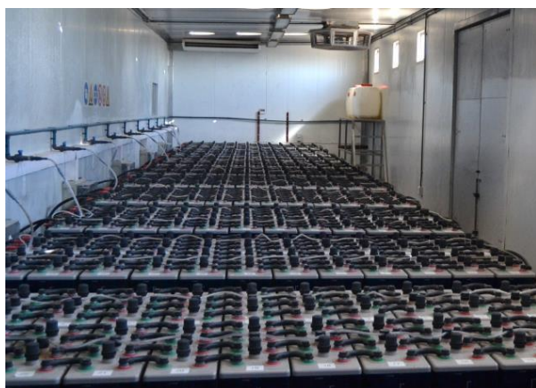
SAEP provides support in analyzing the potential use of battery storage to manage solar variability and reduce energy costs for electricity distributors. Photo: SAEP
