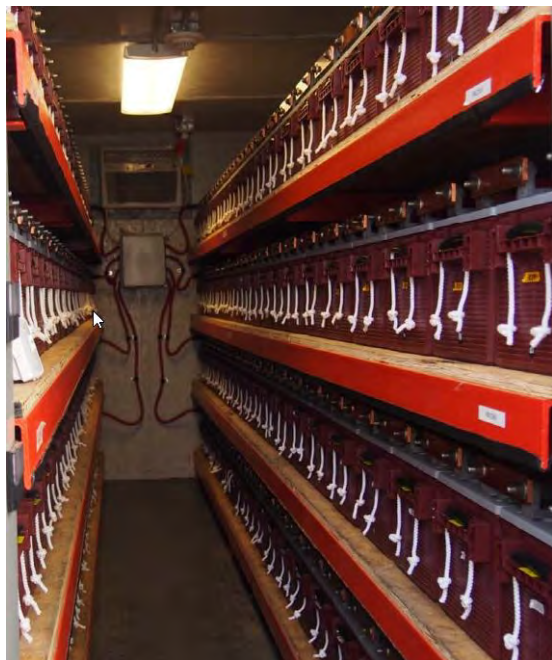
Figure 5.9 Battery bank for mini-grid in Les Anglais, Haiti.
