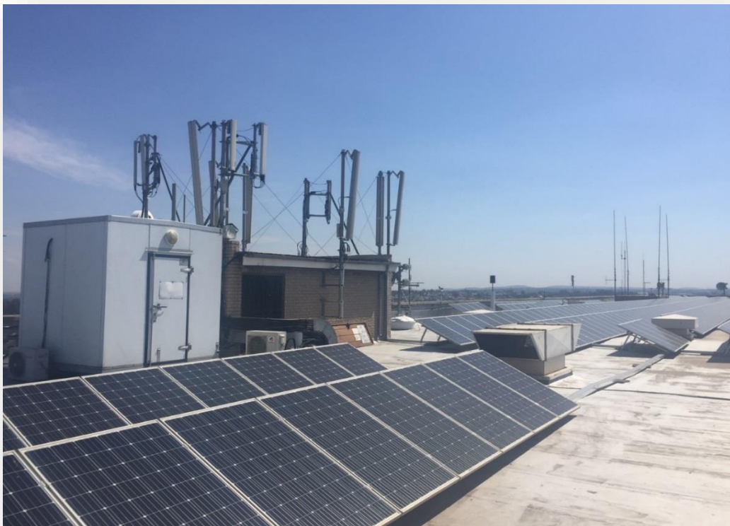
Figure 7 Solar PV Installation at Ekurhuleni Metropolitan Municipality Office
