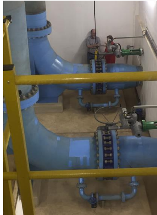
Photo 2: The inside of the plant at Ashley Drive
