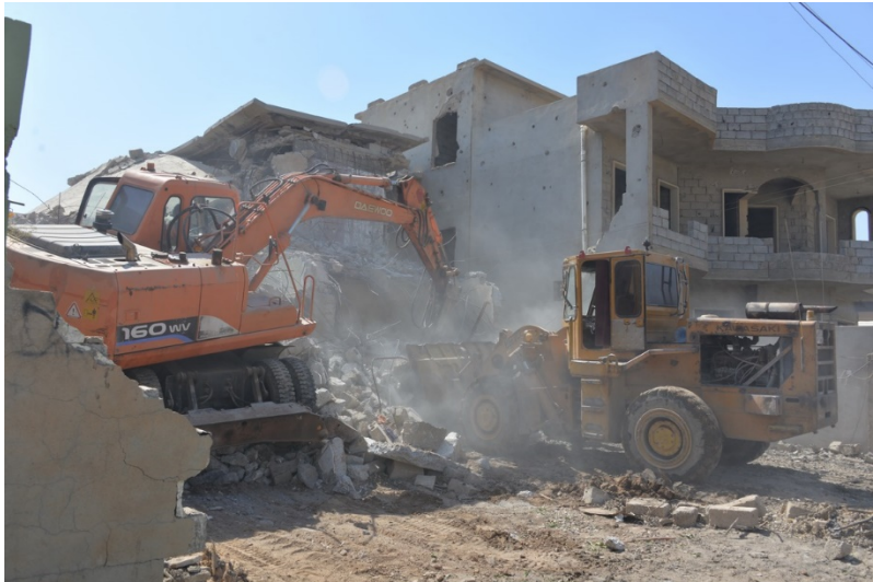
Rubble is cleared from houses that were damaged during the ISIS occupation and subsequent battle for liberation. (Credit: ICRI Field Program Assistant)
