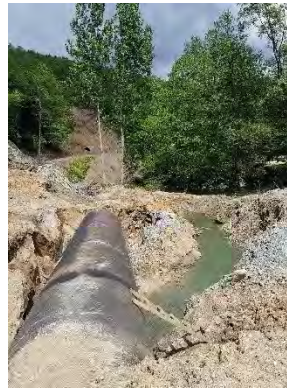
(Photo 4, left). Road construction at the Decani Plave/Plava road in Bjeshtë Nemuna/Prokletije National Park, in part upgraded to serve the Lumbardhi hydropower plants)
