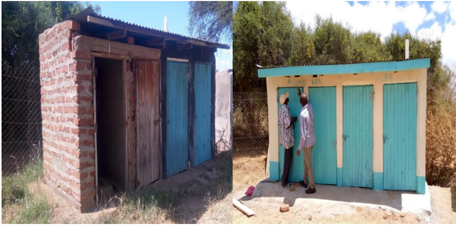
A latrine block at Itoleka Dispensary before and after renovation in Kitui Central sub-county
