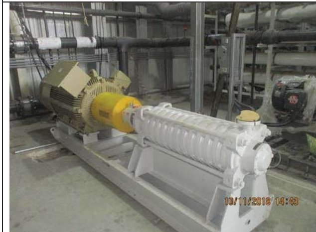
Photo No.05: High pressure pumps arrival Date: November 10, 2018
