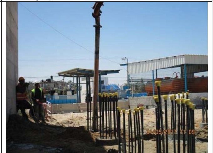
Photo No.16: Casting piles at the new RO building area. Date: May 31, 2017
