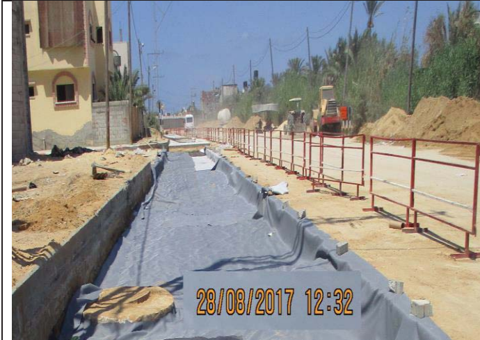
Photo No.67: Surface restoration work at paved concrete road (filter fabric installation). Date: August 28, 2017
