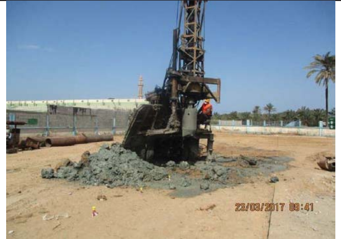
Photo No.24: Excavation for 600mm diameter pile (R08, Type- L, Depth- 16 lm).
