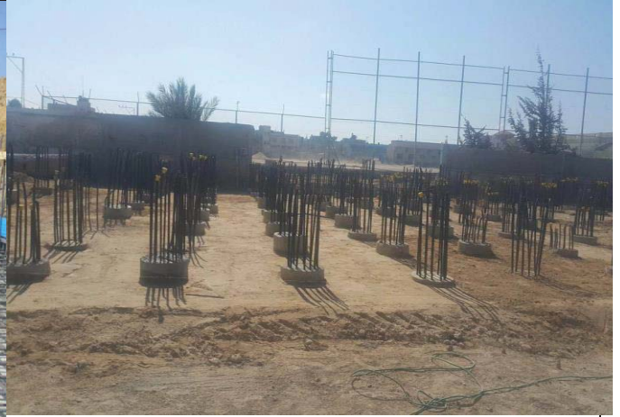
Photo No.10: Pre-treatment building leveling works prior to mud mat works Date: October 7, 2017
