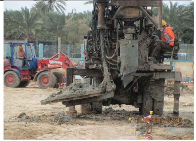
Photo No.12: Pile construction activity at the new pre-treatment building area. Date: April 10, 2017
