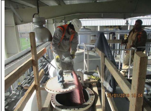
Photo No.19: Garnet filling inside DMF tanks Date: January 25, 2019
