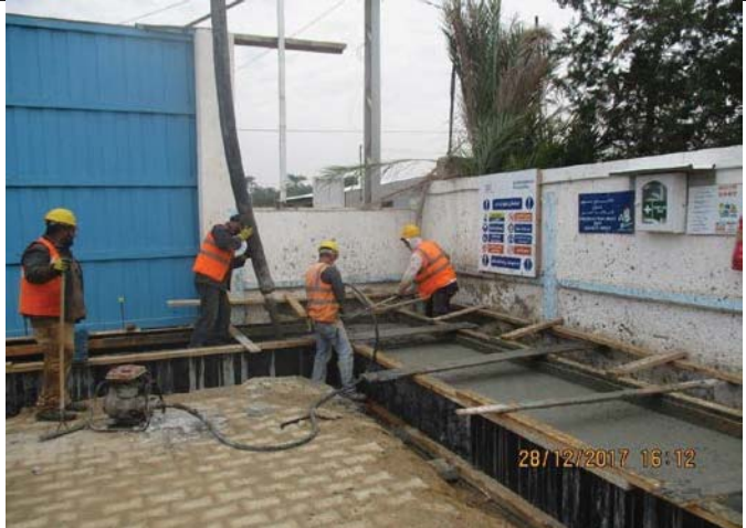
Photo No.51: Casting concrete for the workshop area ground beams Date: December 28, 2017
