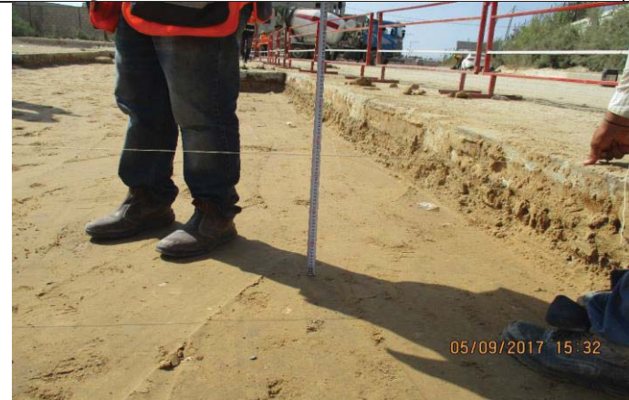
Photo No.05: Surface restoration work at paved concrete road compacted levels control Date: September 5, 2017
