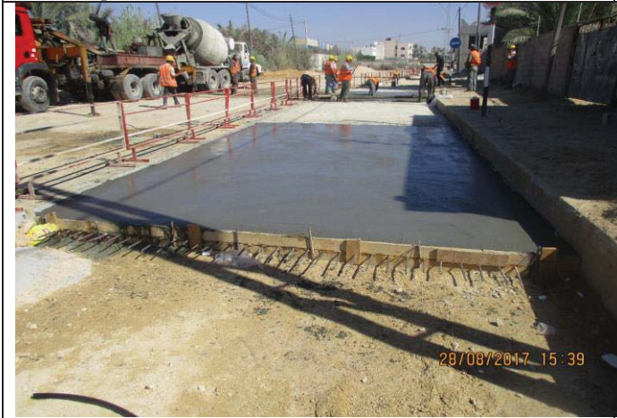
Photo No.69: Surface restoration work at paved concrete road (surface restoration). Date: August 28, 2017
