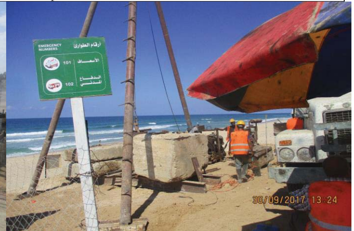
Photo No.36: Beach wells drilling activity (proposed beach well No. 02) Date: September 30, 2017
