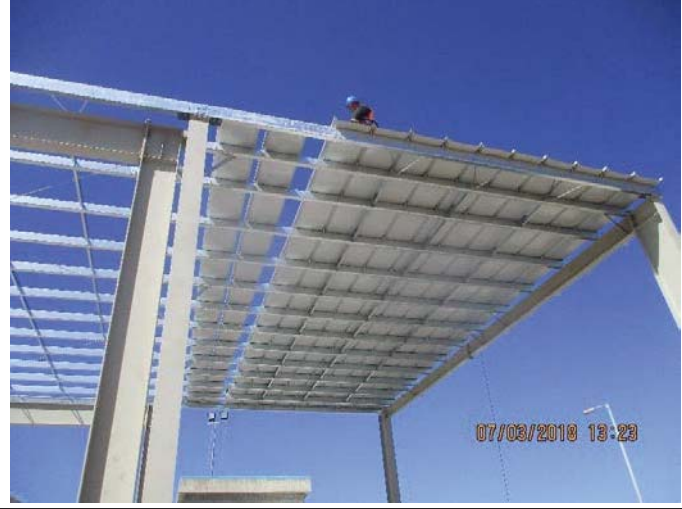
Photo No.06: Start installation for roof panels of generator pad steel structure Date: March 07, 2018
