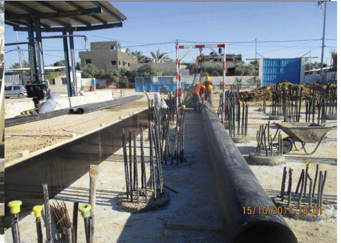
Photo No.30: Welding HDPE pipes 450 mm for intake pipeline up to pre-treatment building. Date: October 15, 2017
