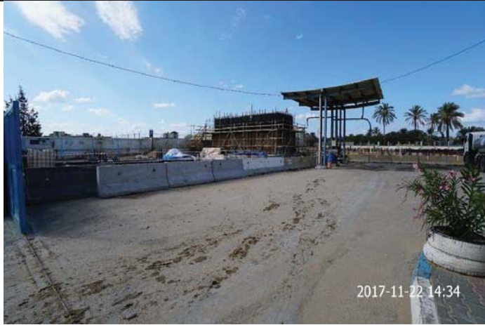
Photo No. 29: Site securing, concrete barriers installation and warning signs installation. Date: November 22, 2017
