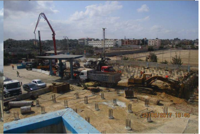
Photo No.34: Pile construction activity (raw water and backwash tanks) & brine excavation Date: September 23, 2017
