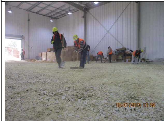
Photo No.05: Leveling and compaction works for the base course layer inside workshop area. Date: January 05, 2019
