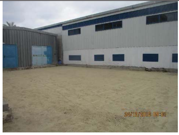
Photo No.22: Compaction works for the base course layer in site yard Date: December 24, 2018
