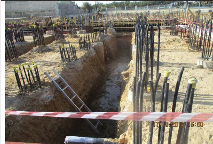
Photo No.33: RO building activities – trench excavation for PVC drainage pipes. Date: October 17, 2017
