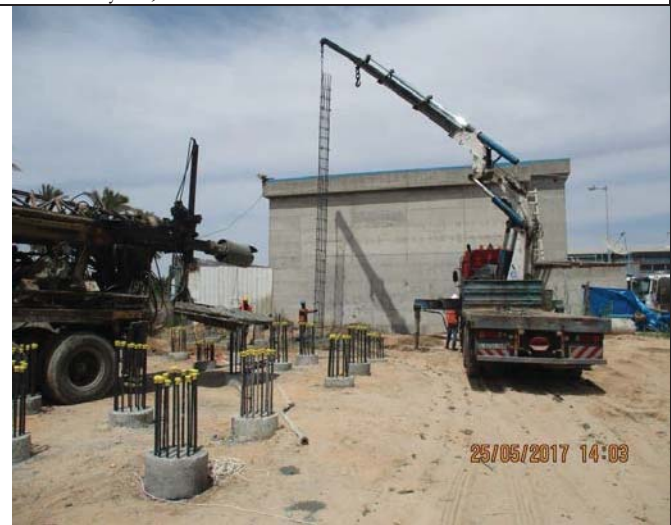
Photo No.10: Drilling and concrete reinforcement activities for the new RO building piles construction. Date: May 25, 2017
