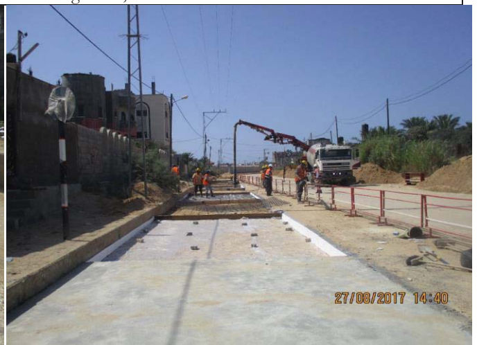
Photo No.66: Surface restoration work at concrete paved road (concrete pouring). Date: August 27, 2017
