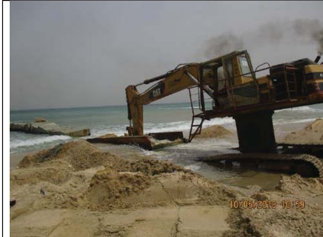
Photo No.13: Start dismantling works for all materials used in outfall pipeline installation Date: May 10, 2018
