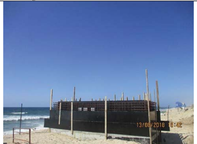
Photo No.18: Second face formwork for second part of beach well No. 1 retaining wall Date: August 13, 2018
