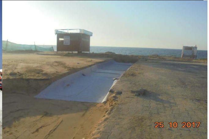
Photo No.48: RO building activities – trench excavation for PVC pipes. Date: October 25, 2017
