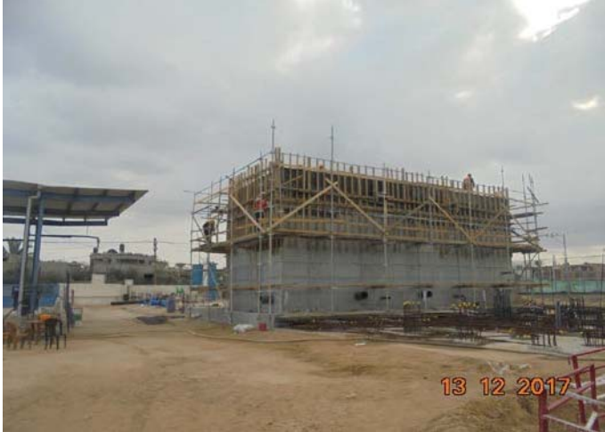
Photo No.27: Raw water and backwash tanks forming, steel reinforcing works for slab casting. Date: December 13, 2017
