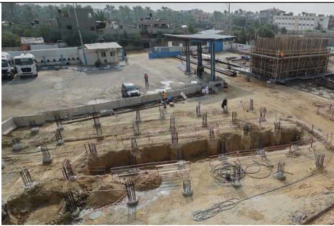
Photo No. 27: Generator pad trench works suspended due to heavy rain. Date: November 21, 2017
