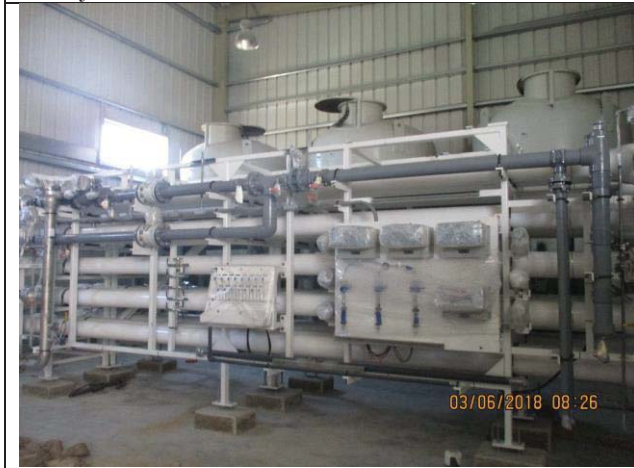
Photo No.03: Installing of 2 nd Pass RO skid unit-2 in place. Date: June 03, 2018
