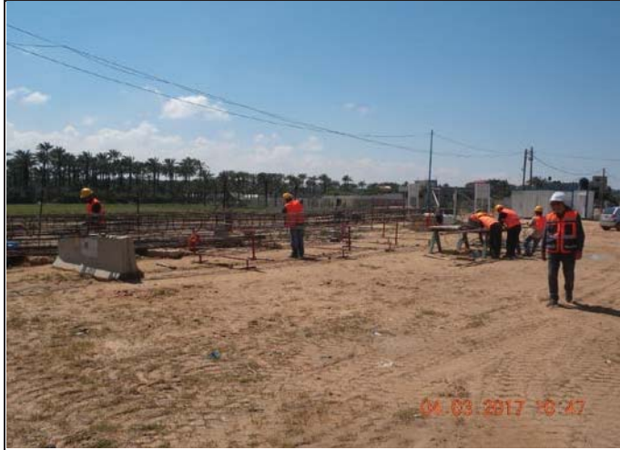
Photo No.01: Fabricating reinforcement steel case for piles at storage yard. Date: April 03, 2017
