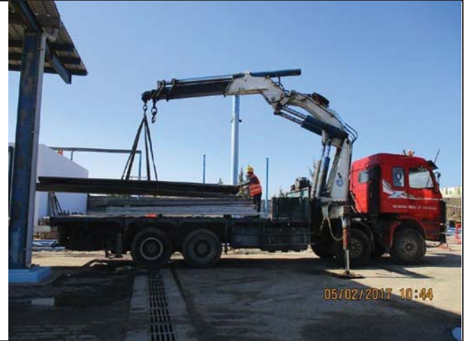
Photo No.06: Continue transferring materials from the steel canopy structure & interlocks to CMWU stores.
