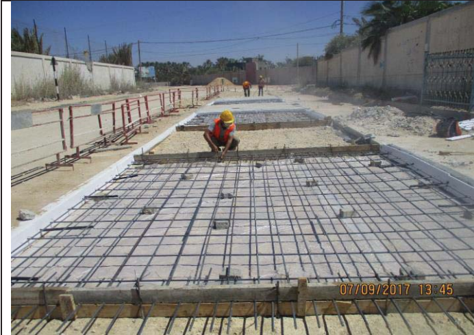
Photo No.11: Surface restoration work at paved concrete road (steel reinforcement) Date: September 7, 2017
