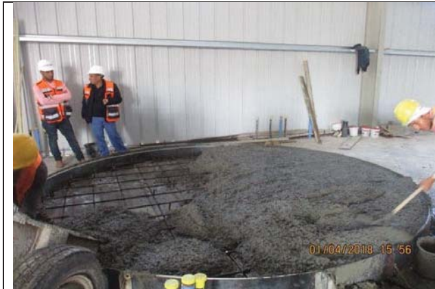
Photo No.01: Casting concrete for 2nd pass RO feed tank base Date: April 01, 2018
