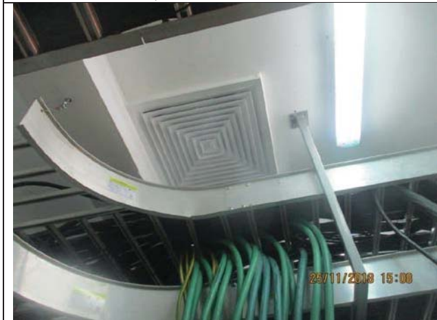
Photo No.15: Diffusers installation for HVAC system in electrical room Date: November 25, 2018
