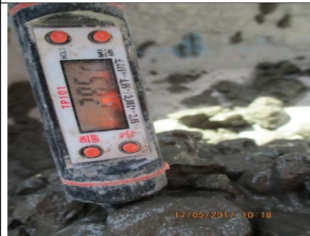
Photo No.07.2: Field quality control tests by CCQC Lab for the casted concrete piles (temperature test). Date: May 17, 2017
