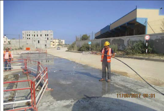
Photo No.19: Surface restoration work at paved concrete road (concrete curing) Date: September 11, 2017
