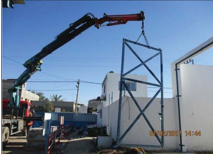
Photo No.11: Demolition of existing ICRC emergency store steel gate Date: February 07, 2017
