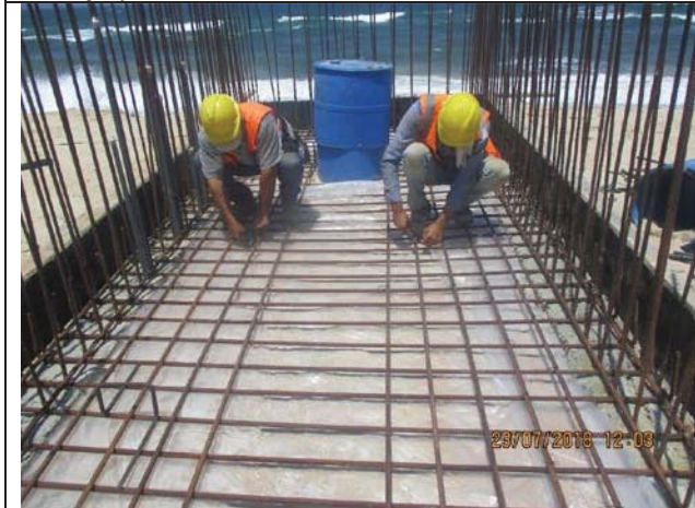
Photo No.27: Formwork and steel reinforcement for the pad of beach well No.1 Date: July 23, 2018
