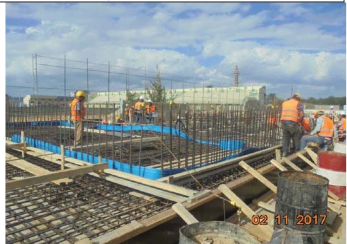
Photo No. 04: Pretreatment foundation (raw water and backwash tanks foundation) reinforcement works.
