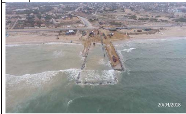
Photo No.29: Supply and installation of 315 mm HDPE pipeline for outfall pipeline from St. 2+045 to St. 2+130. Date: April 20, 2018
