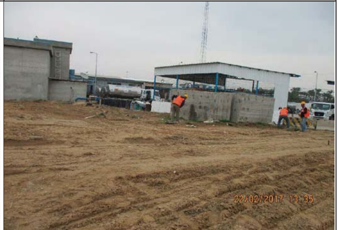
Photo No.20: Pile drilling at the new pre-treatment building area (R06, type L, 16 lm depth). Date: March 22, 2017
