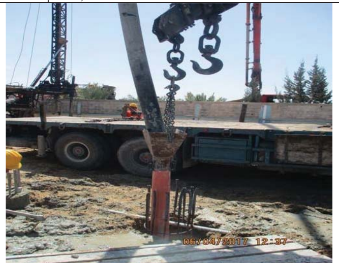
Photo No.10: Supply and cast-in-place concrete using tremie pipes up to end of the pile. Date: April 06, 2017
