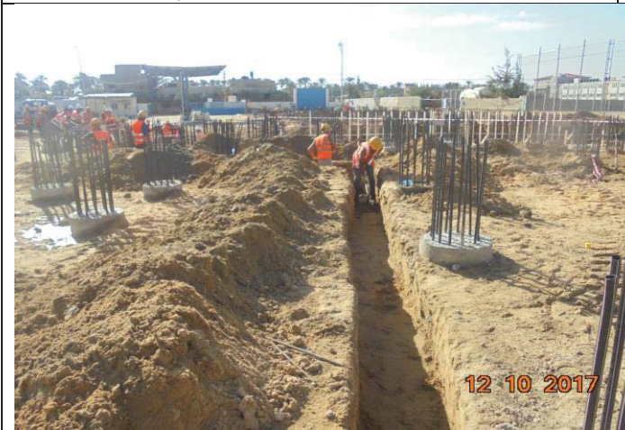
Photo No.21: RO building activities - trench for PVC drainage pipes. Date: October 12, 2017
