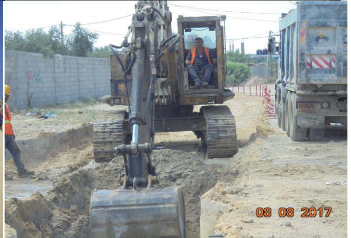
Photo No.20: Pipeline (intake and outfall) construction activities (trench excavation). Date: August 08, 2017
