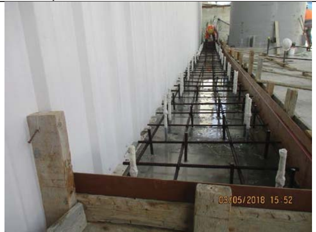
Photo No.04: Shuttering works and steel reinforcement for chemical skid area pad. Date: May 03, 2018
