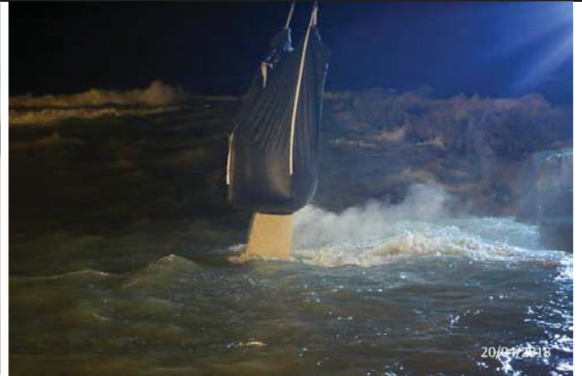
Photo No.32: Pipe surround granular backfilling for outfall pipeline from St. 2+045 to St. 2+130 Date: April 20, 2018
