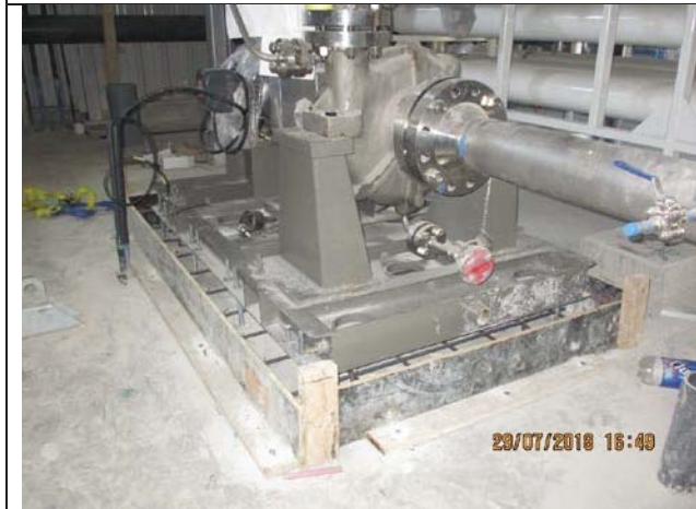
Photo No.35: Formwork and steel reinforcement for booster pumps pads. Date: July 29, 2018
