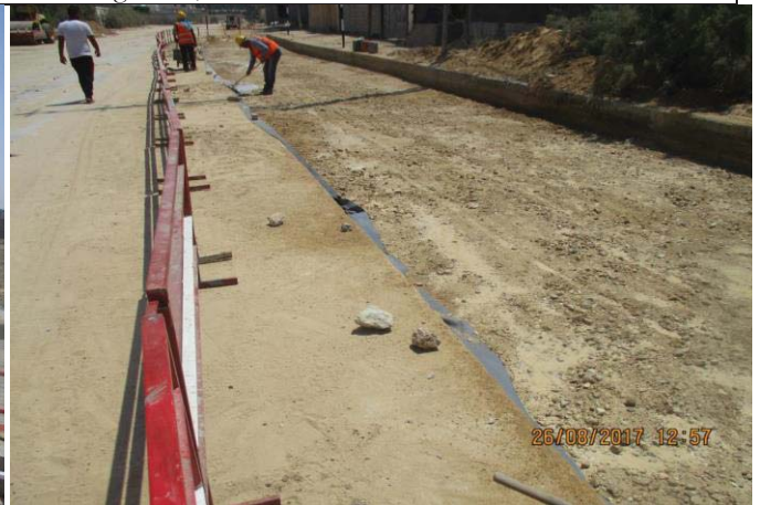
Photo No.64: Surface restoration work at paved concrete road (aggregate base compaction). Date: August 26, 2017
