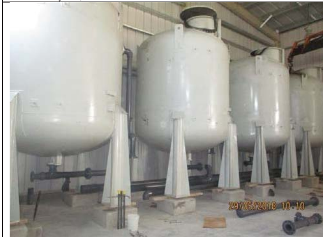
Photo No.27: Installation and continue fabrication of calcite contactors PVC manifold. Date: May 29, 2018
