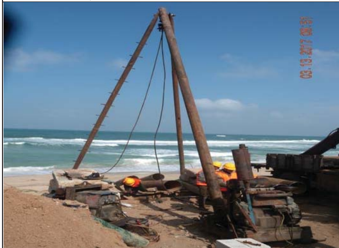
Photo No.09: Hydrogeology investigation by drilling one beach well borehole. Date: March 13, 2017
