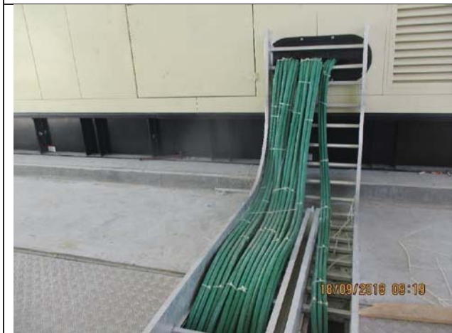
Photo No.23: Cable connections for generator Date: September 18, 2018
