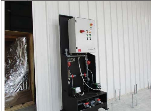
Photo No.03: Chemical dosing skid Date: May 02, 2018
