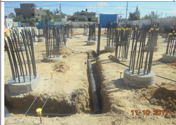
Photo No.15: UPVC pipes 4" for pretreatment. Date: October 11, 2017
