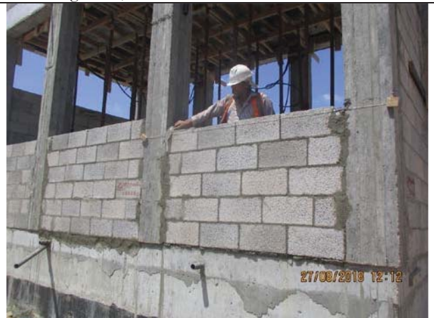
Photo No.22: Blocks building in beach well electrical room Date: August 27, 2018
