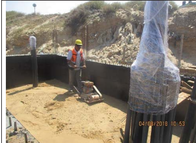
Photo No.05: Backfilling works under concrete pad of beach well electrical room. Date: August 04, 2018
