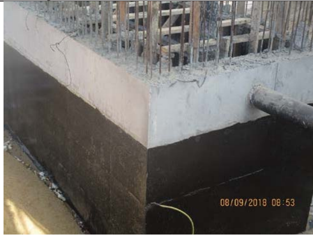
Photo No.09: Epoxy coating for retaining walls of beach wells No.2 Date: September 08, 2018
