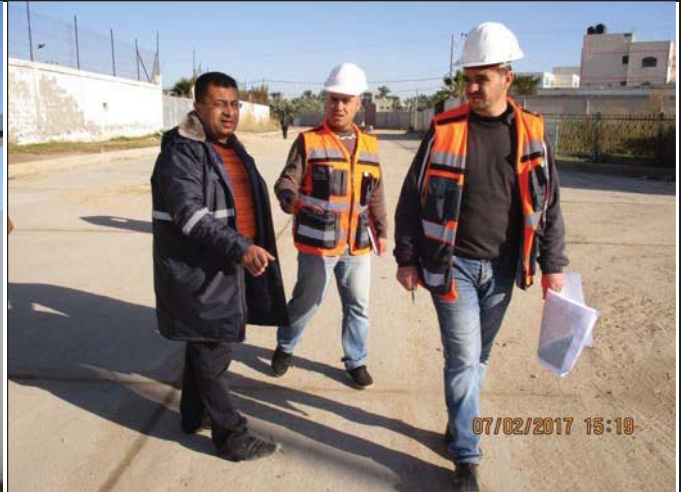
Photo No.12: Walk-through over the proposed pipelines (Intake + Brine) route. Date: February 07, 2017
