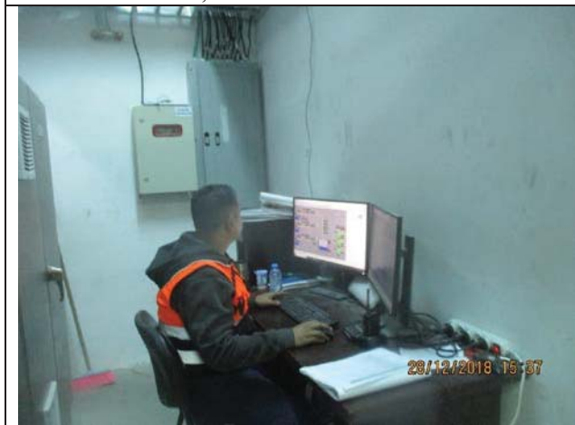
Photo No.27: Configuration and program work inside the electrical room Date: December 28, 2018
