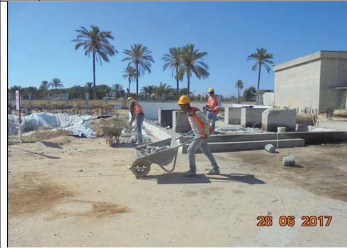
Photo No.15: Demolition of existing fuel tank and relocation of fuel tanks Date: June 28, 2017
