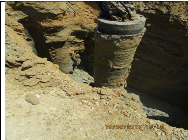
Photo No.11.2: Pile construction activity (quality investigation test at RO building). Date: August 19, 2017
