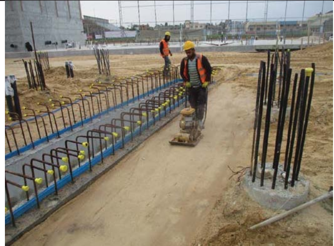
Photo No.10: backfilling and leveling works around the generator pad trench Date: February 06, 2018
