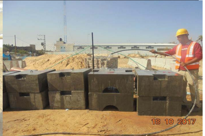
Photo No.38: Weight collars for outfall pipeline - curing the previously casted collars. Date: October 18, 2017
