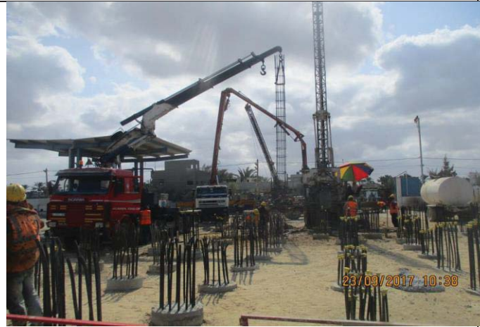
Photo No.33: Pile construction activity (raw water and backwash tanks) Date: September 23, 2017
