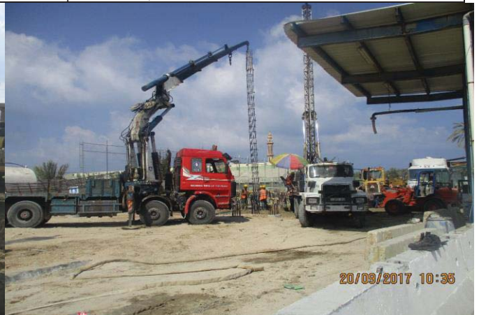
Photo No.30: Pile construction activity (raw water and backwash tanks) Date: September 20, 2017
