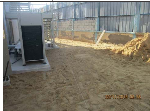
Photo No.11: Backfilling, leveling and compaction works beside RO Building Date: November 20, 2018
