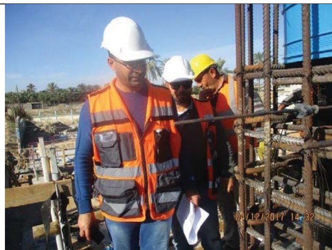
Photo No.06: Raw water and backwash tanks steel reinforcement works. Date: December 04, 2017
