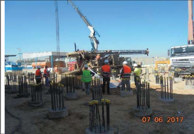
Photo No.07: AECOM CM visit to the project site to witness piles construction Date: June 07, 2017
