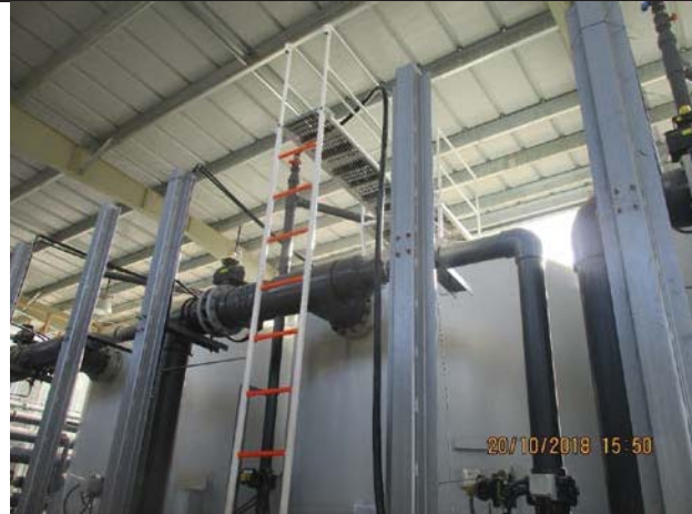
Photo No.11: Continue filling for DMF tanks for hydrostatic testing Date: October 20, 2018
