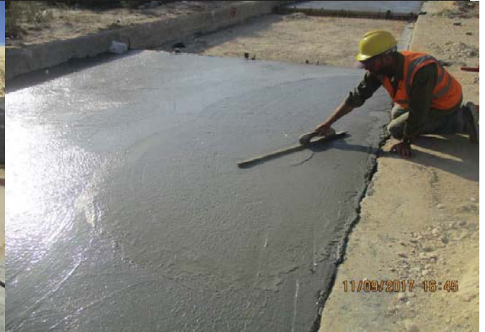
Photo No.20: Surface restoration work at paved concrete road (concrete work) Date: September 11, 2017
