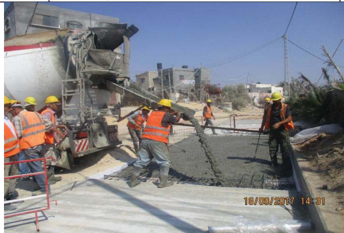
Photo No.27: Surface restoration work at paved concrete road (concrete casting) Date: September 18, 2017
