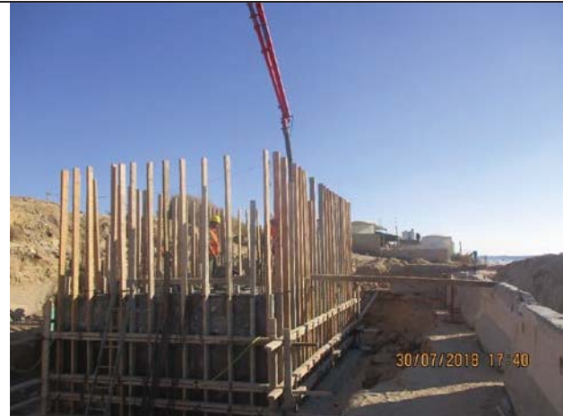
Photo No.39: Casting concrete for retaining walls of beach well electrical room Date: July 30, 2018
