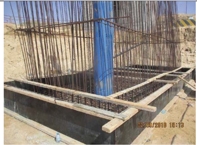
Photo No.02: Formwork and steel reinforcement for beach well No. 2 retaining walls foundation Date: September 02, 2018
