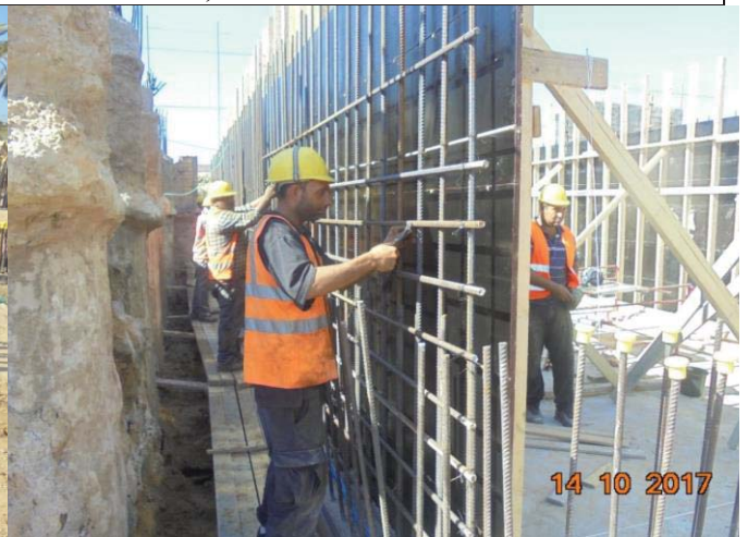
Photo No.24: Continue brine tank construction activities – steel reinforcement fabrication for tank walls. Date: October 14, 2017
