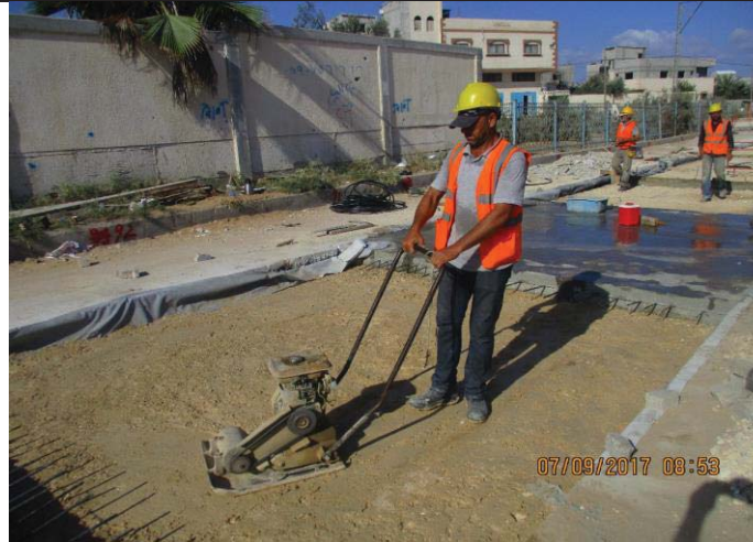
Photo No.13: Surface restoration work at paved concrete road (compaction works) Date: September 7, 2017
