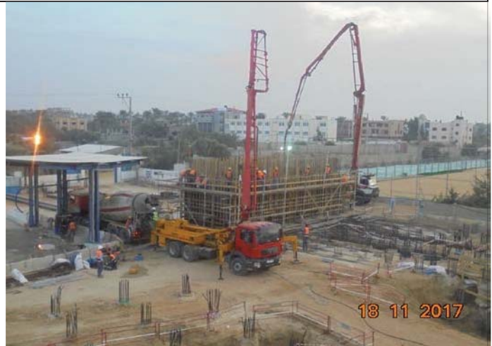
Photo No. 22: Casting concrete for raw water and backwash tanks walls. Date: November 18, 2017
