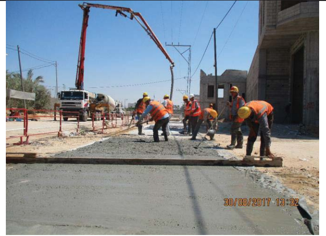
Photo No.74: Surface restoration work at paved concrete road (surface leveling.) Date: August 30, 2017
