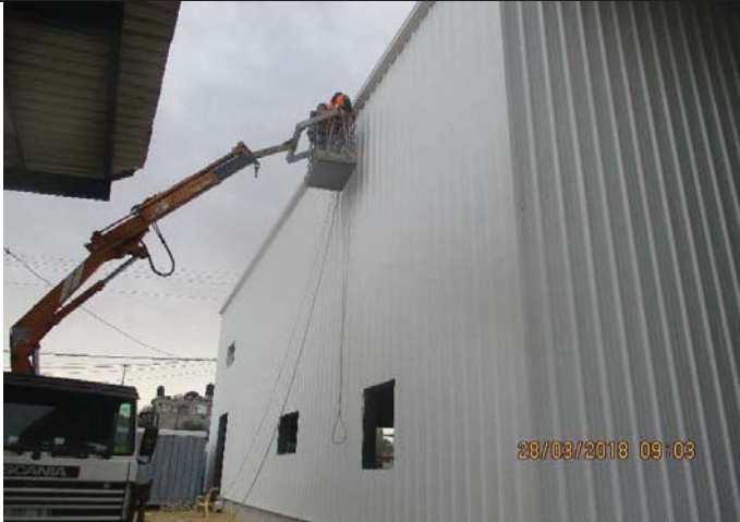
Photo No.29: Continue installation of walls panels for workshop area Date: March 28, 2018
