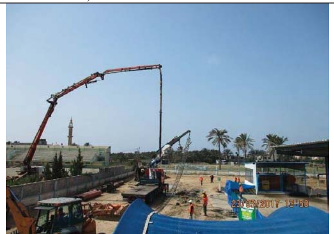
Photo No.26: Installation of reinforcement steel casing and supply & placement of reinforced concrete.
