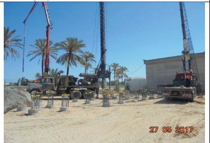
Photo No.12: Drilling and concrete reinforcement activities for the new RO building piles construction. Date: May 27, 2017
