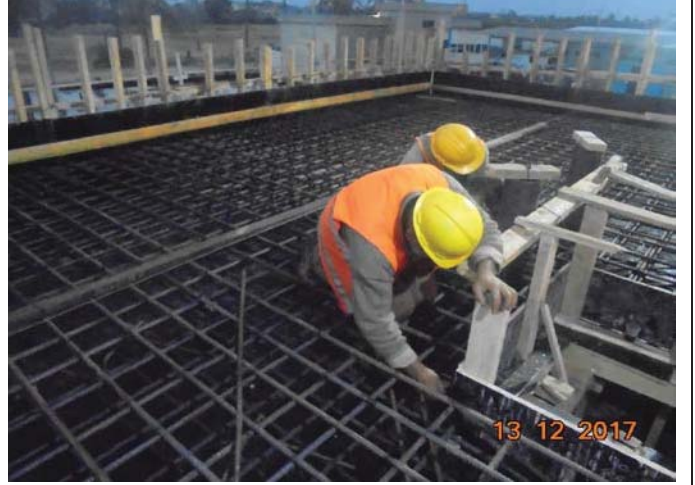
Photo No.28: Raw water and backwash tanks forming, steel reinforcing works for slab casting. Date: December 13, 2017
