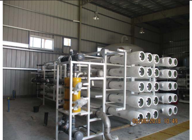
Photo No.10: Installing of energy recovery device (ERD) Unit-2 in place. Date: June 05, 2018
