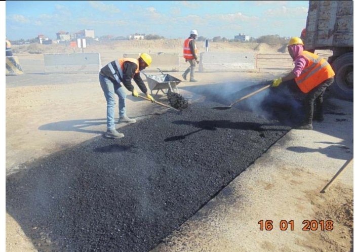
Photo No.20: Reinstatement works for the intake pipelines, which are crossing Al Rasheed street. Date: January 16, 2018
