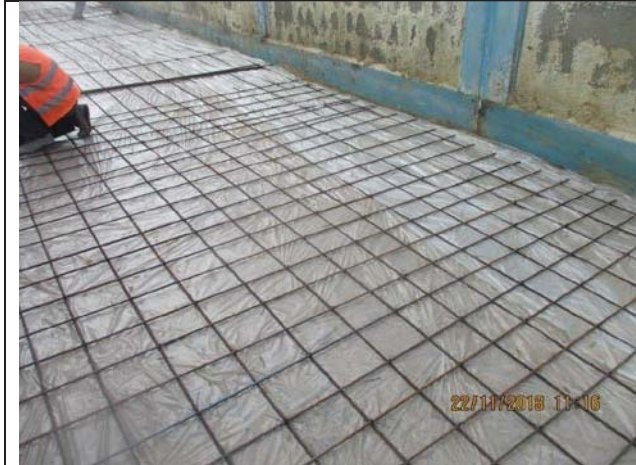
Photo No.13: Shuttering and reinforcement work under concrete sidewalk beside RO Building Date: November 22, 2018
