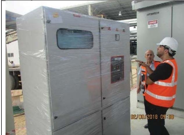
Photo No.03: Metering panel in generator area Date: September 02, 2018
