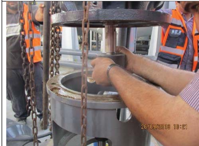
Photo No.29: Coupling connection for brine discharge pumps. Date: September 26, 2018
