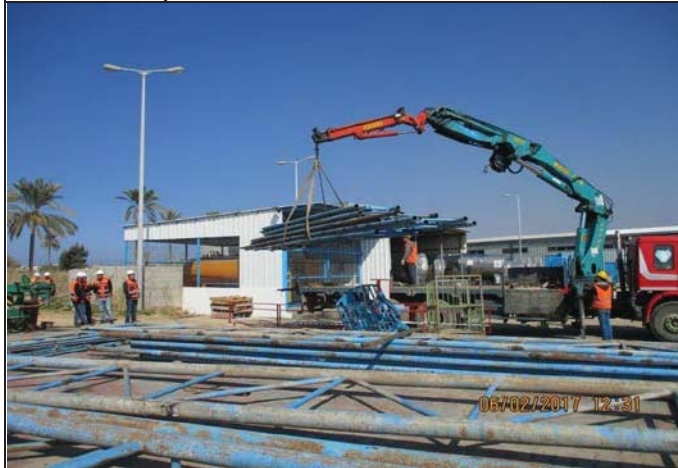
Photo No.09: Continue transferring materials from the steel canopy structure to CMWU stores.
