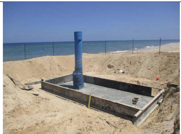
Photo No.18: Formwork for retaining wall foundation beach well No. 1 Date: June 20, 2018
