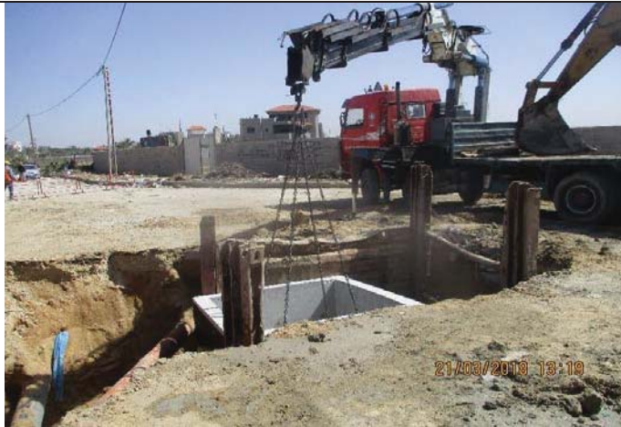
Photo No.21: Excavation works, chamber installation and backfilling works for washout chamber No.2. Date: March 21, 2018
