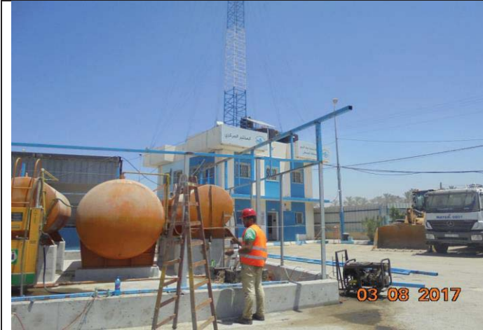
Photo No.13: Continue works at fuel tank area – fabricating the shed. Date: August 03, 2017
