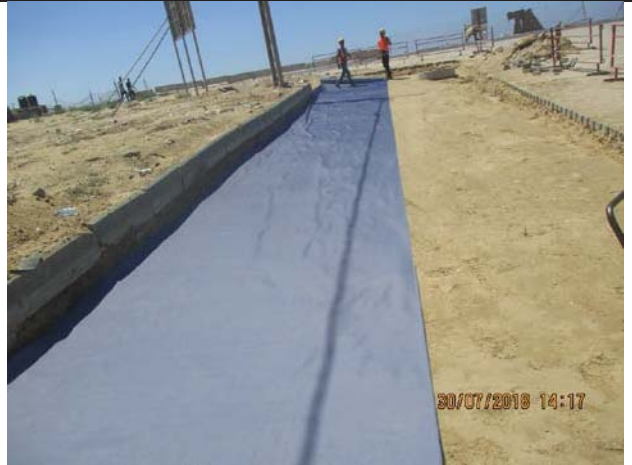
Photo No.38: Backfilling, geotextile laying and base course furnishing on chamber. Date: July 30, 2018
