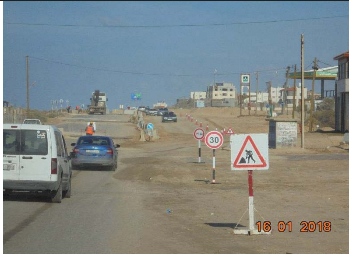
Photo No.19: Safety arrangement for traffic on Al Rasheed street to facilitate crossing road by residents. Date: January 16, 2018
