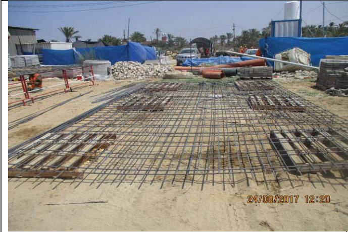
Photo No.61: Surface restoration work at concrete paved road (steel rebar preparation). Date: August 24, 2017
