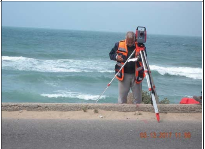
Photo No.10: Survey works to verify obstacles prior to start work at the proposed new beach wells layout. Date: March 13, 2017
