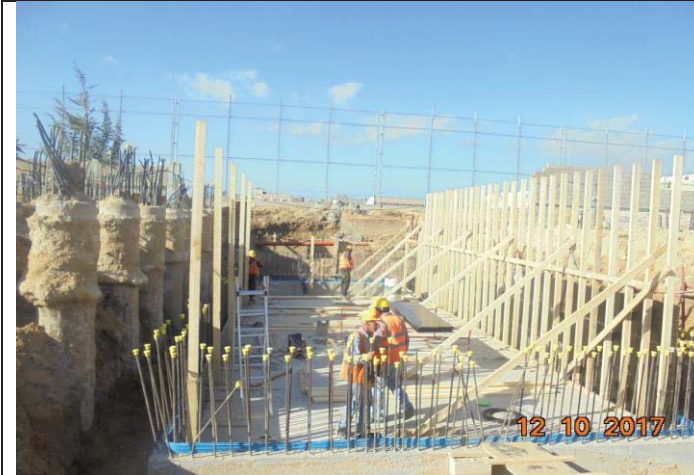
Photo No.19: Continue brine tank construction activities- formwork for tank walls. Date: October 12, 2017
