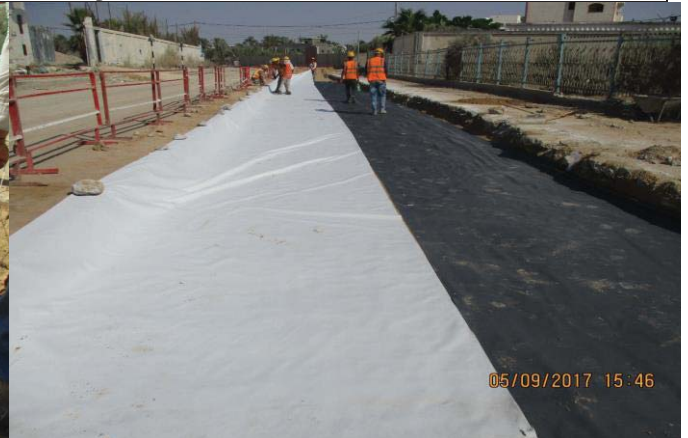
Photo No.06: Surface restoration work at paved concrete road (filter fabric installation) Date: September 5, 2017
