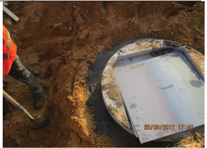
Photo No.46: Electrical conduit manhole laying for MV and fiber optic cable (manhole covering). Date: August 20, 2017.
