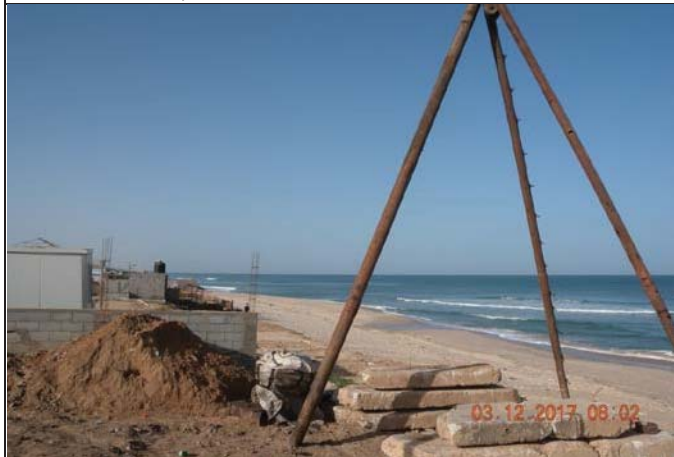
Photo No.07: Preparation works for hydrogeology investigation by drilling one beach well borehole. Date: March 12, 2017
