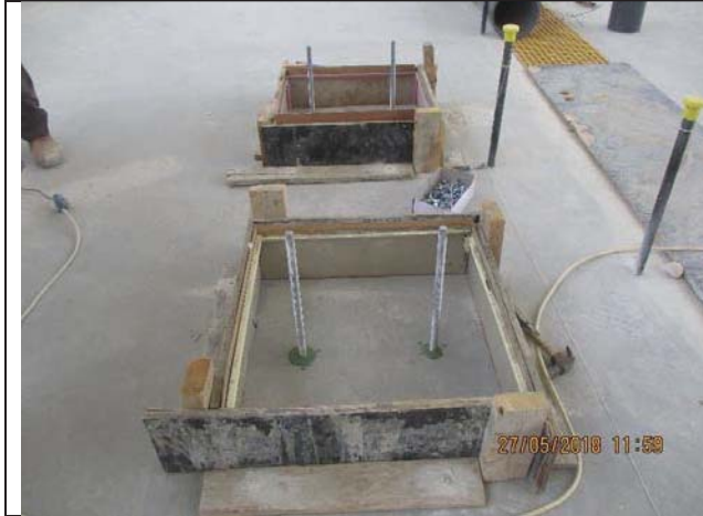
Photo No.25: Formwork and steel reinforcement for dual media filter pads (3 units) Date: May 27, 2018
