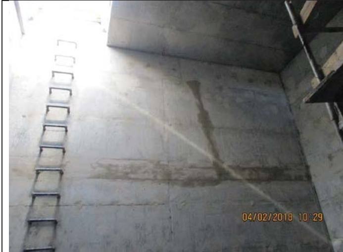
Photo No.05: Repairing works for the internal walls of raw water tank. Date: February 04, 2018
