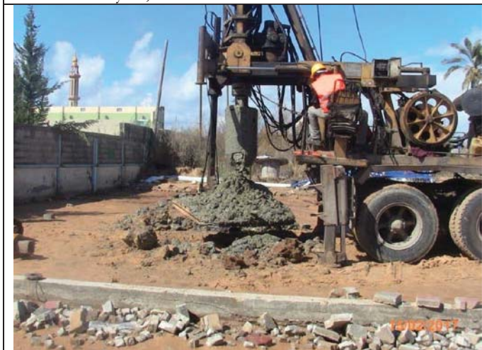
Photo No.15: Pile test investigation at the new proposed pretreatment and RO location Date: February 15, 2017
