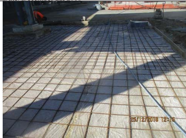
Photo No.23: Shuttering and steel reinforcement under tiling works under existing station Date: December 25, 2018
