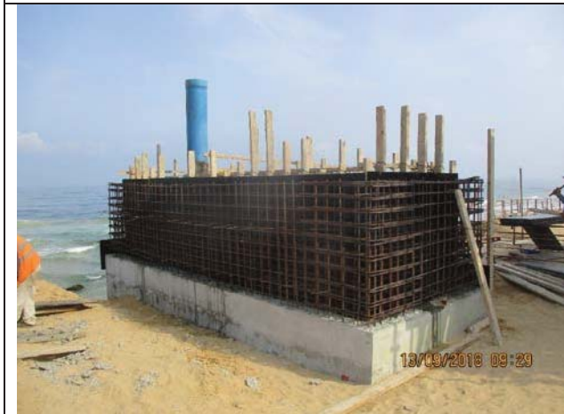
Photo No.15: Formwork and steel reinforcement for part 2 walls of beach well No. 2 Date: September 13, 2018
