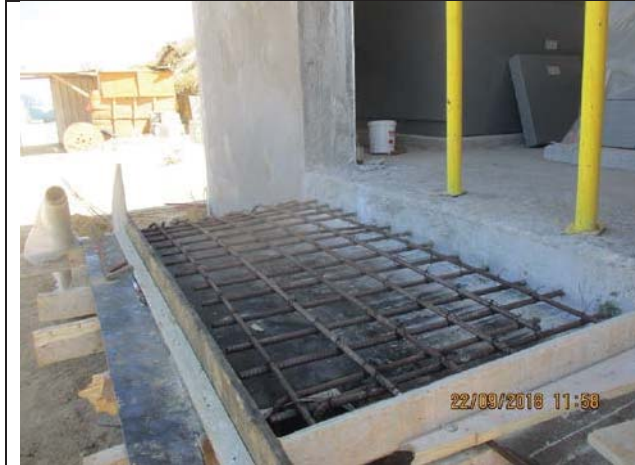
Photo No.25: Formwork, steel reinforcement and casting concrete for stairs of electrical room. Date: September 22, 2018
