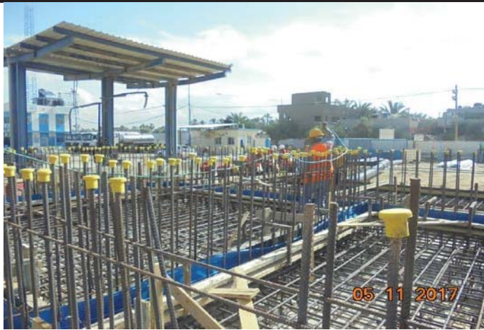
Photo No. 07: Raw water and backwash tanks steel reinforcing, electrical embedment and formwork completion.
