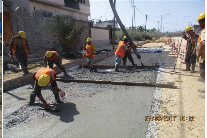
Photo No.62: Surface restoration work at concrete paved road (surface restoration). Date: August 27, 2017
