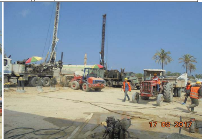
Photo No.40: Pile construction activity (pile drilling at brine tank and pre-treatment building) Date: August 17, 2017
