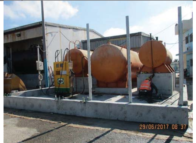
Photo No.16: Relocate the existing tanks to the new area. Date: June 29, 2017
