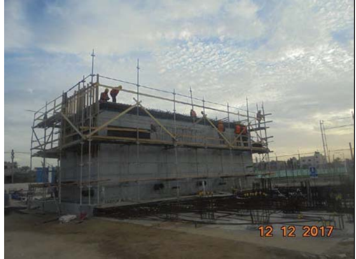
Photo No.26: Internal Formwork and steel reinforcement at raw water and backwash tanks slab. Date: December 12, 2017
