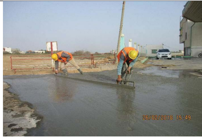
Photo No.38: Casting concrete for reinstatement works of intake pipeline from St. 1+015.00 to St. 1+030.00. Date: February 26, 2018.
