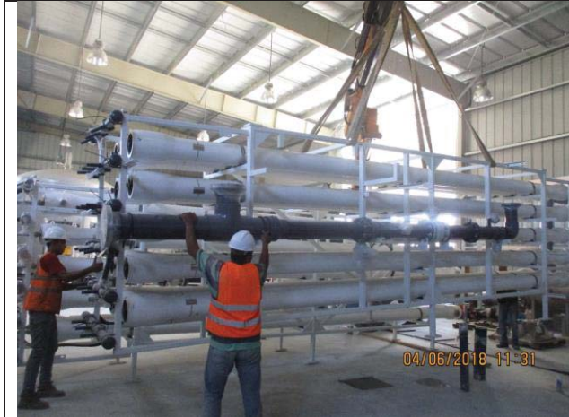
Photo No.07: Installing of 1 st Pass RO skid unit-1 in place. Date: June 04, 2018
