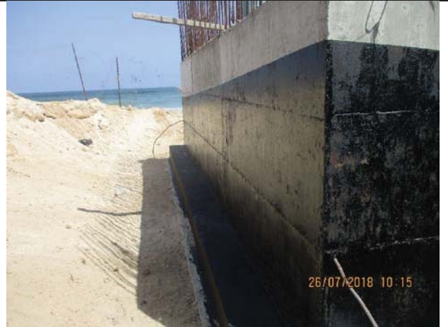
Photo No.32: Repair and insulation works for beach well No. 3 retaining walls. Date: July 26, 2018
