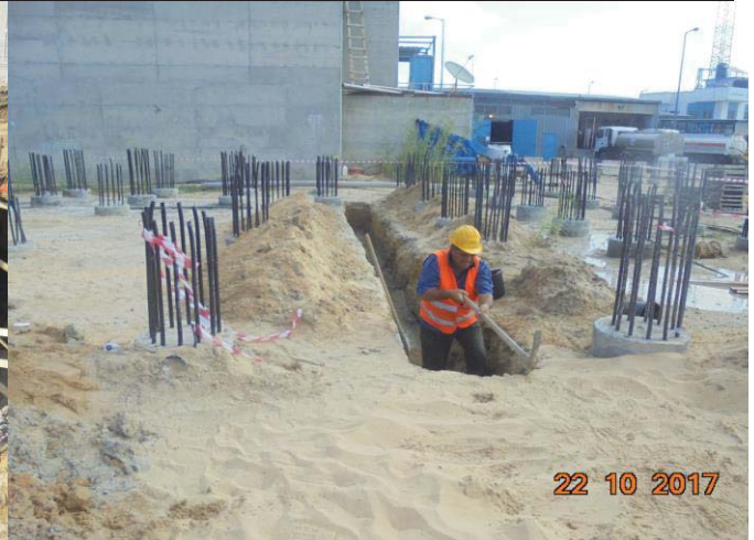
Photo No.44: Trench excavation for PVC underground pipes prior to RO building. Date: October 22, 2017
