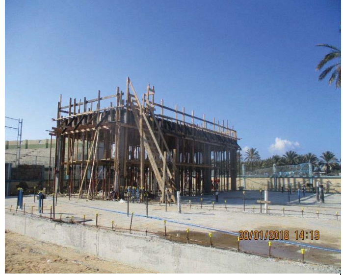
Photo No.42: shuttering works and steel reinforcement for roof slab of electrical room. Date: January 30, 2018
