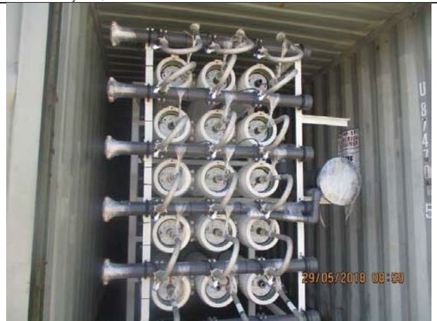
Photo No.28: Preparing works to start installation of 2 nd pass RO skid Date: May 29, 2018
