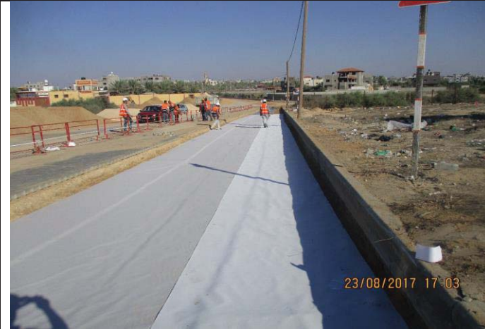
Photo No.55: Surface restoration work at interlock tile area (filter fabric installation). Date: August 23, 2017
