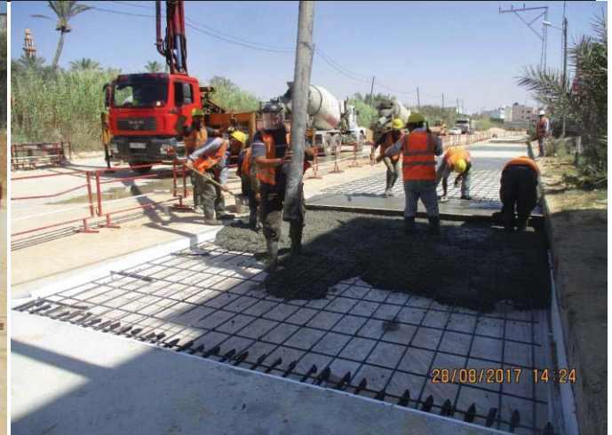
Photo No.68: Surface restoration work at paved concrete road (concrete pouring). Date: August 28, 2017
