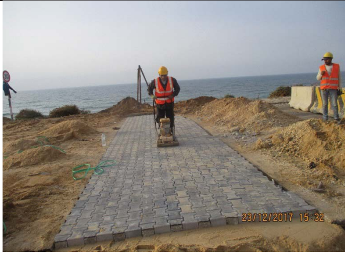
Photo No.47: Installation of temporary tiles above the excavated areas on the existing asphalt road Date: December 23, 2017
