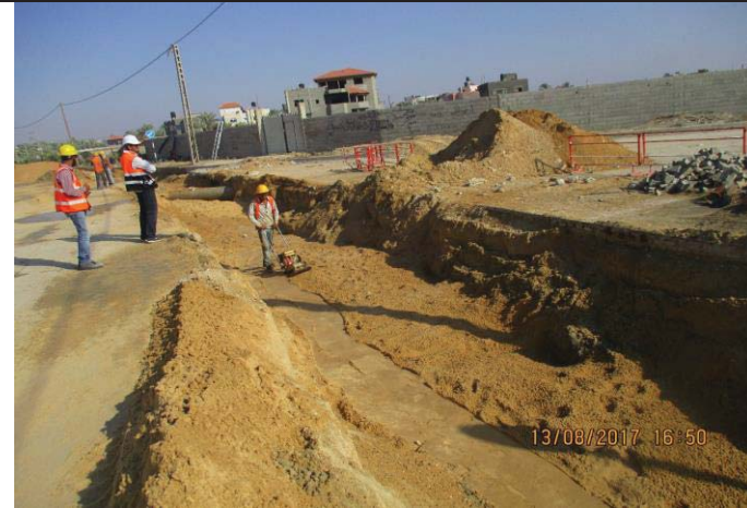
Photo No.33: Pipeline construction activity (excavated material transfer to dumping site). Date: August 13, 2017
