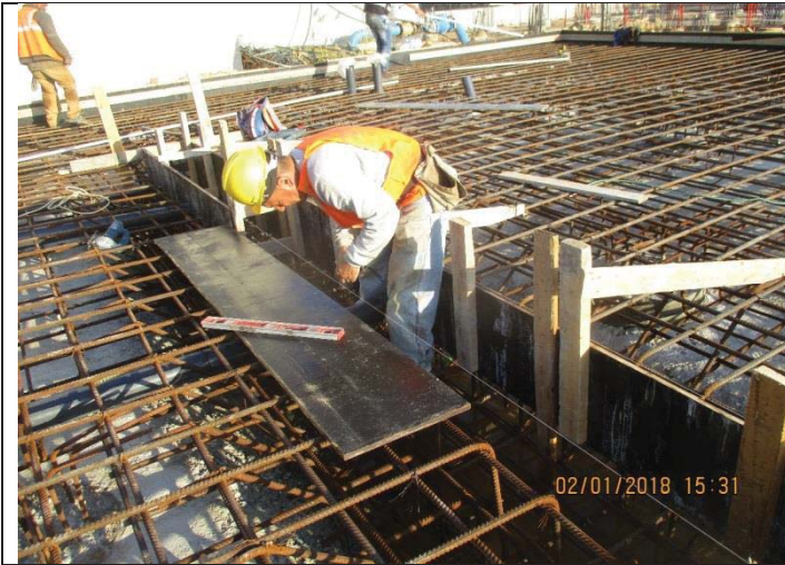
Photo No.01: Continue formwork and steel reinforcement for RO building foundation (phase 01). Date: January 02, 2018
