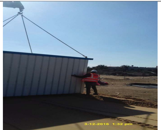
Photo No.04: Containers installation for contractor site office, guardroom & portable WC Date: December 03, 2016
