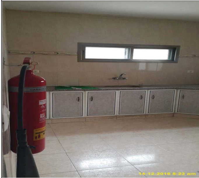
Photo No.11: Fire extinguishers provided in primary field office
