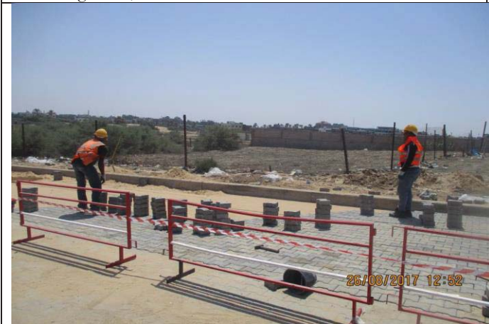
Photo No.63: Surface restoration work at interlock tile area (interlock restoration). Date: August 26, 2017
