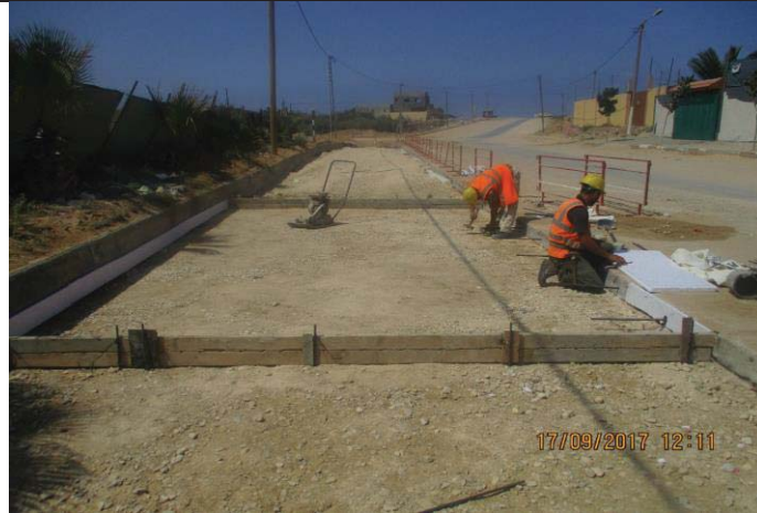
Photo No.25: Surface restoration work at paved concrete road (compaction) Date: September 17, 2017
