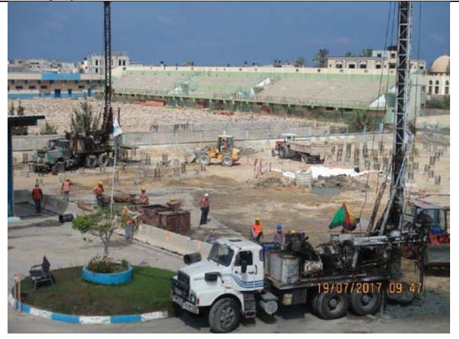
Photo No.24: Piles construction activities in pretreatment and generator pad area. Date: July 19, 2017
