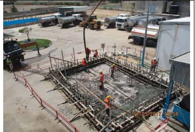
Photo No.04: Fuel tank relocation-Supply and cast-in-place reinforced concrete slab-on-grade and walls. Date: May 14, 2017
