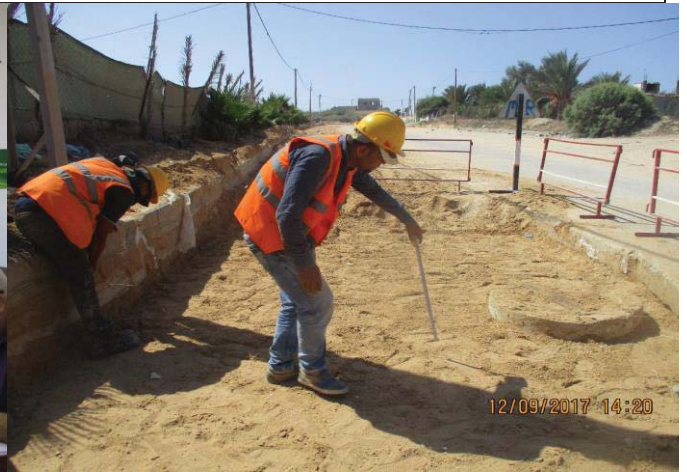
Photo No.22: Surface restoration work at paved concrete road (subgrade works ) Date: September 12, 2017
