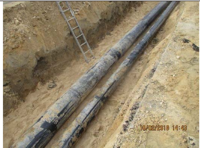
Photo No.16: Supply and install all HDPE piping, fittings, and associated appurtenances for outfall and intake pipelines
