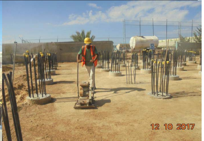
Photo No.20: Pre-treatment construction activities - continue land leveling, watering and compaction. Date: October 12, 2017
