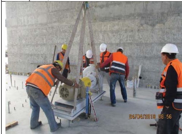
Photo No.35: Installing pumps in its places in RO building and pretreatment area Date: April 24, 2018
