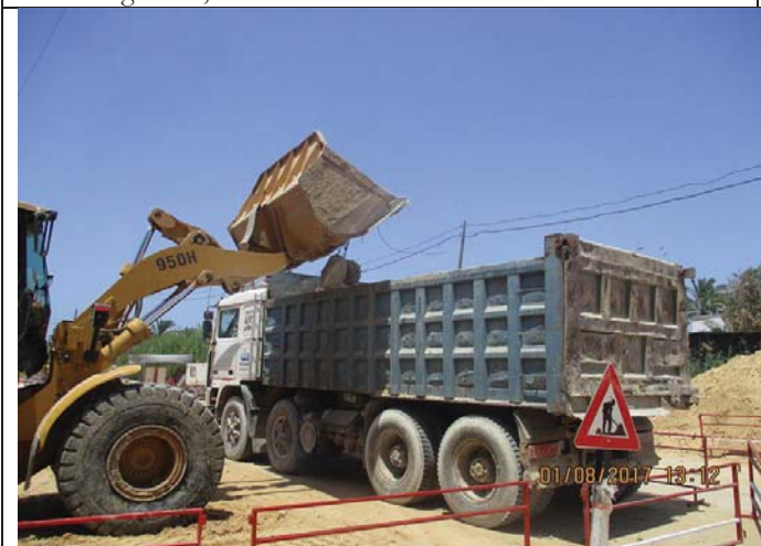
Photo No.05: Pipeline preparation activities (debris transfer to dumping site). Date: August 01, 2017
