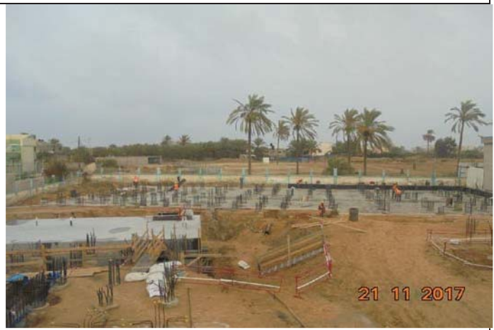
Photo No. 28: R.O building works suspended due to heavy rain. Date: November 21, 2017
