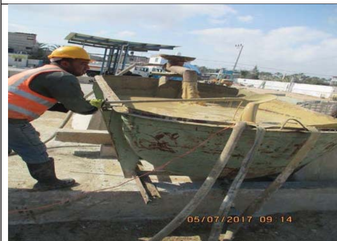
Photo No.09: Bentonite preparing by mixing with water in the tank. Date: July 05, 2017
