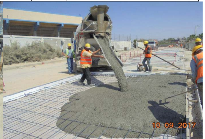
Photo No.18: Surface restoration work at paved concrete road (concrete casting) Date: September 10, 2017
