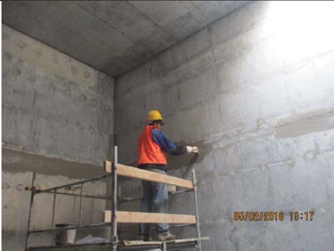
Photo No.09: repairing works for the internal walls of raw water tank. Date: February 05, 2018
