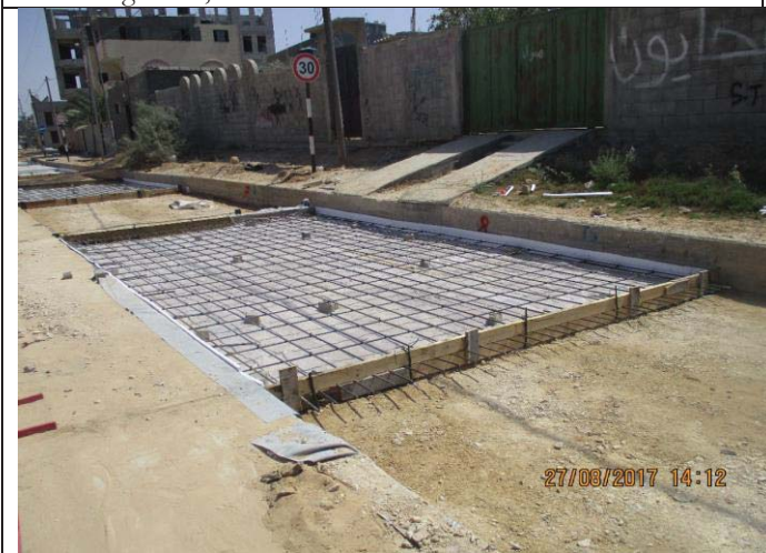
Photo No.65: Surface restoration work at concrete paved road (steel reinforcing). Date: August 27, 2017
