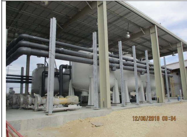
Photo No.15: Fixation of backwash manifold to DMF tanks in place with steel support in pretreatment building. Date: June 12, 2018
