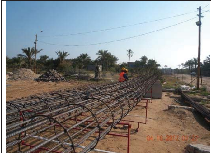
Photo No.15: Reinforcement steel preparation for piles at storage yard. Date: April 16, 2017
