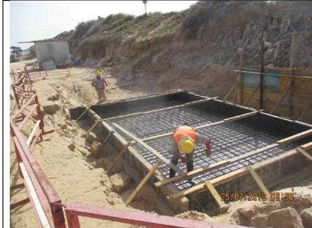
Photo No.31: Formwork and steel reinforcement for the electrical room pad Date: July 25, 2018
