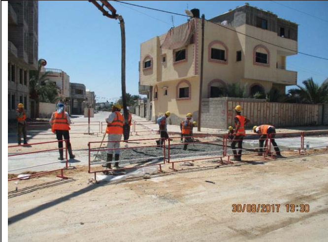
Photo No.73: Surface restoration work at paved concrete road (concrete casting) Date: August 30, 2017
