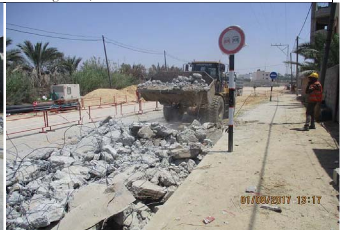
Photo No.04: Pipeline preparation activities (transfer debris to dumping site). Date: August 01, 2017
