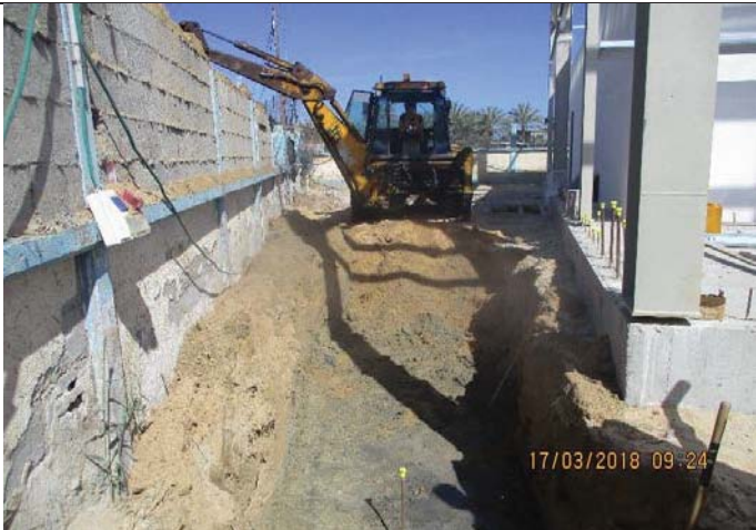
Photo No.15: Excavation works for duct banks inside construction site. Date: March 17, 2018
