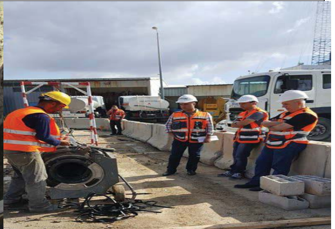
Photo No.12: Welding and fabricating embedded underground pipes in the RO building – 315mm HDPE pipeline. Date: October 10, 2017
