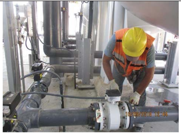
Photo No.12: Instrumentation connections Date: September 10, 2018
