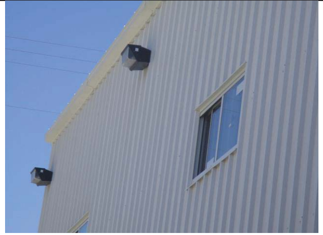
Photo No.20: External lighting installation for workshop area Date: June 20, 2018
