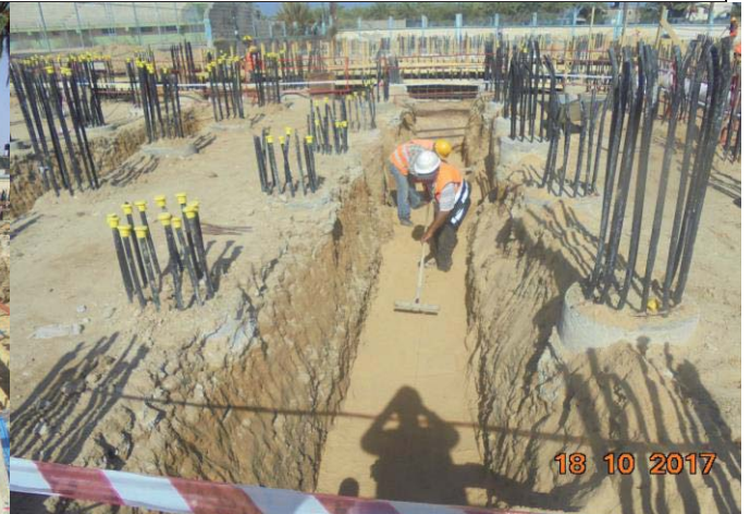
Photo No.36: Pre-treatment building activities – excavation for the two main trenches. Date: October 18, 2017
