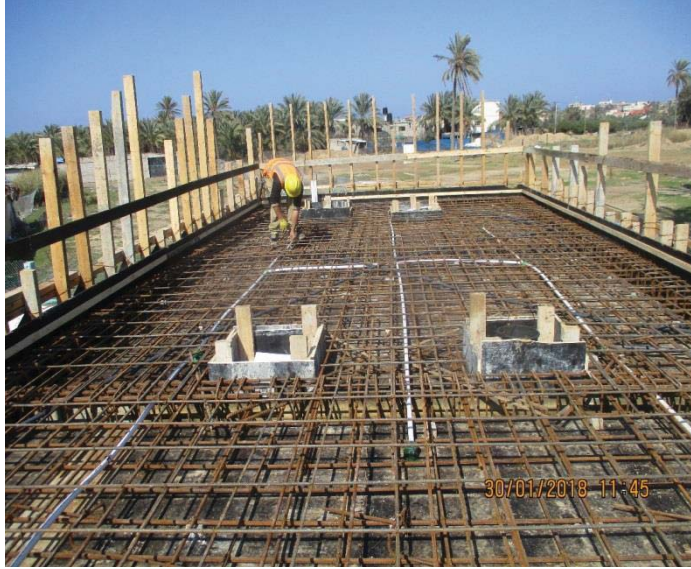
Photo No.41: Electrical and mechanical installation for roof slab of electrical room. Date: January 30, 2018
