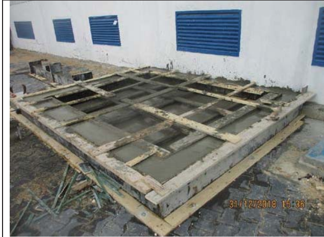
Photo No.33: Formwork, steel reinforcement and casting concrete for existing generator. Date: December 31, 2018
