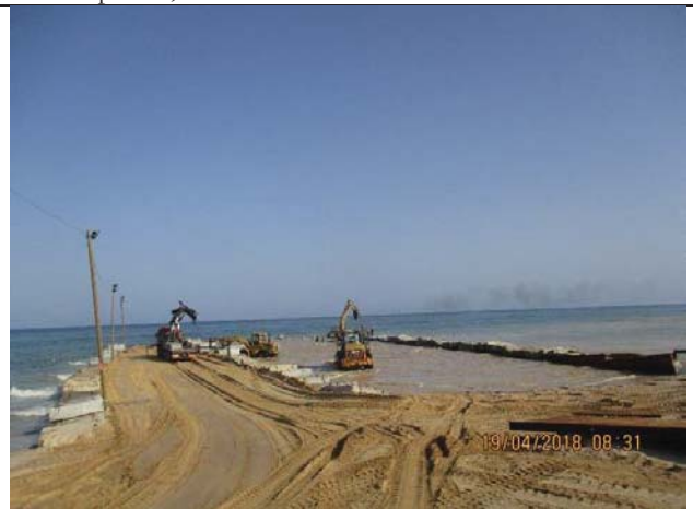
Photo No.24: Resume preparation works for outfall pipeline installation after stoppage Date: April 19, 2018
