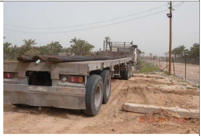
Photo No.08: Delivery of reinforcement steel bars at storage yard. Date: March 12, 2017
