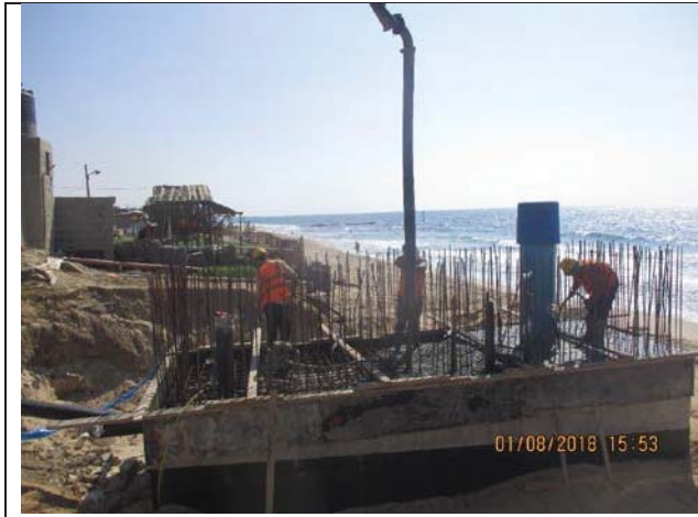
Photo No.01: Casting concrete for concrete pad of beach well No. 1 Date: August 01, 2018
