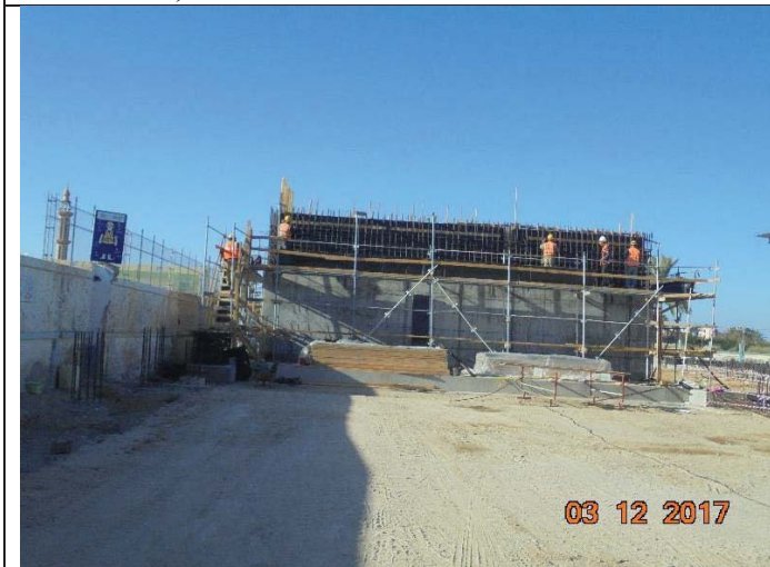
Photo No.03: Steel reinforcement for the second layer of backwash and row water tanks Date: December 03, 2017
