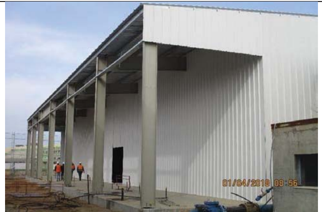
Photo No.02: Continue works in walls and roof panels of RO building Date: April 01, 2018
