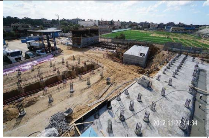
Photo No. 30: Site securing, concrete barriers installation and warning signs installation. Date: November 22, 2017
