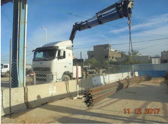
Photo No.25: Raw water and backwash tanks reinforcement steel unloading. Date: December 11, 2017
