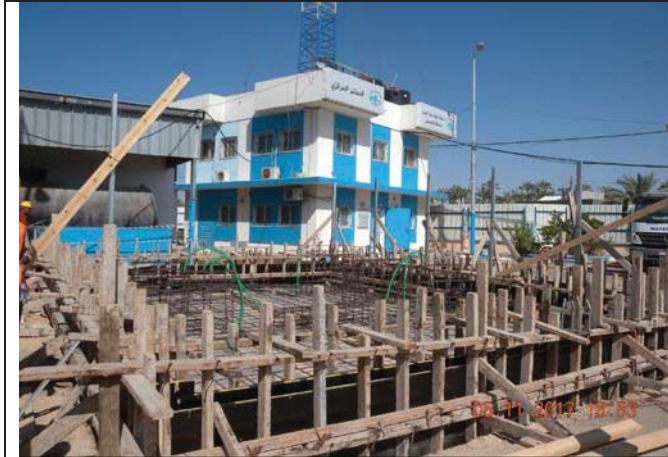
Photo No.03: Fuel tank relocation activity - Installation of posts for fencing and gate before concrete casting. Date: May 11, 2017
