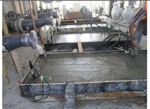
Photo No.34: Casting concrete for the pad of feed and backwash pumps. Date: July 26, 2018
