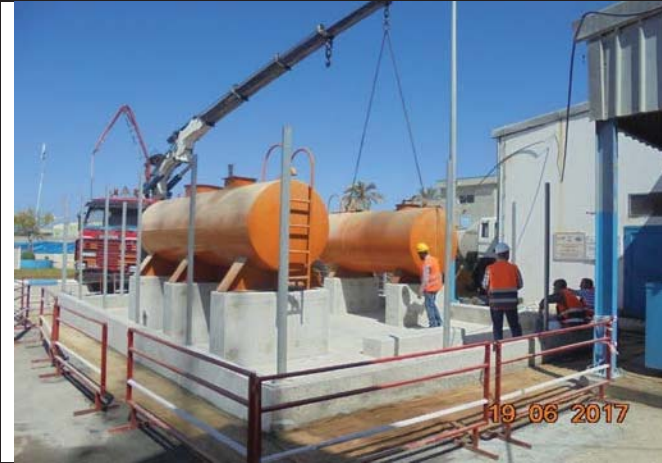
Photo No.13: Continue demolition of existing fuel tank and diesel tanks relocation prior to fuel tank relocation activity. Date: June 19, 2017
