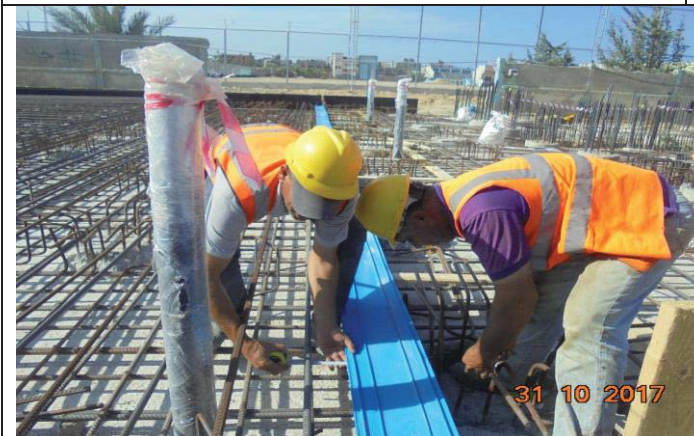
Photo No.59: Raw water and back wash tanks (steel reinforcing). Date: October 31, 2017
