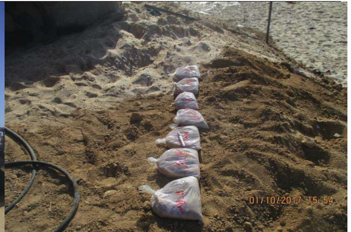
Photo No.02: Beach well construction activity (beach well No. 02- sample collection) Date: October 1, 2017
