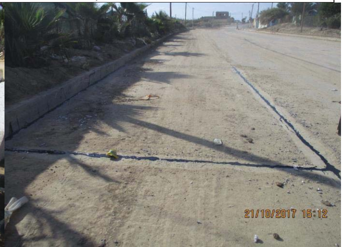
Photo No.42: Continue joints filling in between concrete panels in the road over the pipeline route. Date: October 21, 2017
