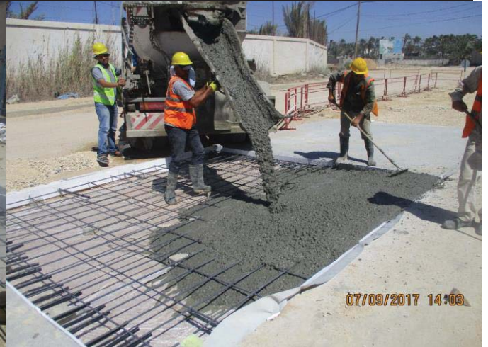
Photo No.12: Surface restoration work at paved concrete road (concrete casting) Date: September 7, 2017
