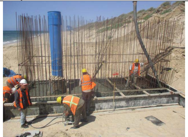
Photo No.22: Casting concrete for the foundation of beach well No. 1 Date: June 21, 2018
