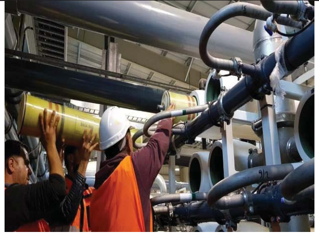
Photo No.14: Membrane installing for the first train of 1 st Pass RO Skid. Date: January 21, 2019
