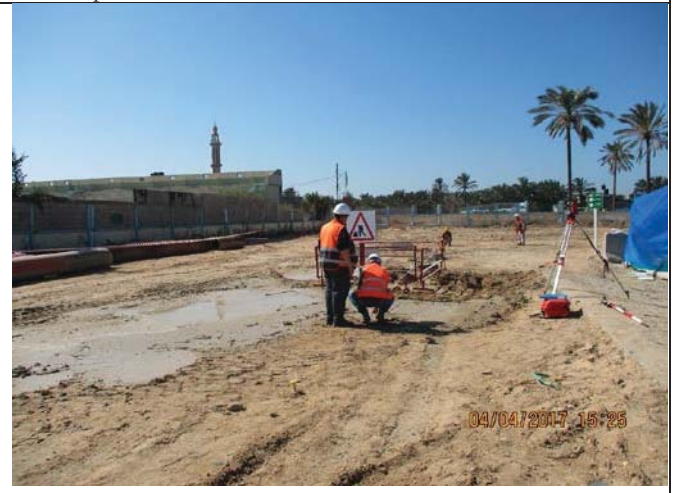
Photo No.04: Surveying works for piles allocation as per approved shop drawing. Date: April 04, 2017
