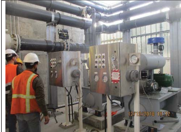
Photo No.13: Blower running Date: December 12, 2018
