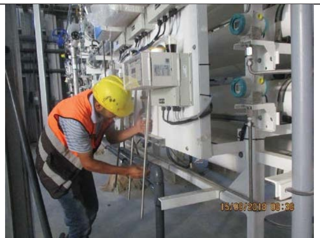
Photo No.18: Instrumentation connection Date: September 15, 2018
