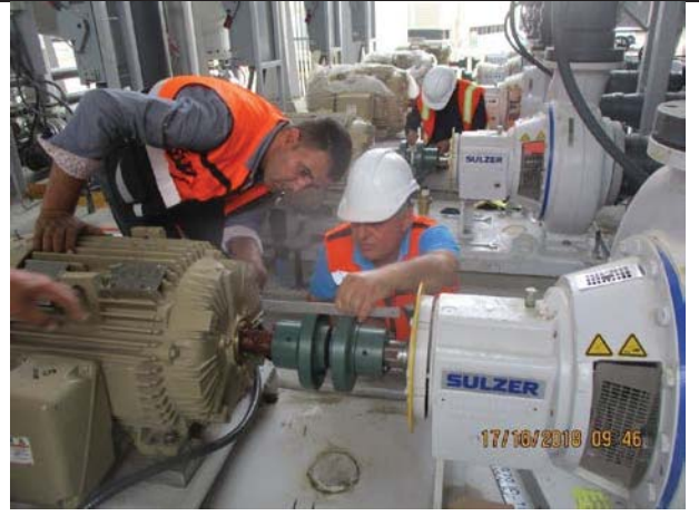
Photo No.10: Shaft coupling for pumps Date: October 17, 2018
