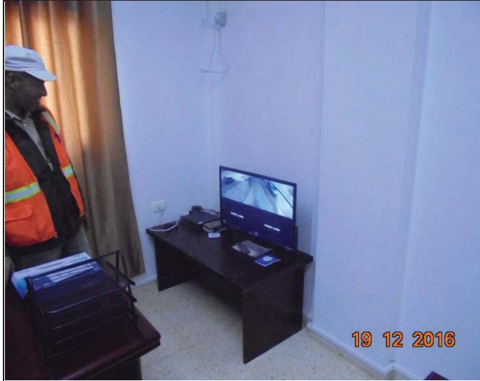
Photo No.13: primary field office CCTV system inspection Date: December 19, 2016
