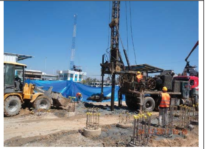
Photo No.16: Pile construction activity at the new pre-treatment building area. Date: April 17, 2017
