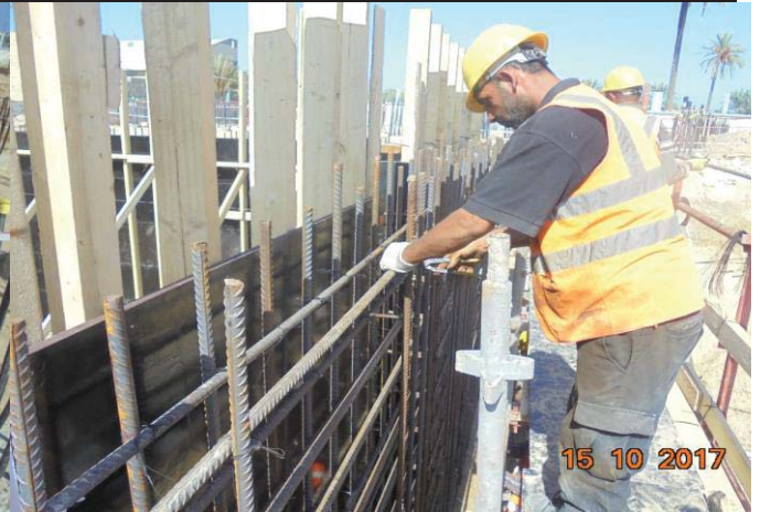
Photo No.28: Continue brine tank construction activities – steel reinforcement fabrication for tank walls. Date: October 15, 2017
