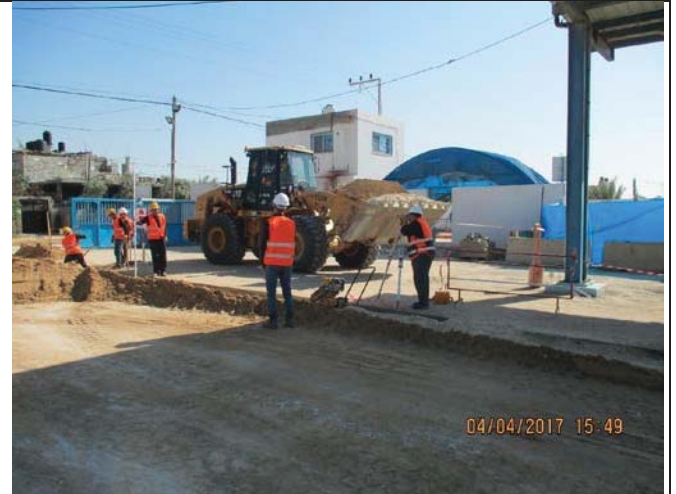
Photo No.02: Reinstatement works for storm-water pipeline - laying and watering base course layer. Date: April 04, 2017
