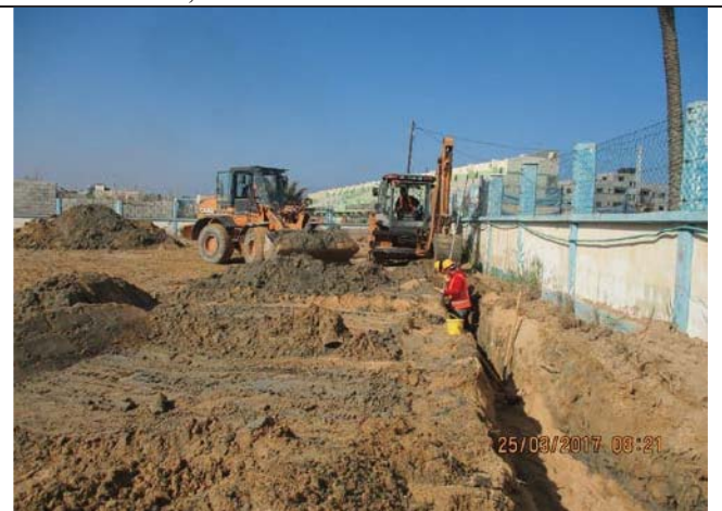
Photo No.28: Continue brine line relocation activities including excavation, bedding, pipe installation and backfilling.
