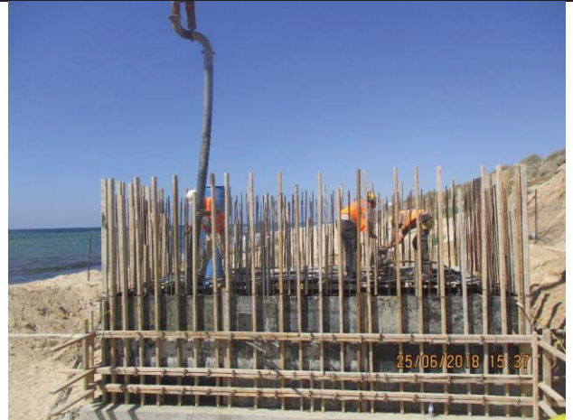
Photo No.26: Casting concrete for retaining wall of Beach well No. 1 Date: June 25, 2018
