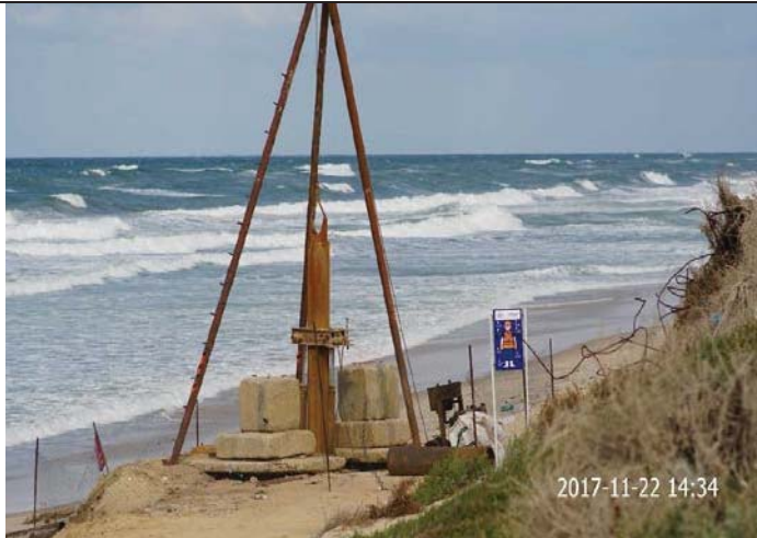
Photo No. 33: Beach well no 01 & 02 securing, concrete barriers installation and warning signs installation – cable tool driller. Date: November 22, 2017
