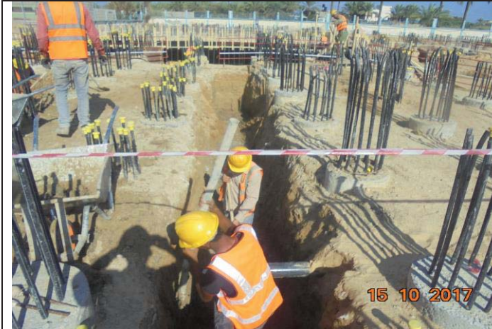
Photo No.27: Pre-treatment building activities – excavation for the two main trenches. Date: October 15, 2017
