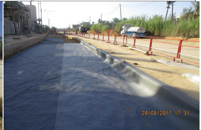
Photo No.60: Surface restoration work at interlock tile area (filter fabric installation). Date: August 24, 2017
