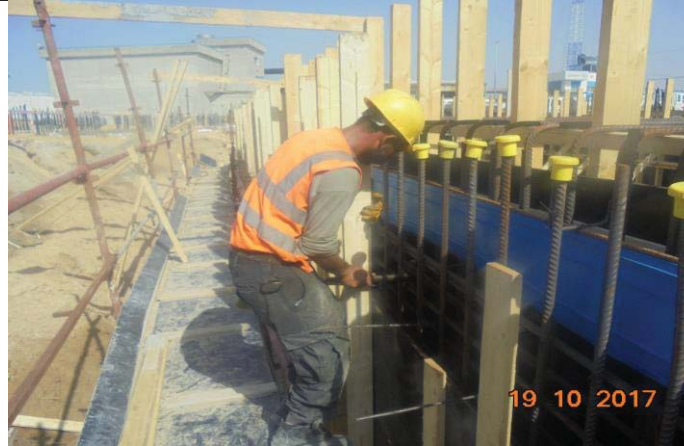
Photo No.39: Formwork and steel reinforcement works for brine tank walls. Date: October 19, 2017
