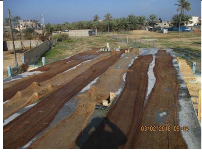
Photo No.02: Curing for the casted concrete of electrical room roof slab by spreading water and furnishing wet burlaps.
