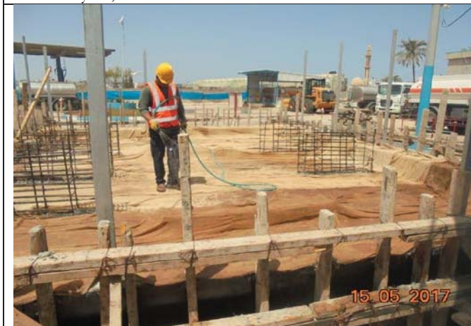
Photo No.05: Fuel tank relocation-Curing of casted-in-place concrete slab and walls. Date: May 15, 2017
