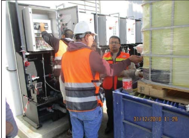
Photo No.31: Onsite training for PWA staff "Liquid chemical feed system" Date: December 31, 2018
