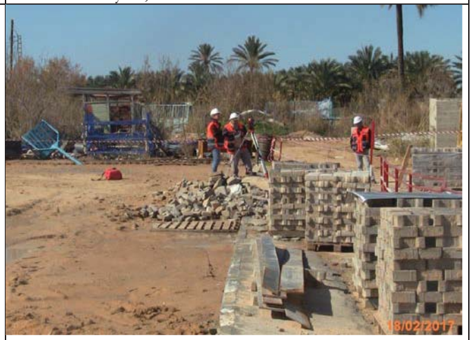
Photo No.16: Surveying works to identify coordinates for new pretreatment building and brine tank. Date: February 18, 2017
