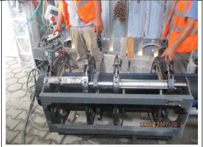
Photo No.14: HDPE pipe welding trial test at storage yard. Date: July 12, 2017
