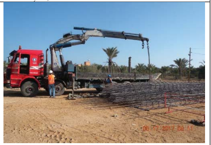
Photo No.06: Continue fabricating reinforcement steel case for piles at storage yard. Date: May 17, 2017
