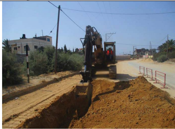
Photo No.45: Electrical conduit laying for MV and fiber optic cable. Date: August 20, 2017
