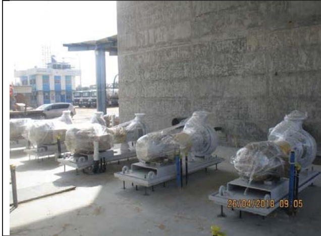
Photo No.37: Installing pumps in its places in RO building and pretreatment area. Date: April 26, 2018
