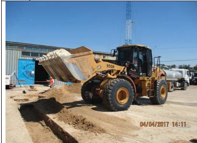
Photo No.03: Reinstatement works for brine line - laying and watering base course layer. Date: April 04, 2017
