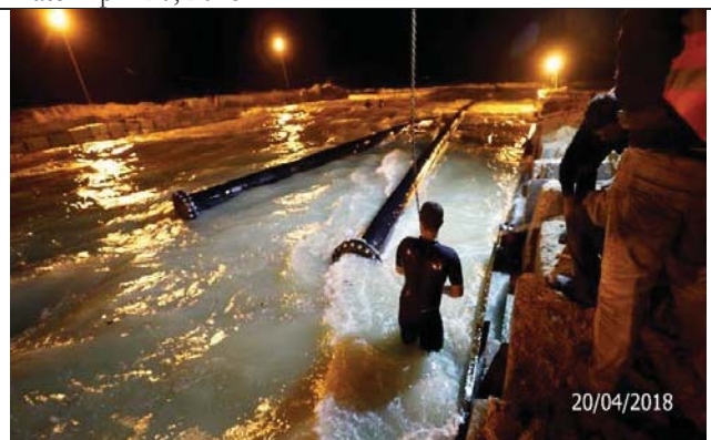
Photo No.30: Supply and installation of 315 mm HDPE pipeline for outfall pipeline from St. 2+045 to St. 2+130. Date: April 20, 2018
