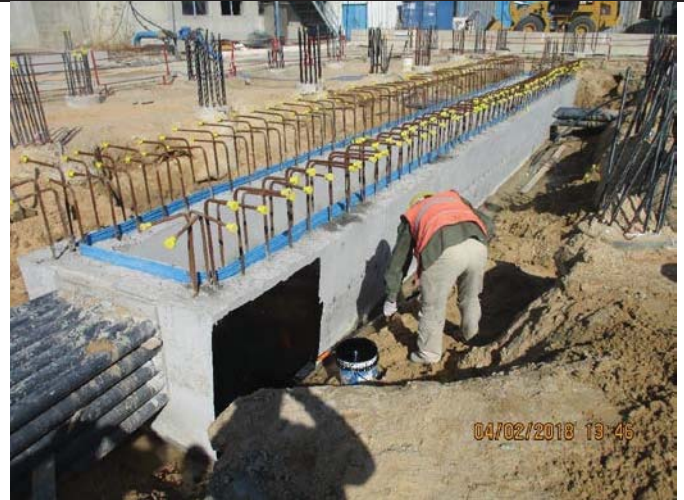
Photo No.06: Coating for external face of the generator pad trench Date: February 04, 2018
