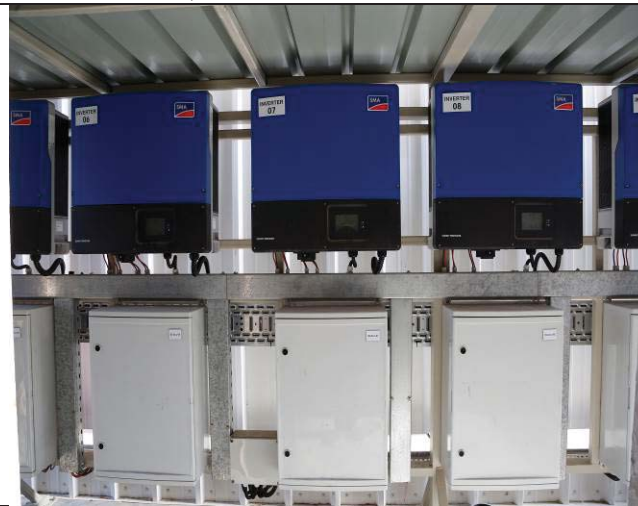
Photo No.15: Solar system Date: October 21, 2018
