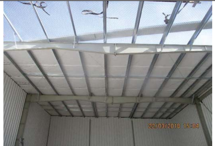
Photo No.22: Start works in roof panels of workshop area Date: March 22, 2018
