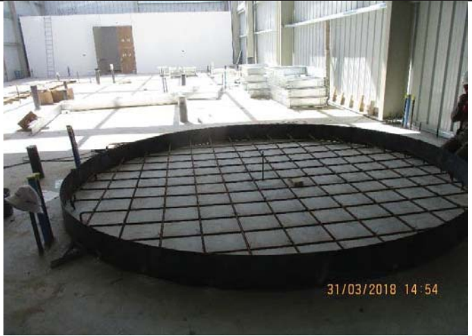
Photo No.32: shuttering works and steel reinforcement for equipment base Date: March 31, 2018
