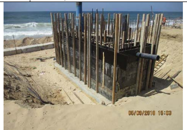
Photo No.06: Second face formwork for beach well No. 2 retaining walls Date: September 05, 2018
