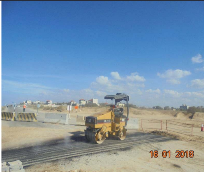
Photo No.21: Reinstatement works for the intake pipelines, which are crossing Al Rasheed street. Date: January 16, 2018
