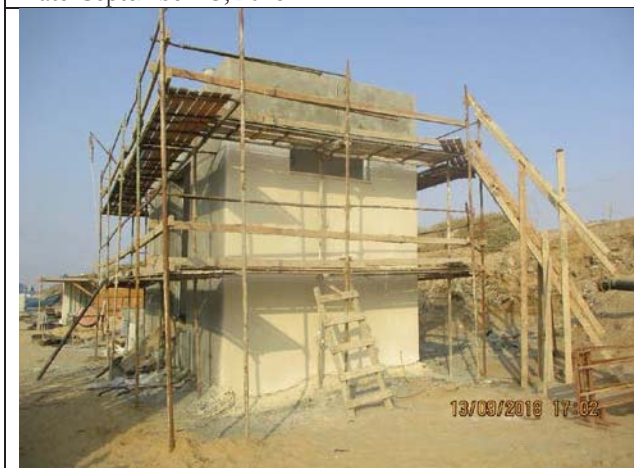
Photo No.17: Plastering works for external walls of beach wells electrical room Date: September 13, 2018
