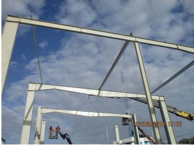
Photo No.39: Start erection works for generator pad steel structure. Date: February 27, 2018.
