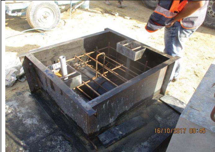
Photo No.31: Continue steel fabrication for outfall pipeline weight collars. Date: October 16, 2017
