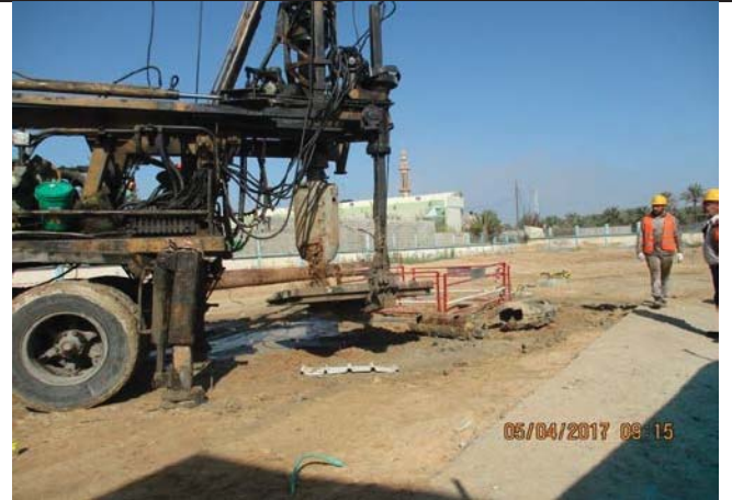
Photo No.06: Pile construction activity at the new pre-treatment building area. Date: April 05, 2017
