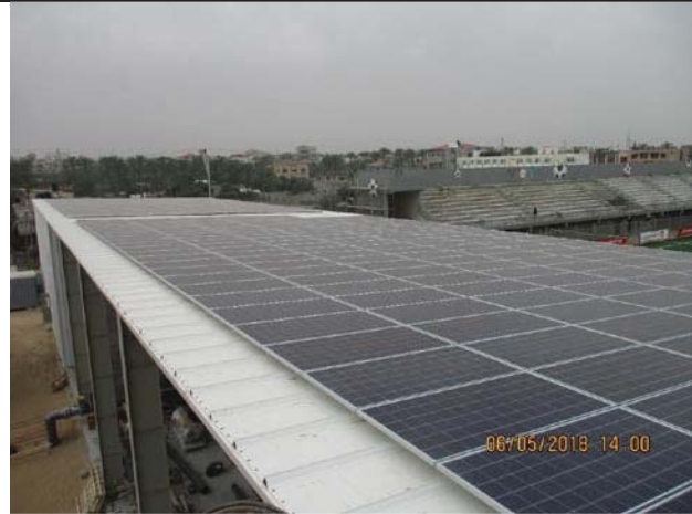
Photo No.09: Finishing installing PV system on the pretreatment canopy Date: May 06, 2018
