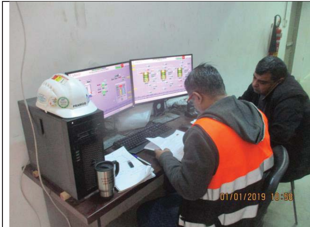
Photo No.01: Configuration works for SCADA system and functional testing. Date: January 01, 2019
