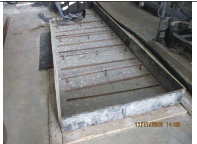
Photo No.06: Shuttering works and steel reinforcement for high pressure pumps pads Date: November 11, 2018
