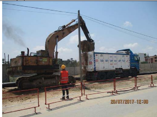
Photo No.27: transferring pipeline trench excavated material to dumping site. Date: July 20, 2017
