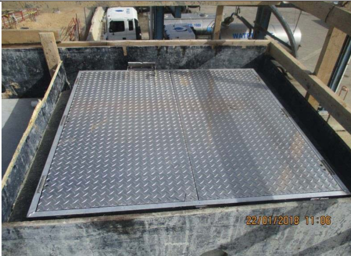
Photo No.29: Formworks for Bilco hatches on brine tank and backwash/raw water tanks.
