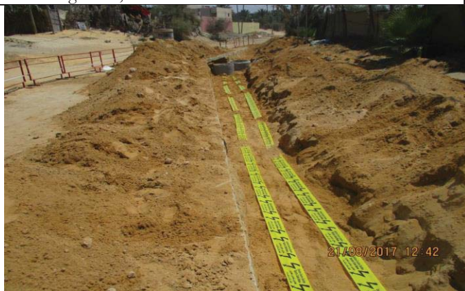
Photo 53: Electrical conduit laying for MV and fiber optic cable (warning tape installation). Date: August 21, 2017
