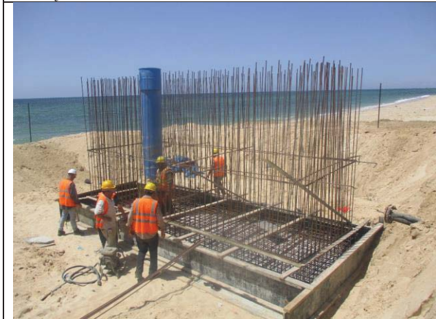
Photo No.21: Formwork & steel reinforcement for retaining wall foundation beach well No. 1 Date: June 21, 2018
