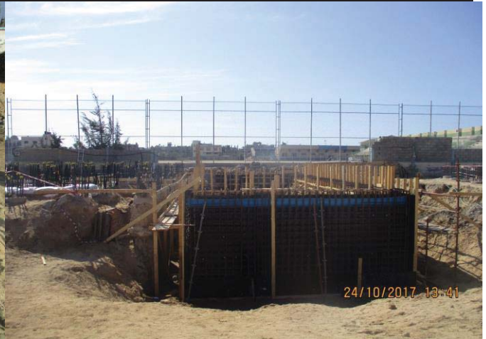
Photo No.46: Formwork activities for raw water and backwash tanks. Date: October 24, 2017
