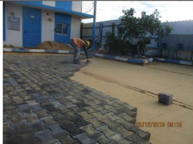
Photo No.21: Reinstatement of interlock tiling for the eastern side of site yard. Date: December 22, 2018
