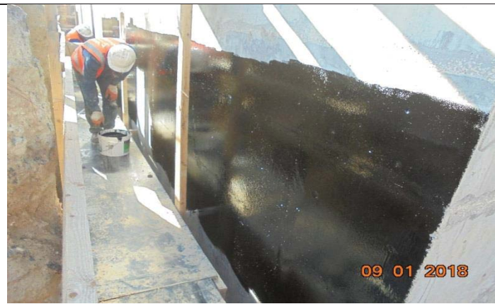
Photo No.09: First layer coating for the external walls of brine tank. Date: January 09, 2018
