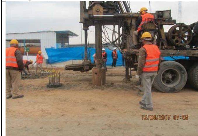
Photo No.13: Drilling, steel reinforcement and concrete casting for pile No. T10. Date: April 12, 2017
