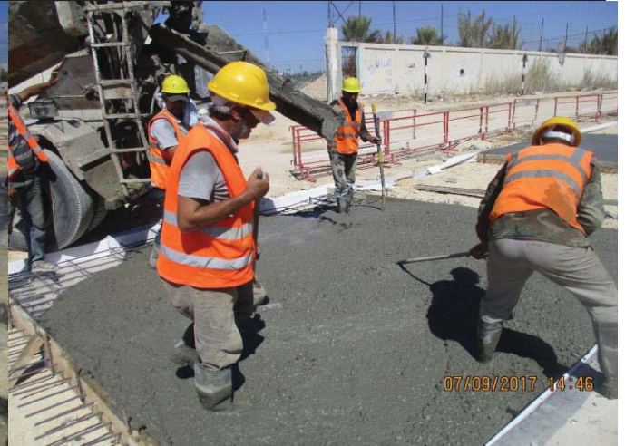
Photo No.14: Surface restoration work at paved concrete road (concrete leveling) Date: September 7, 2017
