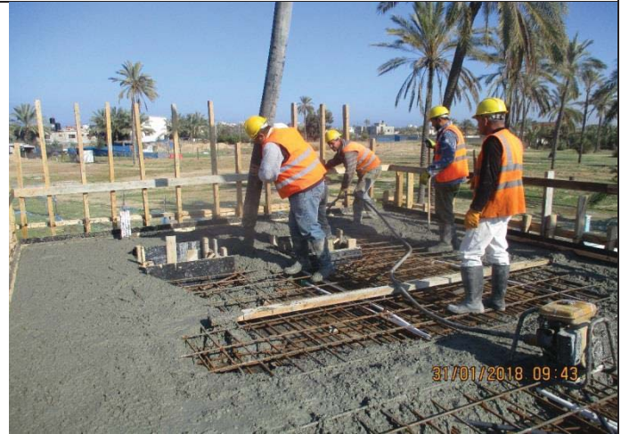
Photo No.48: Casting concrete for roof slab of electrical room Date: January 31, 2018
