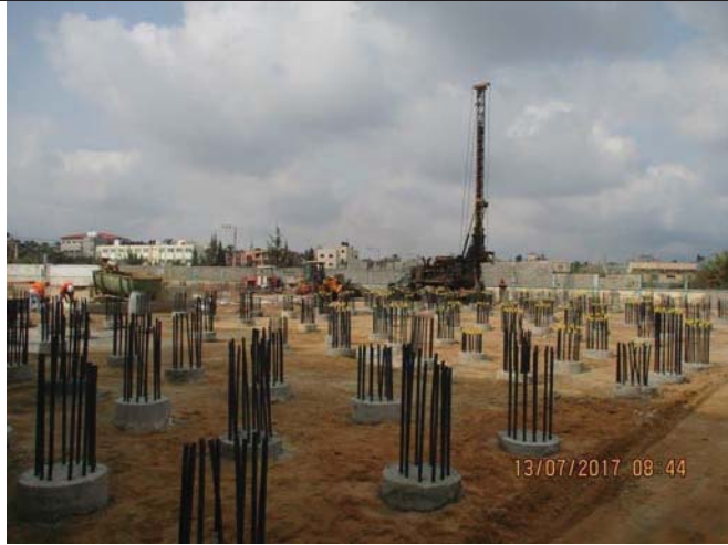
Photo No.15: Pile construction activity at the new RO building area. Date: July 13, 2017
