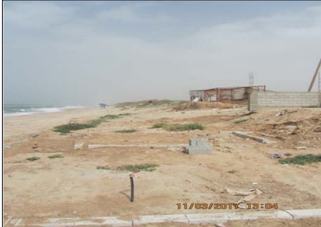
Photo No.05: Survey works to allocate proposed beach wells 01, 02 & 03 coordinates based on the new layout. Date: March 11, 2017
