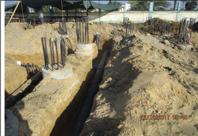
Photo No.45: Installation of PVC underground pipes prior to RO building. Date: October 22, 2017
