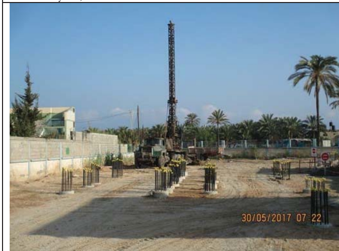
Photo No.15: Drilling and concrete reinforcement activities for the new RO building piles construction. Date: May 30, 2017
