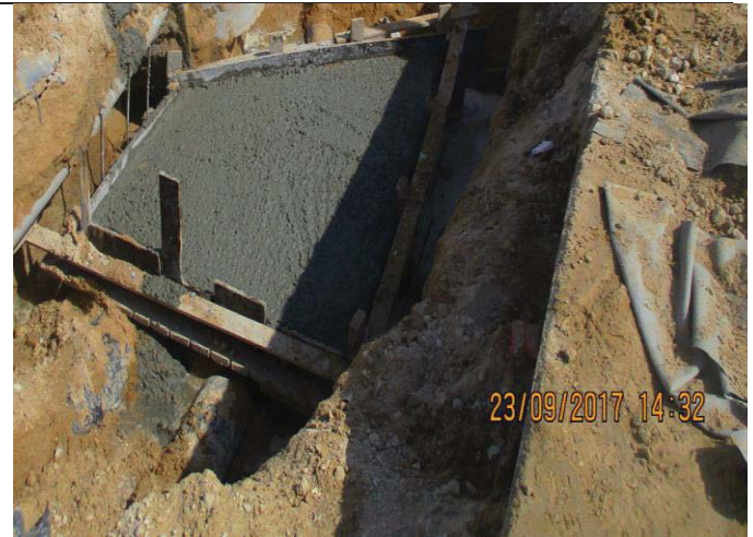
Photo No.32: Thrust block installation on outfall and intake pipelines Date: September 23, 2017
