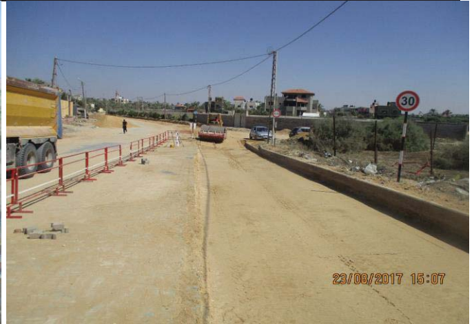
Photo No.50: Surface restoration work at interlock tile area (sub-base compaction). Date: August 23, 2017
