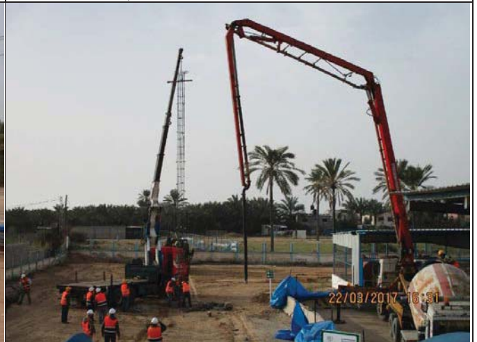
Photo No.22: Installation of reinforcement steel casing & supply & placement of concrete. Date: March 22, 2017
