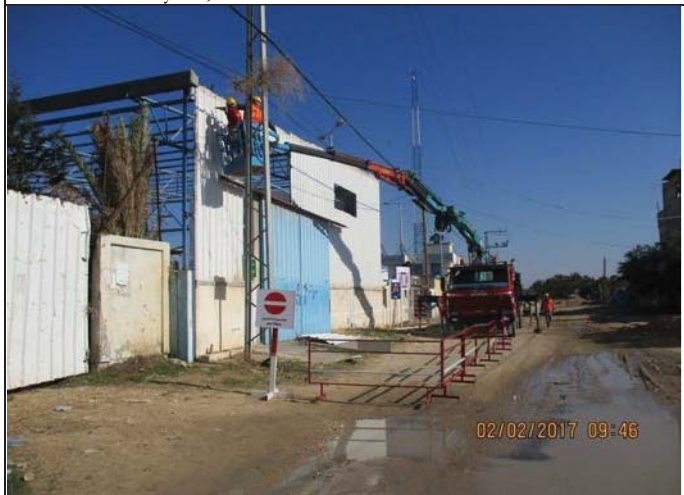
Photo No.03: Continue demolition works of existing steel canopy structure. Date: February 02, 2017
