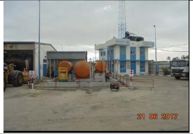
Photo No.14: Demolition of existing fuel tank and relocation of fuel tanks Date: June 21, 2017
