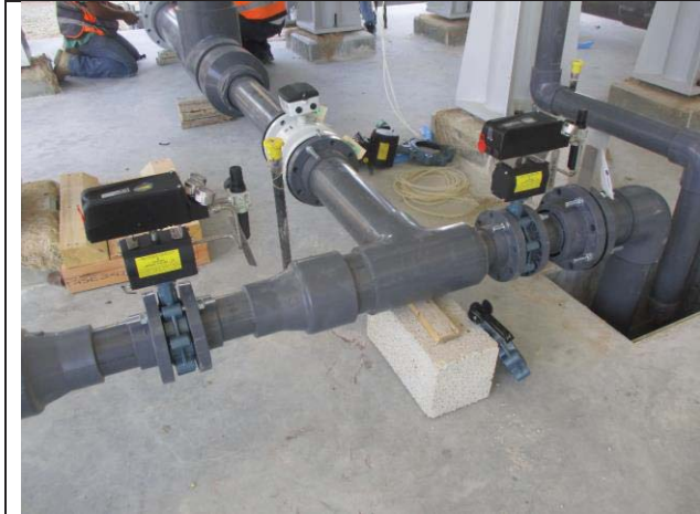
Photo No.19: Butterfly valve and flowmeter installation for DMF tanks Date: June 20, 2018
