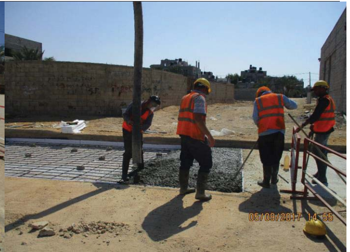
Photo No.02: Surface restoration work at paved concrete road (concrete casting) Date: September 5, 2017
