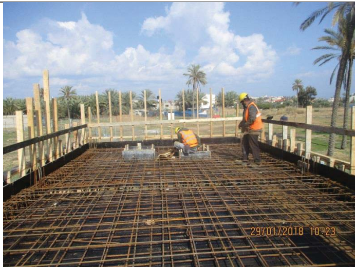
Photo No.39: shuttering works and steel reinforcement for roof slab of electrical room.
