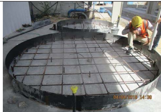
Photo No.09: Shuttering works, steel reinforcement HCL tank and NaOH tank pads Date: April 04, 2018
