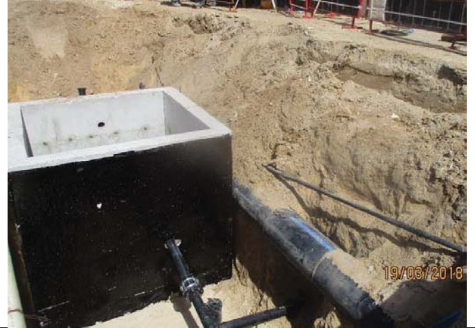
Photo No.20: Excavation works, chamber installation and backfilling works for washout chamber No.3 Date: March 19, 2018
