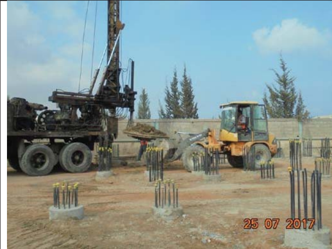
Photo No.37: Piles construction activity using Bentonite at the brine tank location. Date: July 25, 2017
