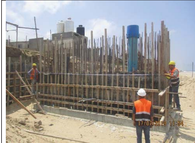
Photo No.19: Formwork and steel reinforcement for beach well retaining wall Date: July 17, 2018
