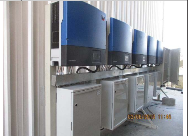
Photo No.04: Electrical works for PV system in pretreatment area Date: June 03, 2018
