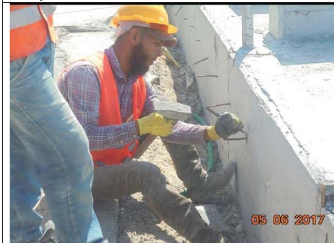
Photo No.05: Continue fuel tank base construction – removal of tie rods from walls and neck pads.
