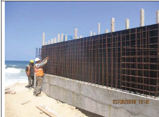
Photo No.21: Formwork and steel reinforcement for 2 nd part of retaining walls of beach Well No. 3 Date: August 27, 2018
