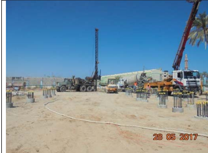
Photo No.13: Drilling and concrete reinforcement activities for the new RO building piles construction. Date: May 28, 2017
