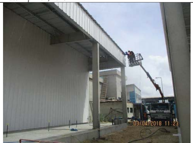
Photo No.06: Continue works in walls and roof panels of RO building Date: April 03, 2018
