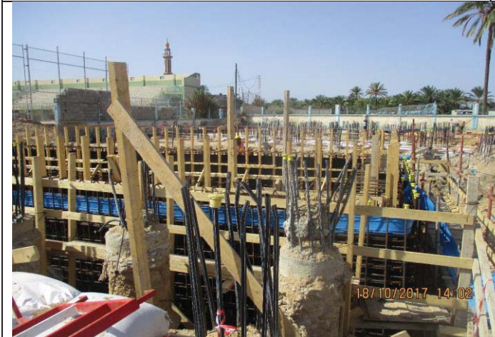
Photo No.35: Continue brine tank construction activities – formwork & steel reinforcement fabrication for tank walls. Date: October 18, 2017
