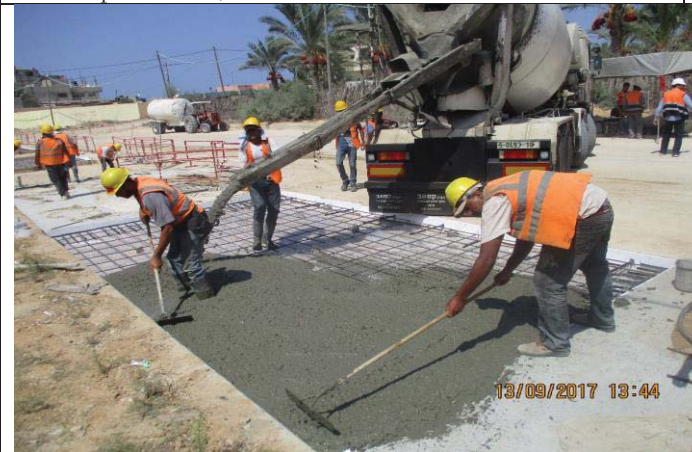
Photo No.23: Surface restoration work at paved concrete road (concrete casting) Date: September 13, 2017
