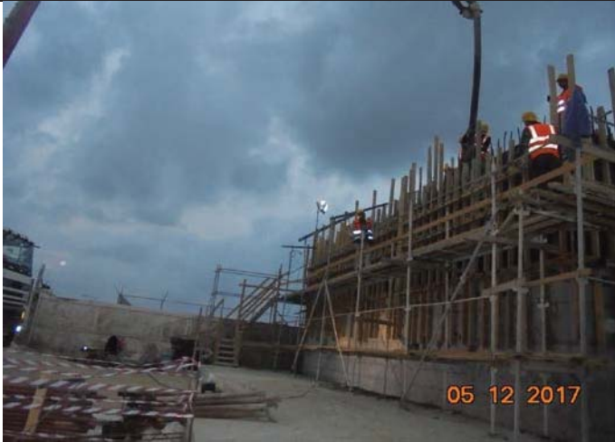
Photo No.09: Concrete casting for raw water and backwash tanks Date: December 05, 2017
