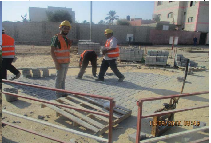
Photo No.28: Surface restoration work at paved interlock road (interlock works) Date: September 18, 2017
