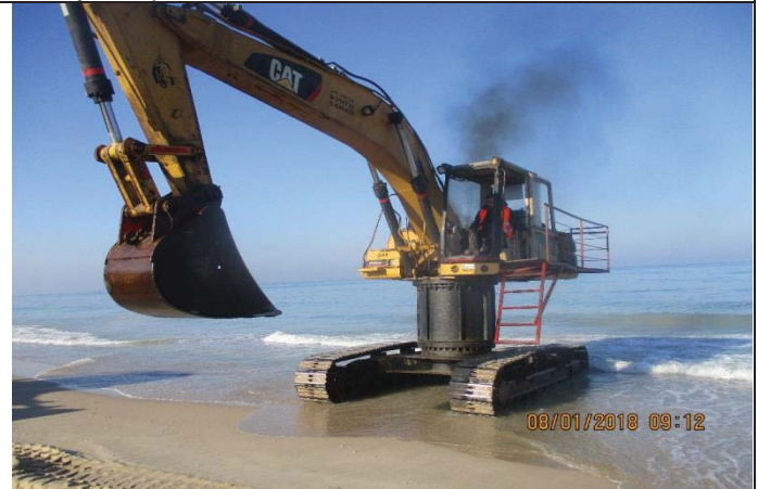
Photo No.08: Trial run and training for staff, working in outfall pipe installation on beach. Date: January 08, 2018
