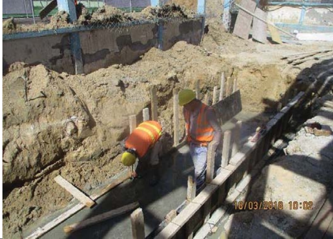
Photo No.17: Casting plain concrete for duct bank inside construction site. Date: March 18, 2018
