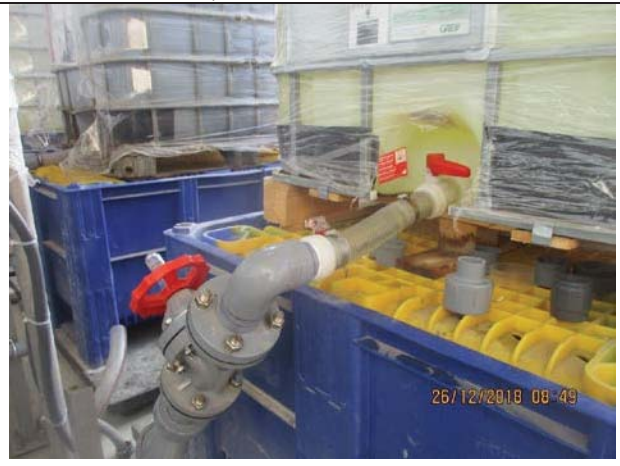
Photo No.24: IBC tanks connections Date: December 26, 2018
