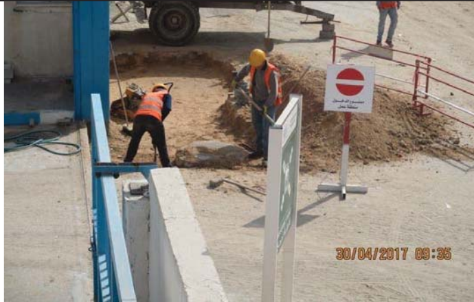
Photo No.25: Reinstatement works for storm water pipeline relocation (interlock segment). Date: April 30, 2017
