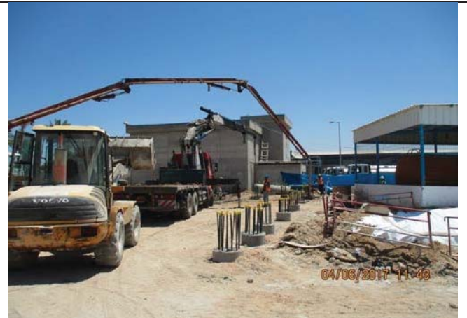
Photo No.02: Piles reinforced concrete casting at the new RO building area.
