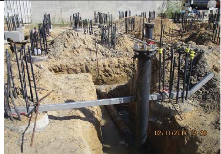
Photo No. 06: PVC Pipe SCH 80, 10-inch pipe R.O underground 1st and 2nd pass dump preparation Date: November 02, 2017
