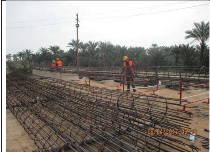
Photo No.11: Continue fabricating reinforcement steel casing for piles at storage yard. Date: April 09, 2017
