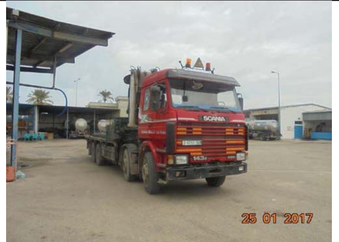
Photo No.06: Mobile Crane (SCANIA, 1996) used for demolition of existing steel canopy structure. Date: January 25, 2017
