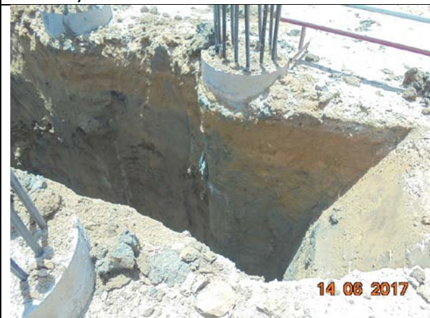
Photo No.09.2: Piles integrity test (I2L, I2M, I3L & I3M) at pre-treatment building. Date: June 14, 2017
