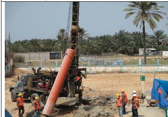
Photo No.25: Excavation for 600 mm diameter piles (R10, Type- L, Depth- 16 lm) using surface casing.
