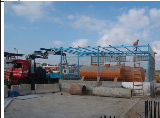
Photo No.11: Demolition and relocation works for the existing fuel tank – demolish of steel structure. Date: June 15, 2017
