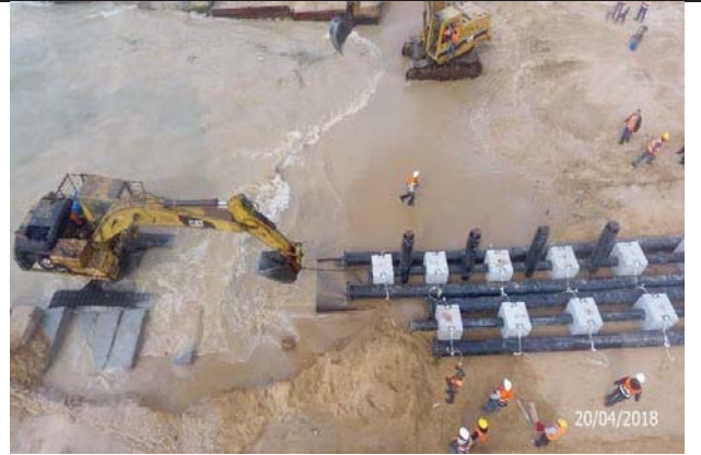
Photo No.26: Supply and installation of 315 mm HDPE pipeline for outfall pipeline from St. 2+045 to St. 2+130. Date: April 20, 2018
