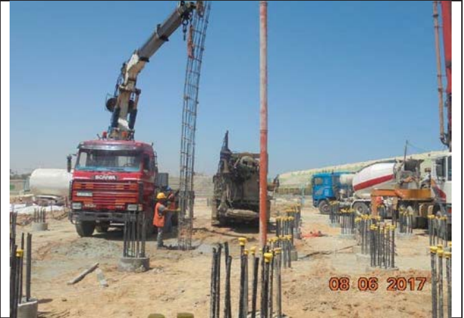
Photo No.08: Pile construction activity at the new RO building area. Date: June 08, 2017
