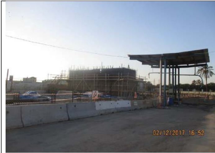
Photo No.01: Site Securing, completely with steel fence and concrete barriers with signs of No-Entry. December 02, 2017
