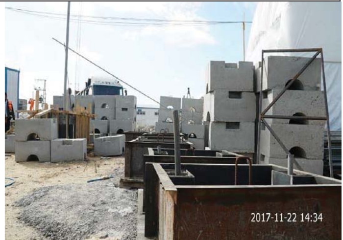
Photo No. 34: Outfall pipe line casted weight collars, navigation signs Date: November 22, 2017
