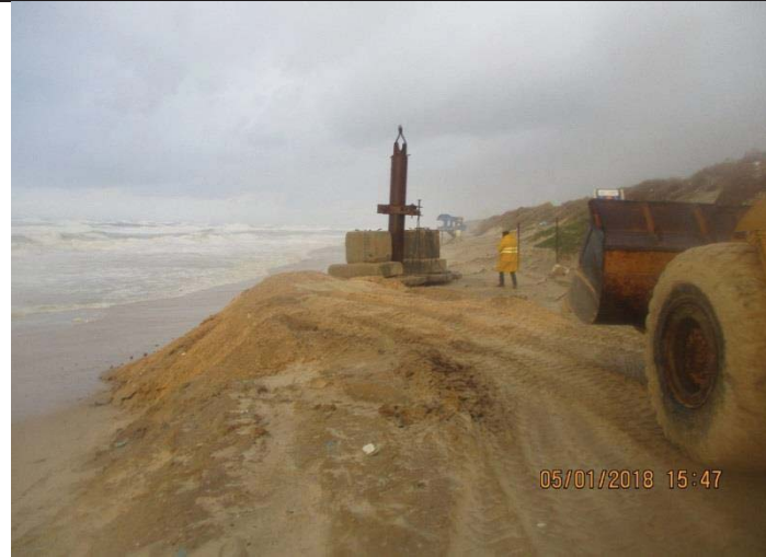
Photo No.05: Repair works due to the heavy windy storm and the rainy weather. Date: January 05, 2018
