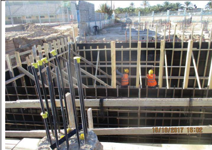
Photo No.29: Continue brine tank construction activities – formwork for tank walls. Date: October 15, 2017
