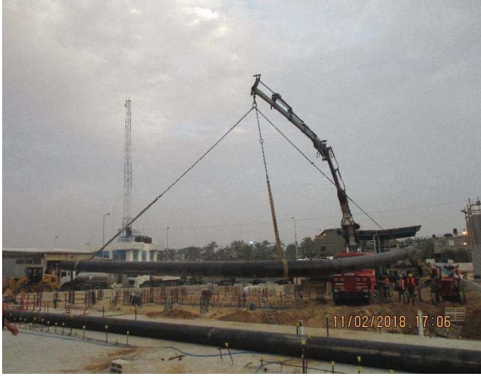
Photo No.17: supply and install all HDPE piping, fittings, and associated appurtenances for outfall and intake pipelines Date: February 11, 2018
