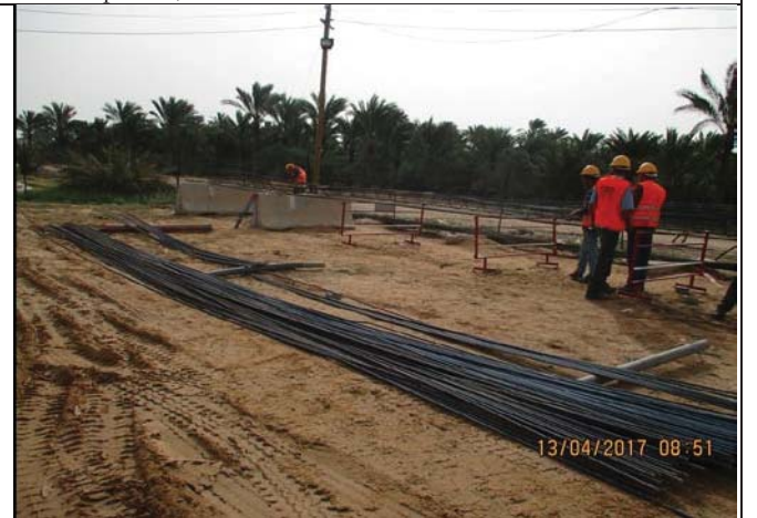
Photo No.14: Preparation of reinforcing steel structure for piles in storage yard. Date: April 13, 2017
