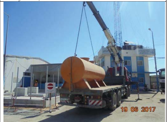
Photo No.12: Continue demolition of existing fuel tank and diesel tanks relocation prior to fuel tank relocation activity. Date: June 19, 2017
