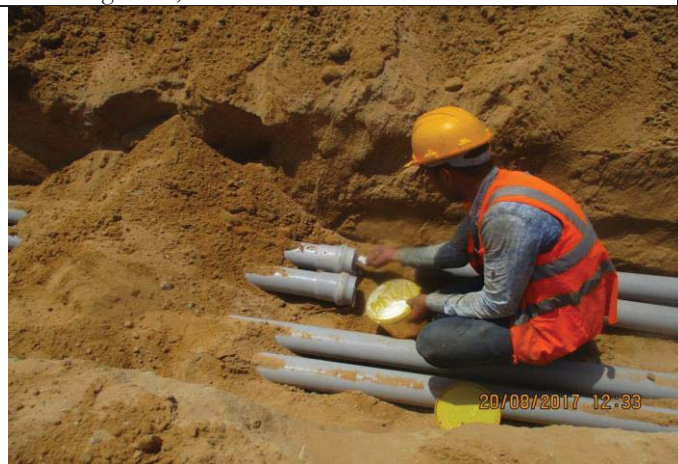
Photo No.47: Electrical conduit laying for MV and fiber optic cable (conduit connection). Date: August 20, 2017
