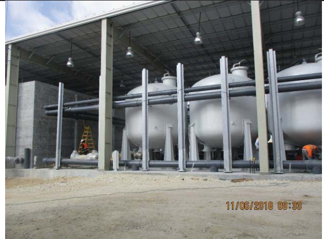
Photo No.14: Continue fabrication of PVC manifolds for dual media filter tank Date: June 11, 2018
