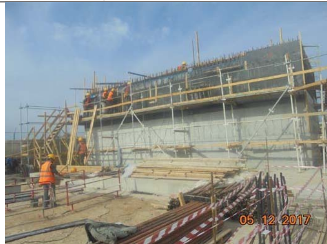
Photo No.08: External formwork completion for raw water and backwash tanks Date: December 05, 2017
