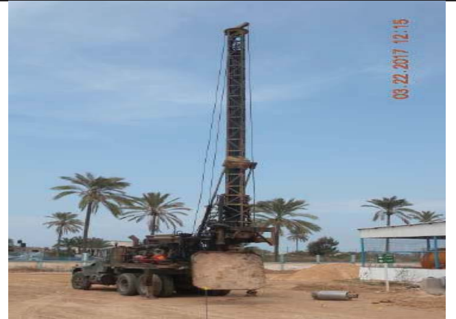
Photo No.18: Pile drilling at the new pre-treatment building area (R06, type L, 16 lm depth). Date: March 22, 2017
