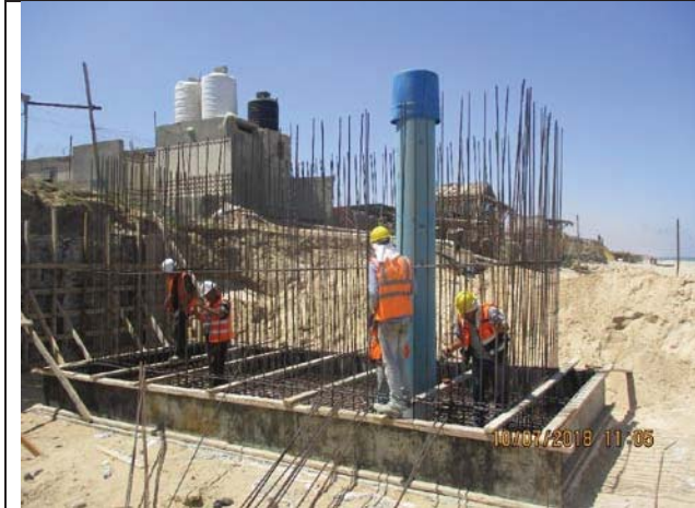
Photo No.13: Formwork & steel reinforcement for beach well retaining wall foundation Date: July 10, 2018
