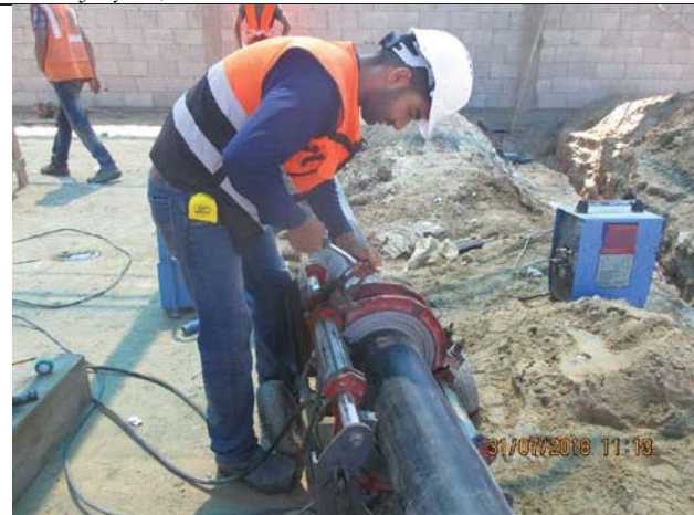
Photo No.41: HDPE pipe connection for beach well No. 1 from asphalt road to beach well room Date: July 31, 2018
