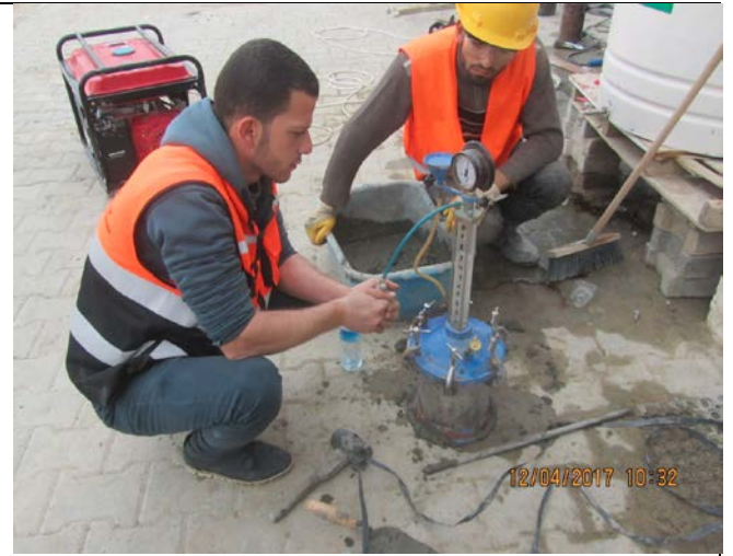
Photo No.06.2: Quality control tests on received concrete job mix in presence of CCQC lab (air content test). Date: April 12, 2017
