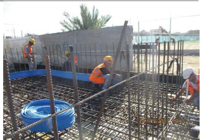
Photo No. 02: Raw water and backwash tanks (steel reinforcing and electrical works)
