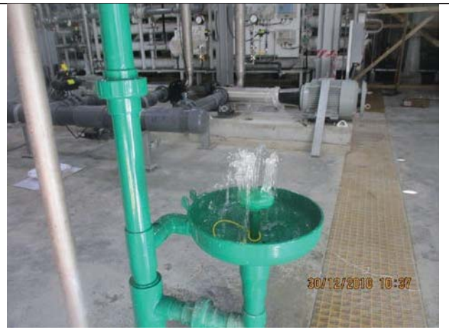
Photo No.30: Running emergency eye wash Date: December 30, 2018
