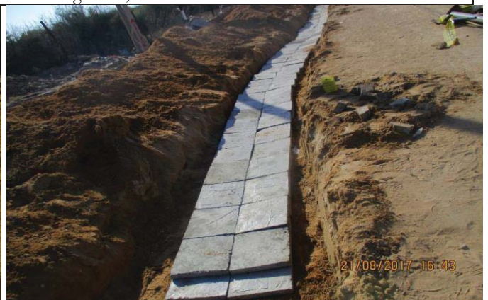
Photo 54: Electrical conduit manhole laying for MV and fiber optic cable (concrete block placement). Date: August 21, 2017
