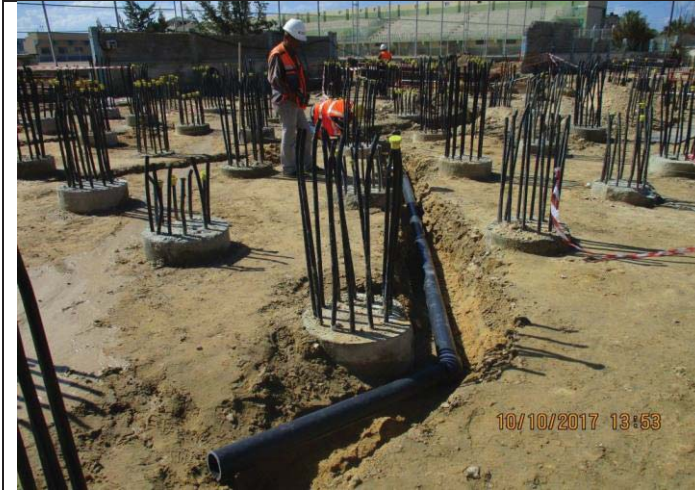
Photo No.13: Welding and fabricating embedded underground pipes in the pre-treatment – PVC pipes. Date: October 10, 2017
