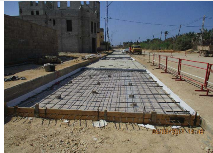
Photo No.01: Surface restoration work at paved concrete road (steel reinforcement) Date: September 5, 2017
