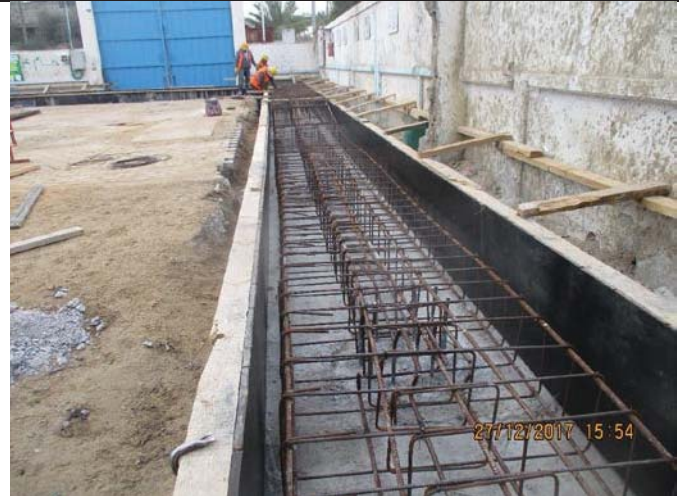
Photo No.48: De-shuttering works and steel reinforcement of the workshop area ground beams Date: December 27, 2017
