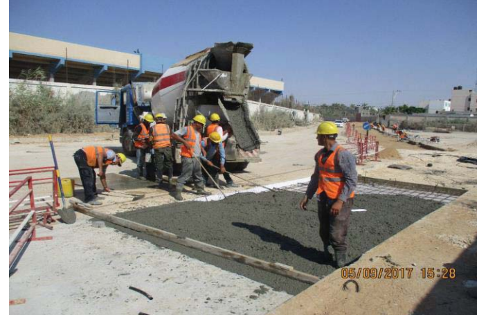
Photo No.03: Surface restoration work at paved concrete road (surface leveling.) Date: September 5, 2017
