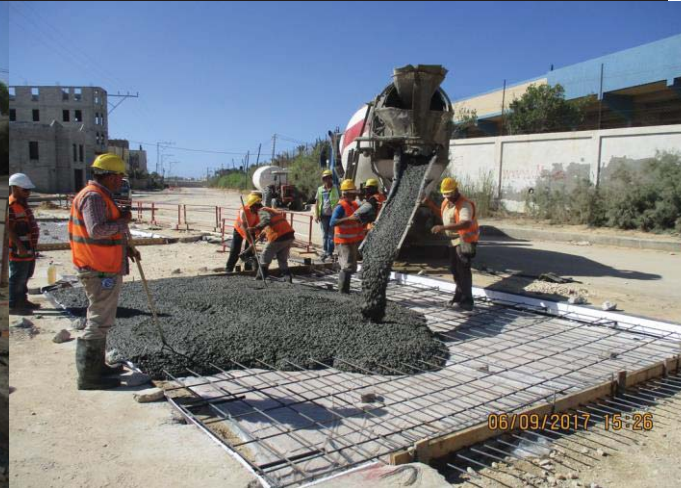
Photo No.08: Surface restoration work at paved concrete road (concrete casting) Date: September 6, 2017
