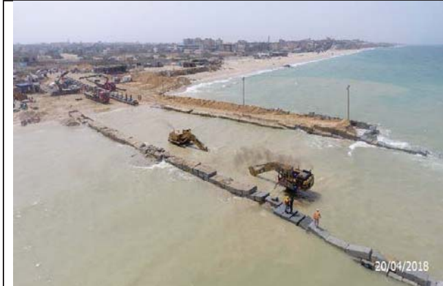
Photo No.25: Excavation works for outfall pipeline from St. 2+045 to St. 2+130. Date: April 20, 2018
