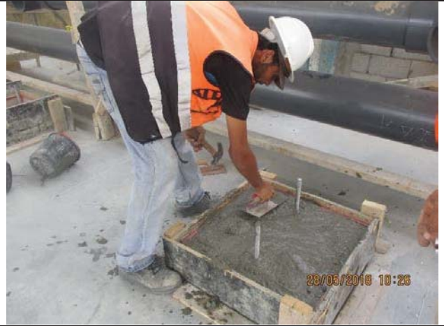
Photo No.26: Formwork and casting concrete for dual media filter tank pads. Date: May 28, 2018
