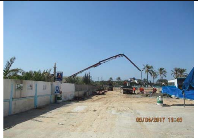
Photo No.08: Supply and cast-in-place concrete using tremie pipes up to end of the pile. Date: April 05, 2017
