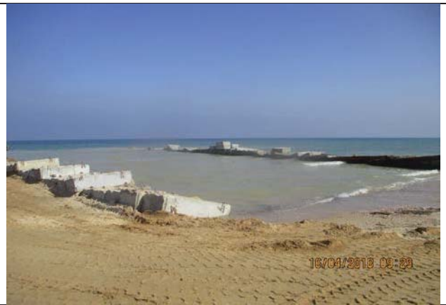
Photo No.22: Stopped preparation works of outfall pipeline installation due to instructions from local authorities Date: April 16, 2018
