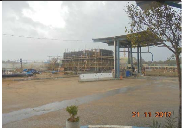
Photo No. 26: Raw water works suspended due to heavy rain. Date: November 21, 2017
