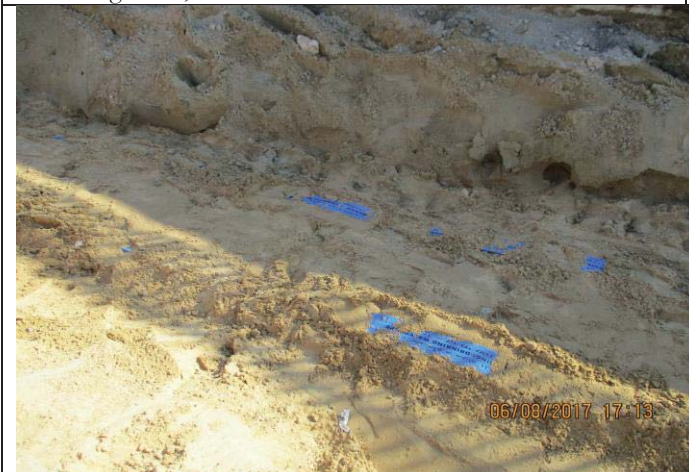
Photo No.17: Pipeline construction activity (warning tape & backfill the 30 cm above the pipeline). Date: August 06, 2017
