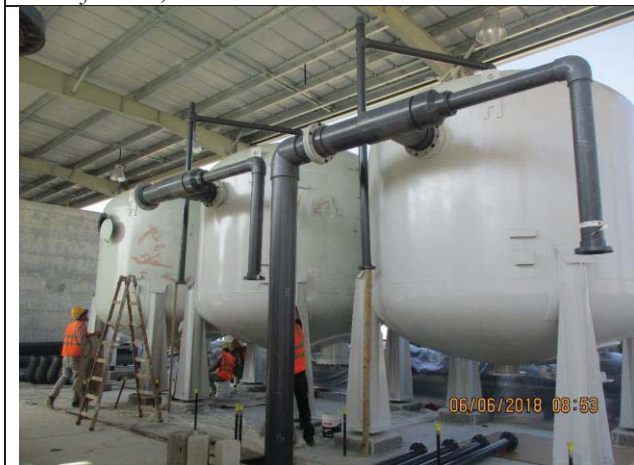
Photo No.11: Start installation of prefabricated PVC manifolds for dual media filter tanks Date: June 06, 2018
