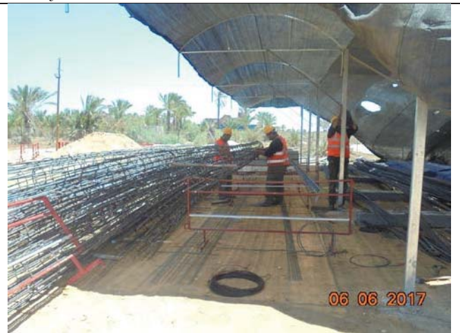
Photo No.06: Continue fabricating reinforcement steel case for piles at storage yard.
