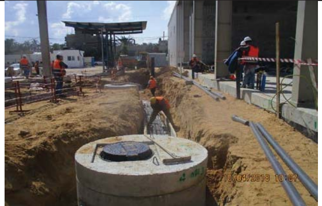
Photo No.14: Excavation works, steel reinforcement, electrical conduits installation and casting concrete for duct banks inside construction site. Date: April 10, 2018
