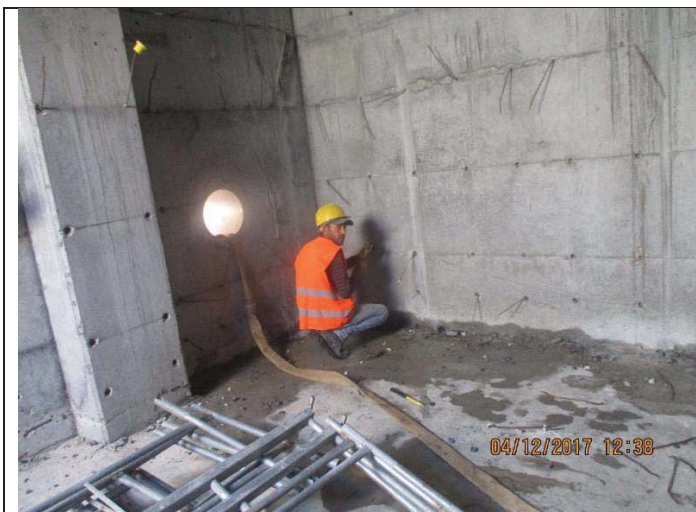
Photo No.05: Preparation of internal surfaces of brine tank walls. Date: December 04, 2017
