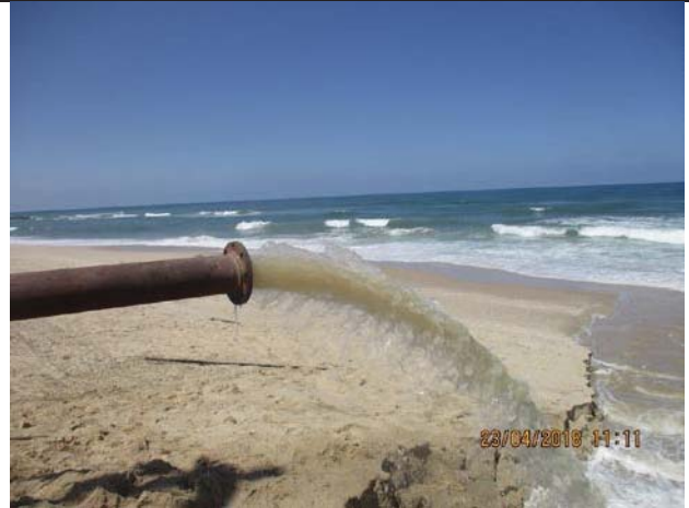
Photo No.34: Cleaning and test works for beach well No.1 Date: April 23, 2018
