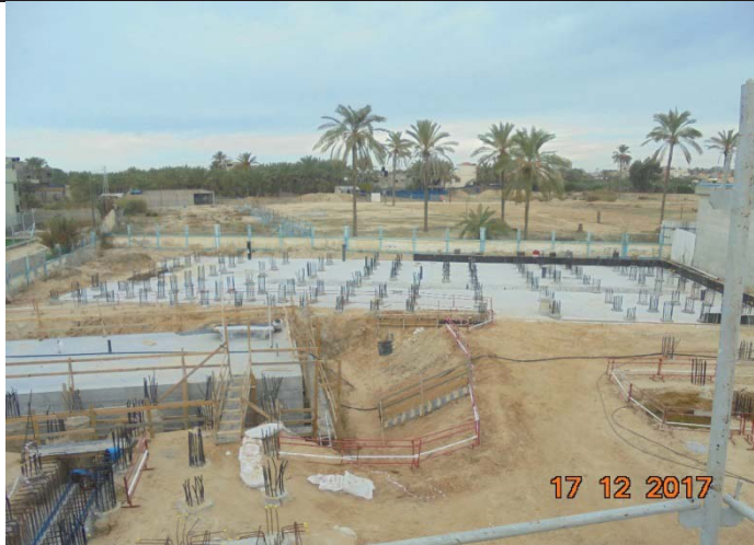
Photo No.35: Desalination plant site housekeeping and brine tank filling work. Date: December 17, 2017
