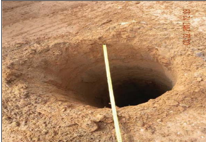
Photo No.19: Pile drilling at the new pre-treatment building area (R06, type L, 16 lm depth). Date: March 22, 2017
