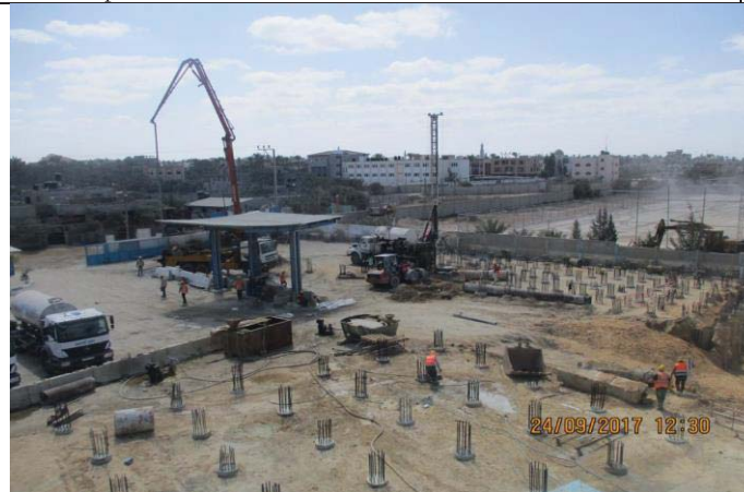
Photo No.35: Pile construction activity prior to works, back wash and raw water tanks. Date: September 24, 2017
