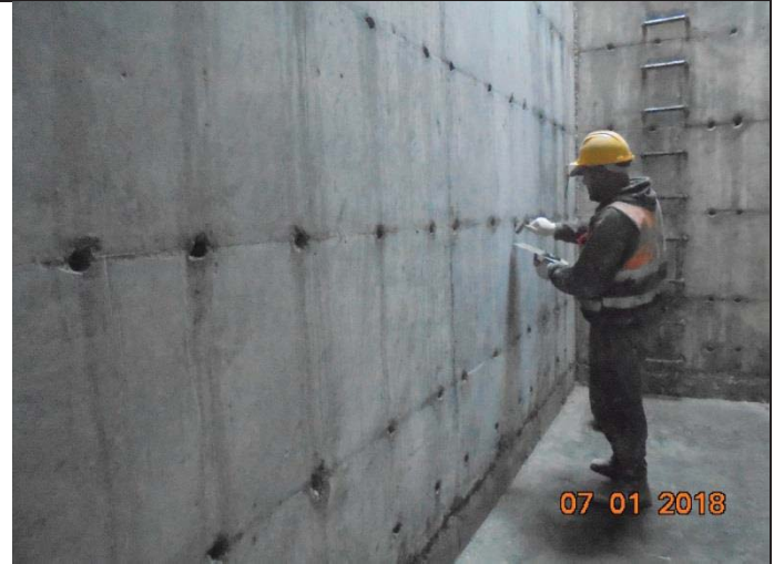
Photo No.06: Repairing works for internal walls of backwash/raw water tanks. Date: January 07, 2018
