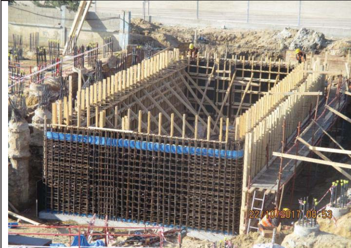
Photo No.43: Continue brine tank construction activities – formwork & steel reinforcement fabrication for tank walls. Date: October 22, 2017
