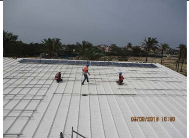
Photo No.08: Start installing PV system on the RO canopy. Date: May 05, 2018
