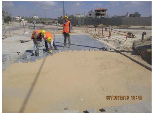
Photo No.12: Tiling works for reinstatement works from St. 1+500 to St. 1+550. Date: August 07, 2018
