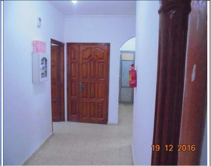
Photo No.14: Firefighting system and first aid inspection at Engineers office Date: December 19, 2016
