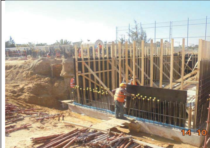
Photo No.25: Continue brine tank construction activities – formwork for tank walls Date: October 14, 2017
