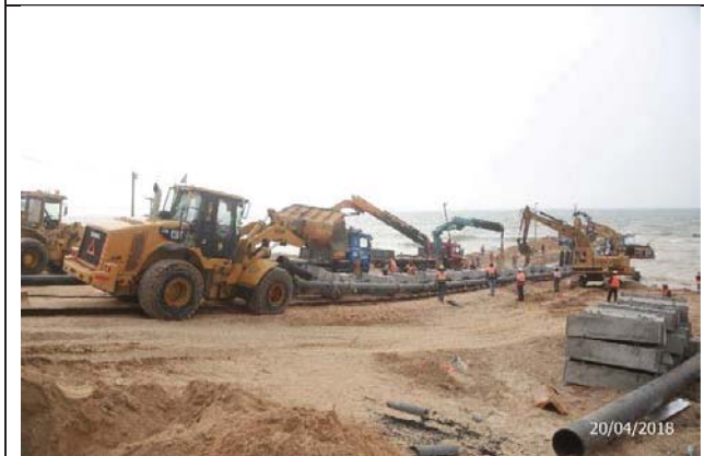
Photo No.27: Supply and installation of 315 mm HDPE pipeline for outfall pipeline from St. 2+045 to St. 2+130. Date: April 20, 2018
