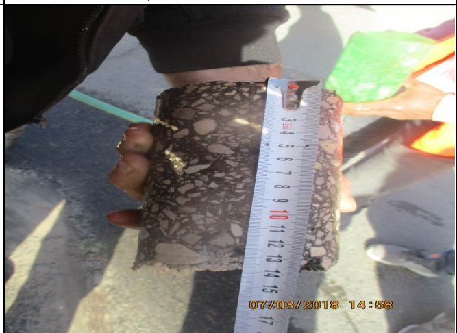
Photo No.14.2: Taking sample for reinstatement works in Al Rasheed ST. for core test Date: March 07, 2018
