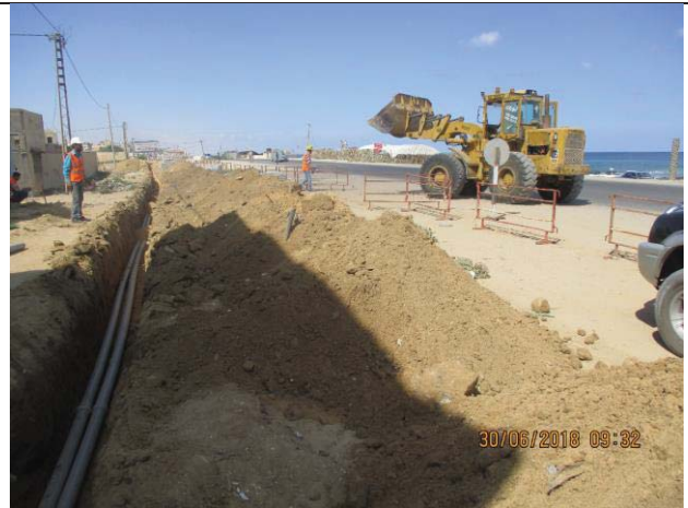
Photo No.34: Electrical manhole and conduits installation for beach wells Date: June 30, 2018
