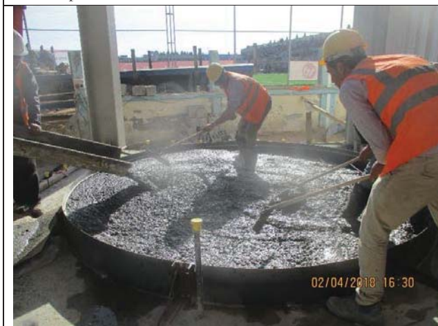
Photo No.05: Shuttering works, steel reinforcement and casting concrete for RO flushing tank pad and neutralization tank pad. Date: April 02, 2018
