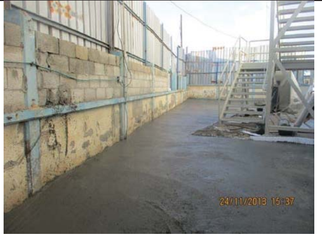
Photo No.14: Casting concrete for concrete sidewalk beside RO Building Date: November 24, 2018
