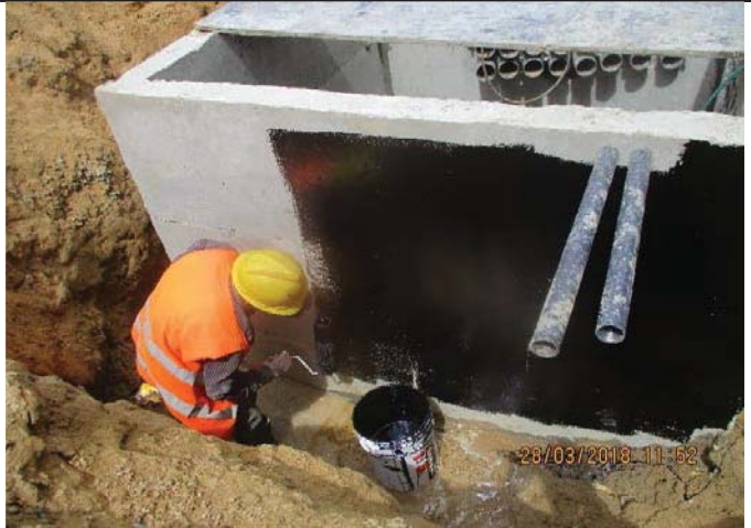
Photo No.30: Epoxy coating for the external face of electrical manholes Date: March 28, 2018
