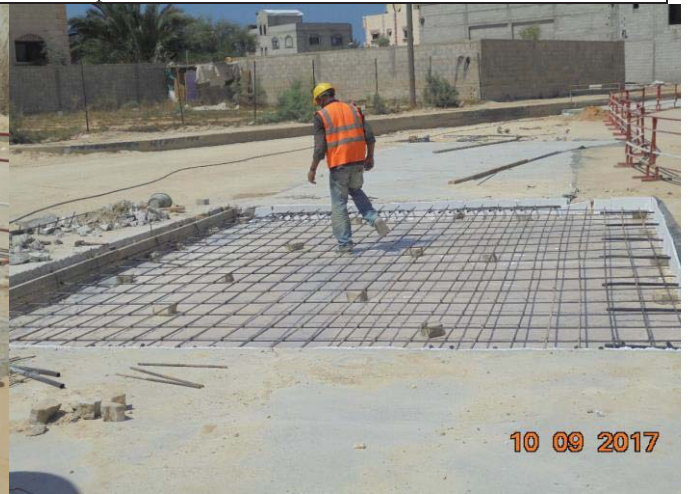
Photo No.16: Surface restoration work at paved concrete road (reinforcement works) Date: September 10, 2017
