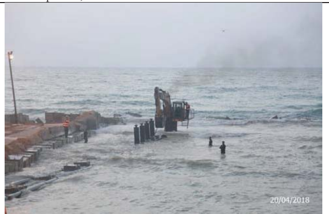
Photo No.28: Supply and installation of 315 mm HDPE pipeline for outfall pipeline from St. 2+045 to St. 2+130. Date: April 20, 2018
