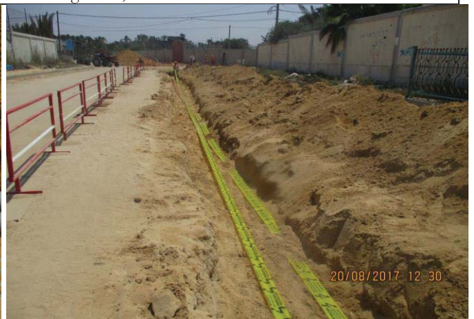
Photo No.48: Electrical conduit laying for MV and fiber optic cable (warning tape). Date: August 20, 2017
