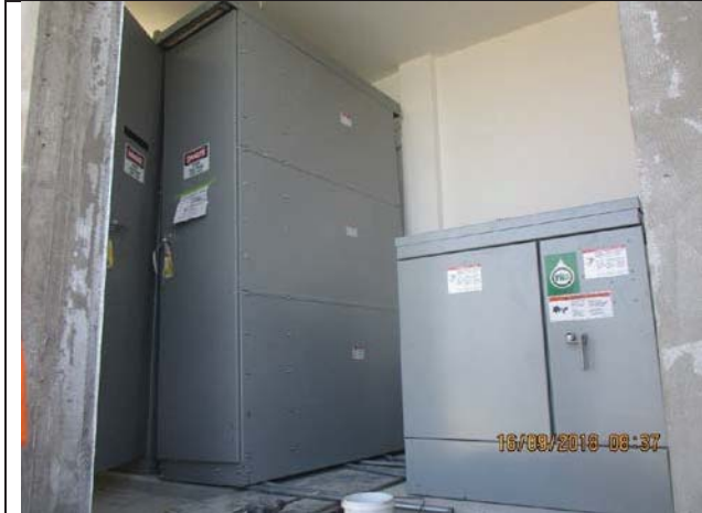
Photo No.19: Installation works for electrical boards inside beach well electrical room. Date: September 16, 2018
