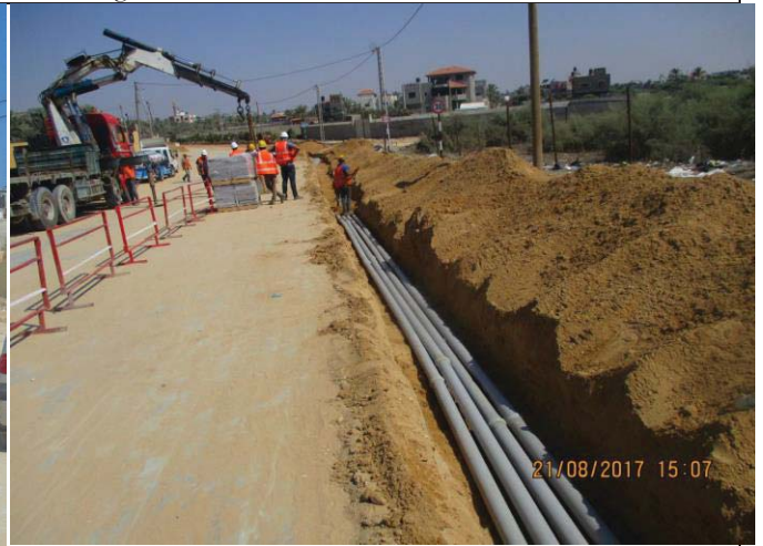
Photo 52: Electrical conduit laying for MV and fiber optic cable (conduit laying). Date: August 21, 2017
