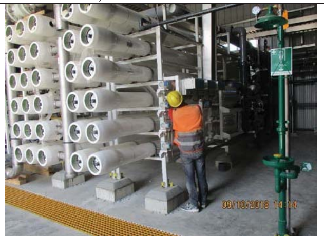
Photo No.06: Instrumentation connections Date: October 09, 2018
