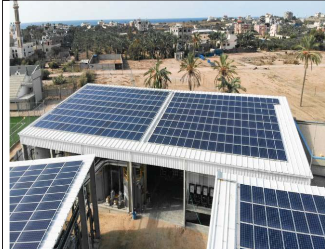
Photo No.13: Solar system Date: October 21, 2018
