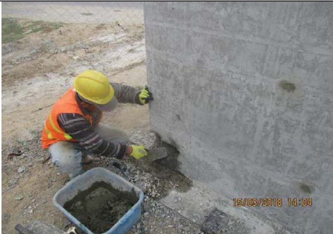
Photo No.13: Preparation works for mechanical chambers before epoxy coating. Date: March 15, 2018
