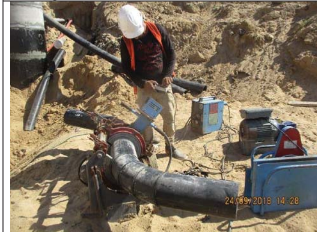
Photo No.27: Connection works for 200 mm HDPE pipes to Beach Well No. 2. Date: September 24, 2018
