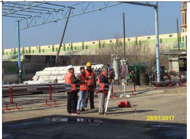
Photo No.10: Walk-through and surveying works for brine line demolition and relocation Date: January 29, 2017
