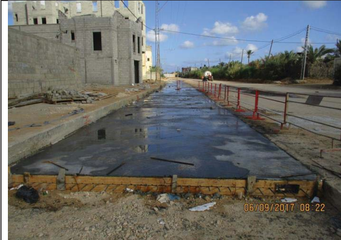
Photo No.07: Surface restoration work at paved concrete road (curing previously casted) Date: September 6, 2017
