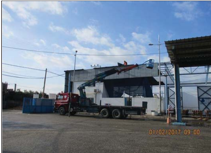
Photo No.01: Continue demolition works of existing steel canopy structure. Date: February 01, 2017
