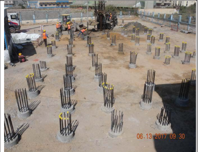
Photo No.10: Piles construction at the new RO building area. Date: June 13, 2017
