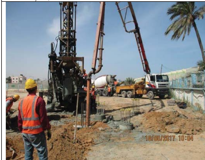
Photo No.09: Drilling and concrete reinforcement activities for the new RO building piles construction. Date: May 18, 2017
