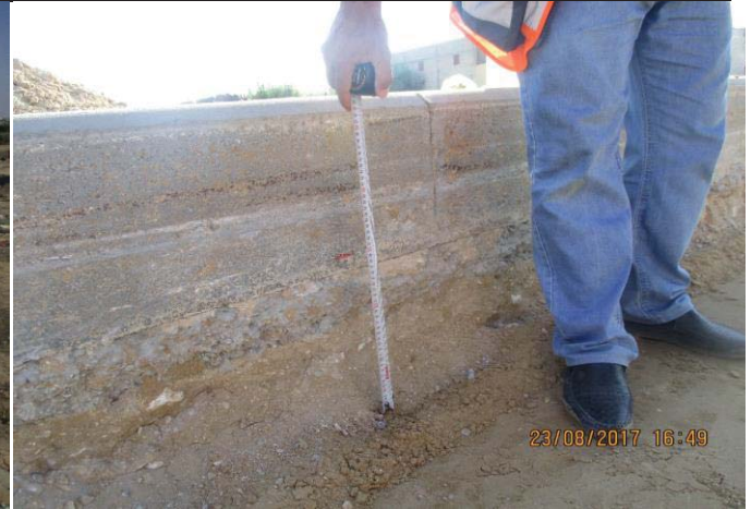
Photo No.56: Surface restoration work at interlock tile area (trench dimensions). Date: August 23, 2017
