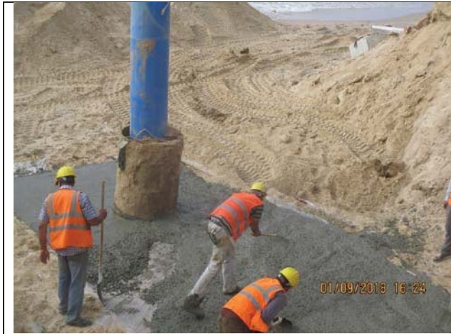
Photo No.01: Casting concrete for plain concrete of the foundation of beach well No.2 retaining wall Date: September 01, 2018
