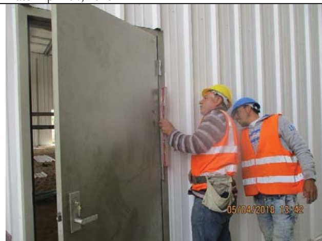
Photo No.11: Accessories installation for steel structures (doors, louvers... etc.) Date: April 05, 2018
