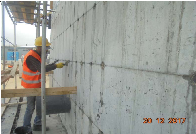
Photo No.39: Repair works for external walls of backwash tanks Date: December 20, 2017
