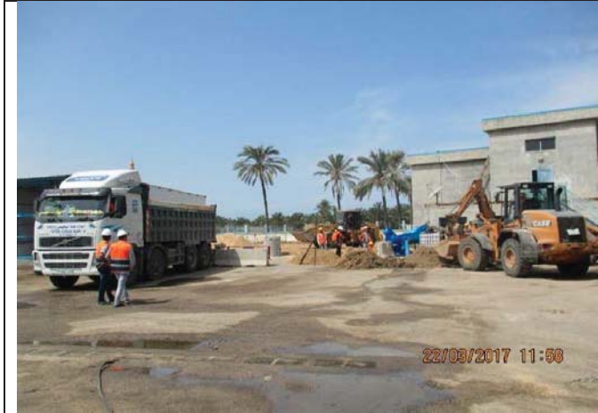
Photo No.17: Brine line relocation excavation, bedding, pipe installation & backfilling. Date: March 22, 2017
