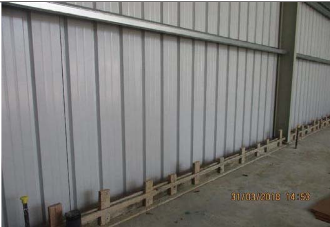
Photo No.33: Shuttering works and steel reinforcement for concrete ground beams on RO pad Date: March 31, 2018
