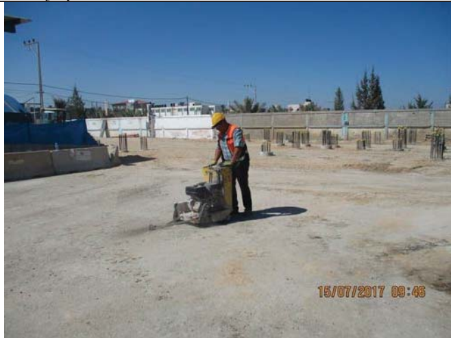
Photo No.21: Asphalt cutting prior to piles construction at the new generator pad area. Date: July 15, 2017
