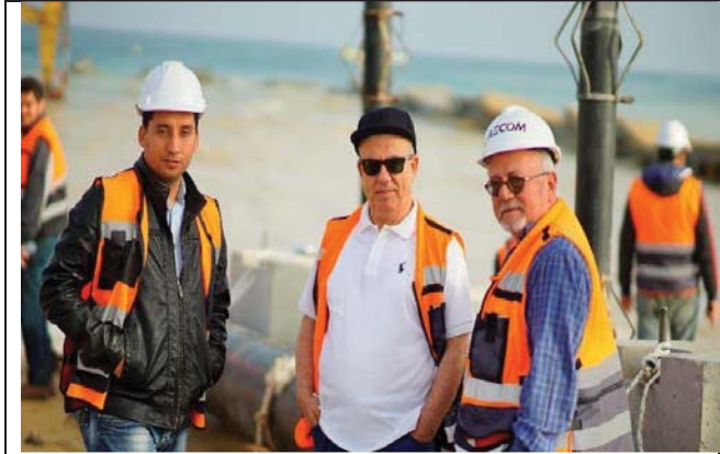
Photo No.31: USAID, AECOM & BES representatives monitoring the supply and installation of 315 mm HDPE pipeline for outfall pipeline from St. 2+045 to St. 2+130. Date: April 20, 2018
