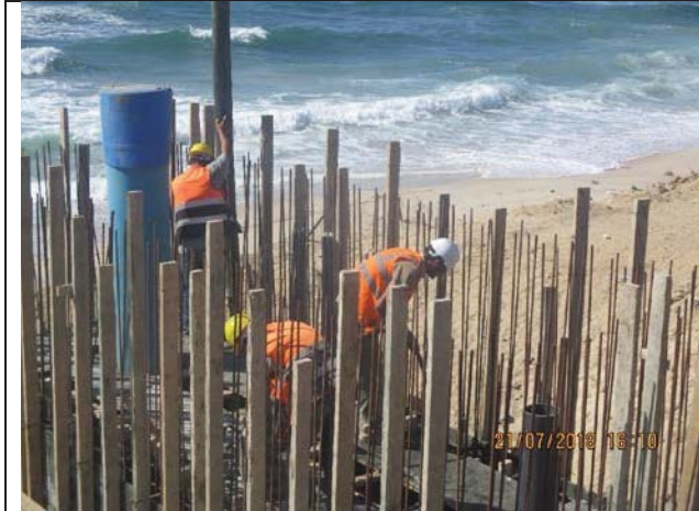
Photo No.25: Casting concrete for beach well No. 3 retaining wall Date: July 21, 2018
