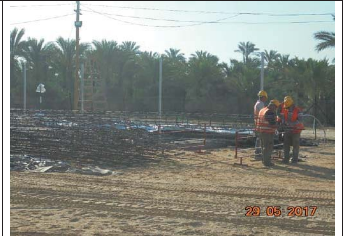
Photo No.14: Continue fabricating reinforcement steel case for piles at storage yard. Date: May 29, 2017
