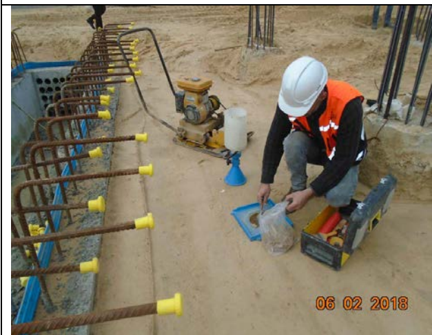
Photo No.13.2: Field quality control test for generator pad trench Date: : February 06, 2018
