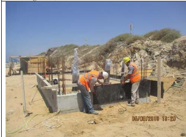
Photo No.09: Formworks and steel reinforcement for concrete pad of beach well electrical room. Date: August 05, 2018
