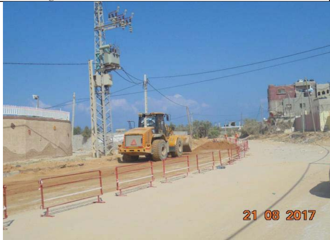
Photo 51: Electrical conduit laying for MV and fiber optic cable (excavation). Date: August 21, 2017
