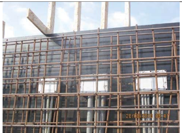
Photo No.24: Formwork, electrical first fix, and steel reinforcement for 2 nd part of retaining walls of beach well No. 3 Date: August 28, 2018
