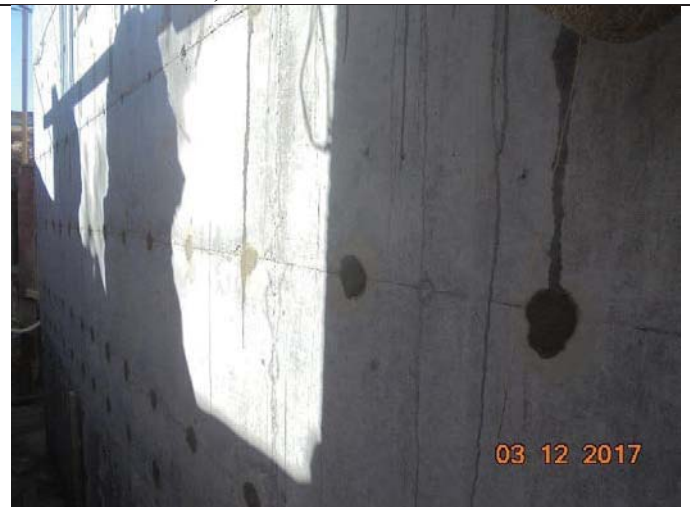
Photo No.04: Preparation of external surfaces for the brine tank before coating Date: December 03, 2017
