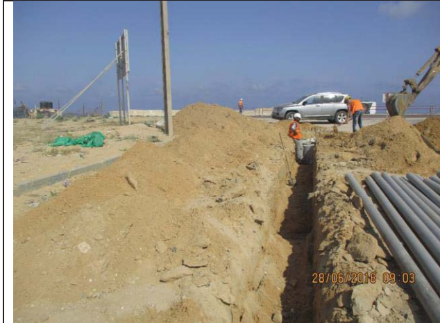
Photo No.31: Electrical manhole and conduits installation for beach wells Date: June 28, 2018
