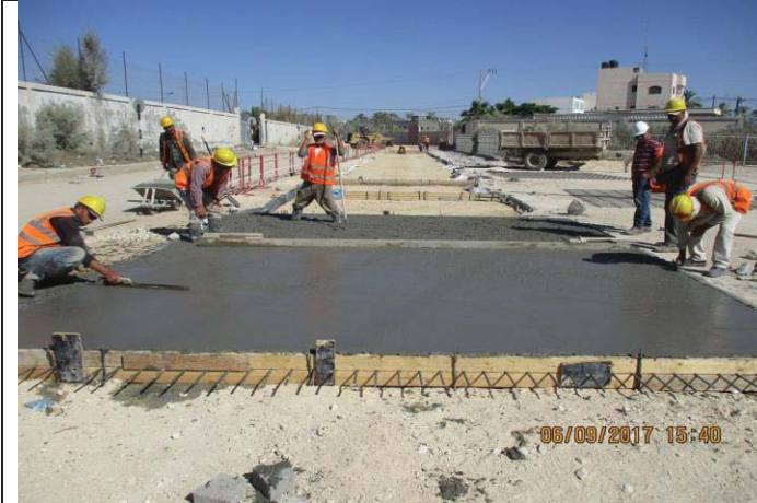
Photo No.09: Surface restoration work at paved concrete road (concrete leveling) Date: September 6, 2017
