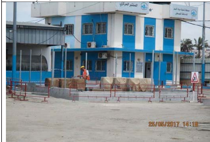
Photo No.11: Curing of the previously casted fuel tank neck pads. Date: May 25, 2017
