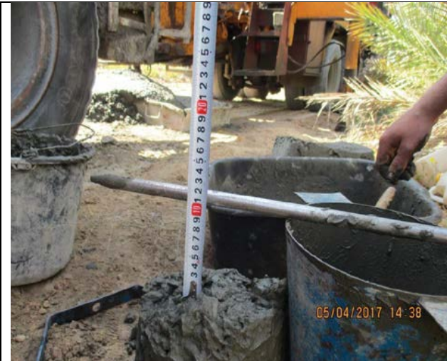
Photo No.05.2: Field control tests by CCQC Lab for cast-in-place concrete for piles R07 & R14-Slump test Date: April 05, 2017
