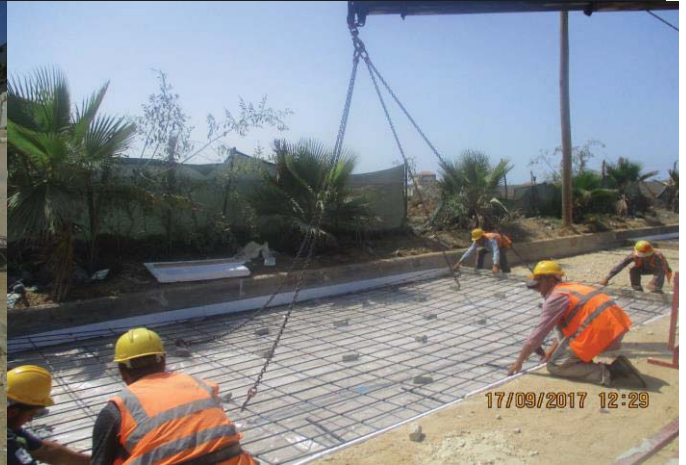
Photo No.26: Surface restoration work at paved concrete road (reinforcement works) Date: September 17, 2017
