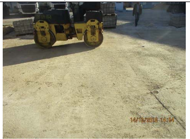
Photo No.16: Compaction for base course layer for site yard interlock tiling. Date: December 14, 2018
