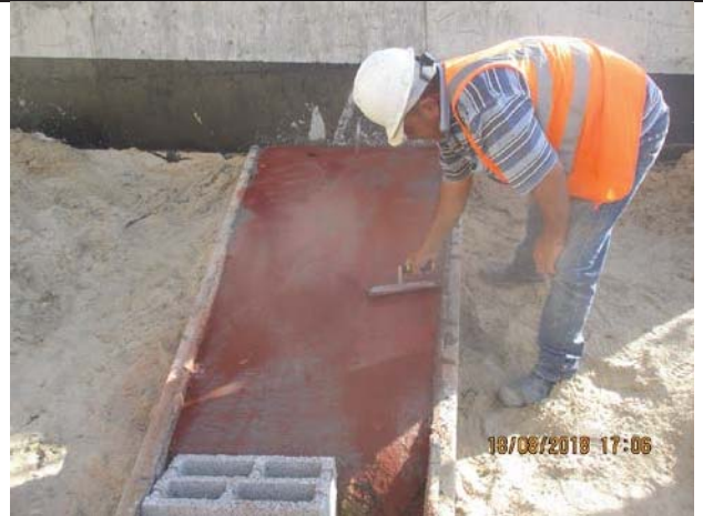
Photo No.20: Casting concrete for duct bank for beach wells. Date: August 18, 2018
