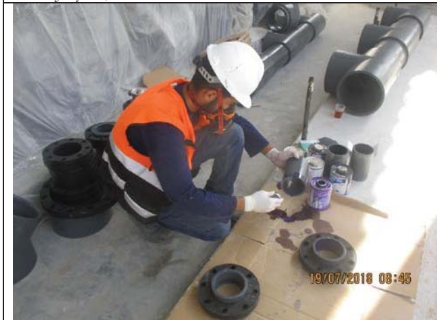
Photo No.21: Fabrication of PVC manifolds For 2 nd pass feed pump Date: July 19, 2018
