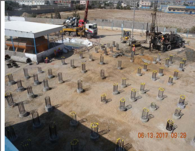
Photo No.09: Piles construction at the new RO building area. Date: June 13, 2017
