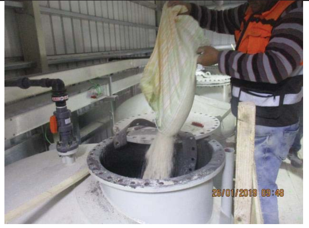
Photo No.20: Limestone filling inside calcite contactors Date: January 26, 2019
