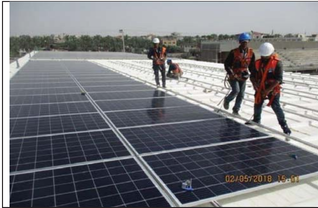
Photo No.01: Continue installing PV system on the pretreatment canopy. Date: May 02, 2018
