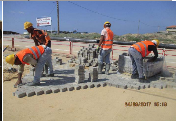
Photo No.58: Surface restoration work at interlock tile area (interlock restoration work). Date: August 24, 2017
