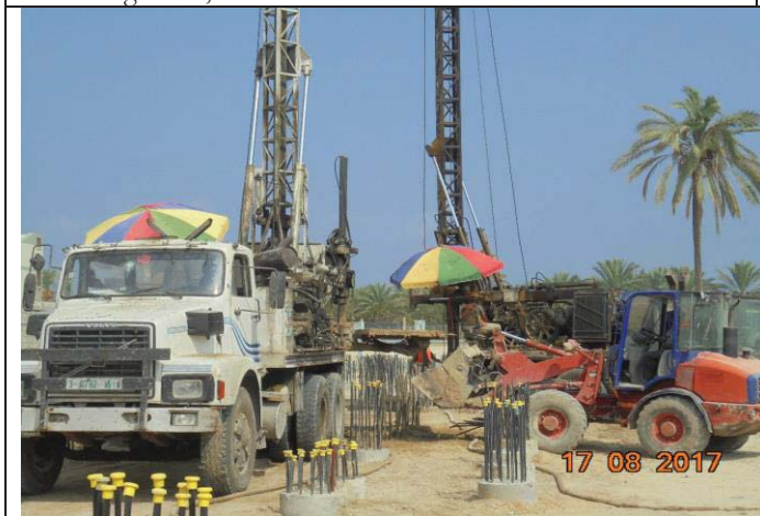
Photo No.39: Pile construction activity (pile drilling at brine tank and pre-treatment building) Date: August 17, 2017
