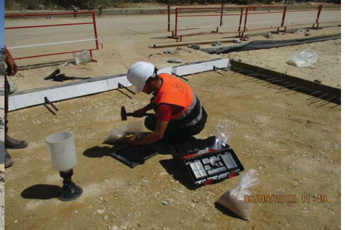
Photo No.10: Surface restoration work at paved concrete road (field density test) Date: September 6, 2017
