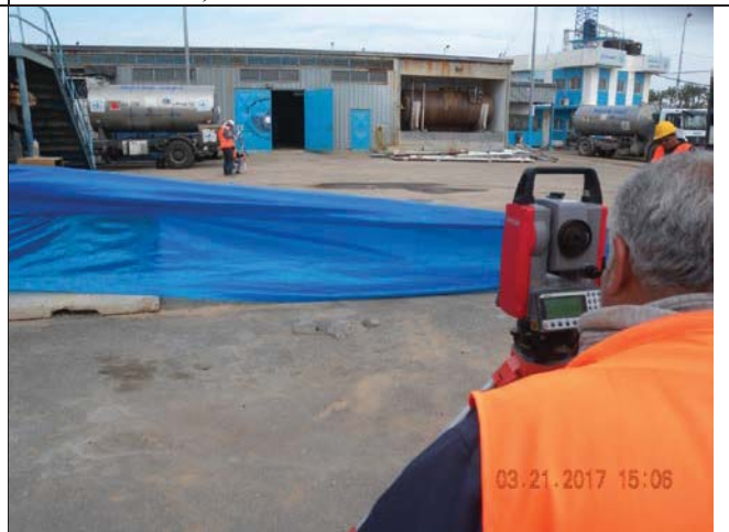
Photo No.16: Surveying works for brine line relocation & piles of pre-treatment building. Date: March 21, 2017
