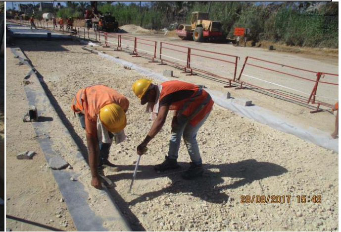
Photo No.70: Surface restoration work at paved concrete road (filling aggregate base). Date: August 28, 2017
