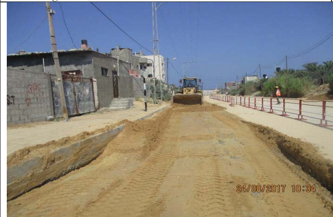
Photo No.59: Surface restoration work at interlock tile area (subgrade base preparation). Date: August 24, 2017
