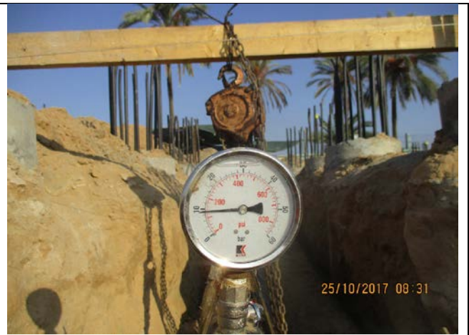
Photo No.12.2: Filtrated water to cartridge filter underground pipe DN 315 mm SDR 11 pressure test completion. Date: October 25, 2017
