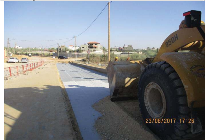
Photo No.57: Surface restoration work at interlock tile area (aggregate base). Date: August 23, 2017
