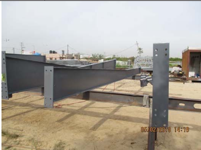
Photo No.07: Preparation works for steel structure before epoxy painting Date: February 05, 2018
