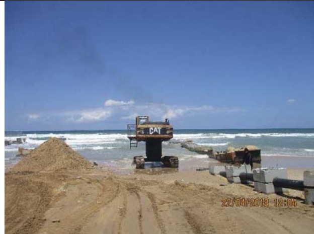
Photo No.33: Backfilling works with filter gravels around outfall pipeline. Date: April 22, 2018
