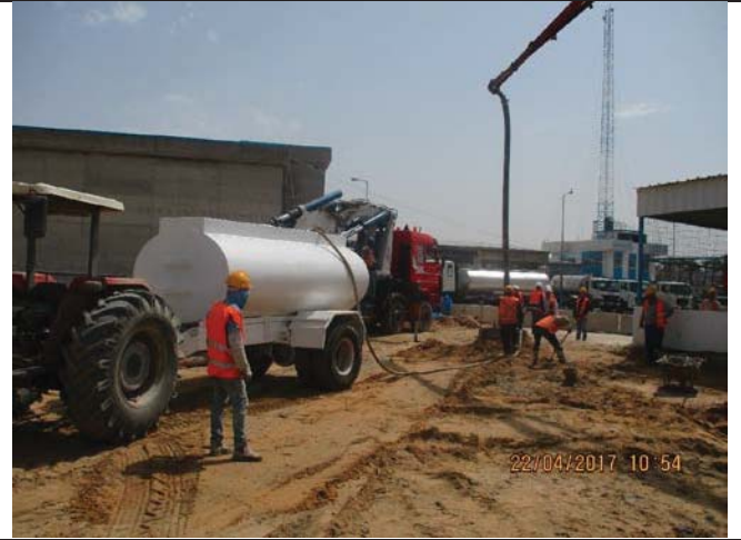
Photo No.18: Drilling control activities during piles construction at the RO building.
