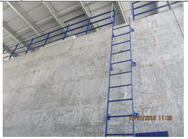
Photo No.10: Handrail and ladder installation for raw water/backwash tank Date: January 17, 2019
