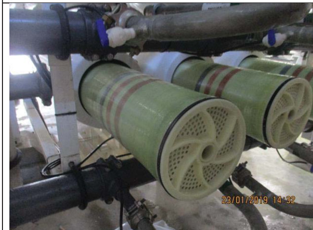
Photo No.17: Loading the membrane for the 2 nd train of the 1 st pass Date: January 23, 2019
