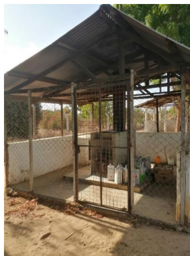
The incinerator at Gongoni Health Centre
