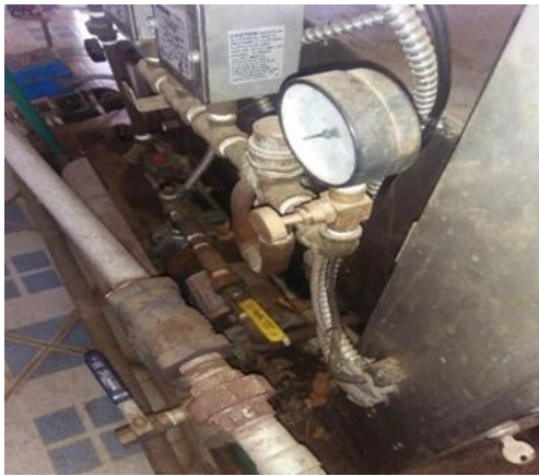
The faulty Steam generator
