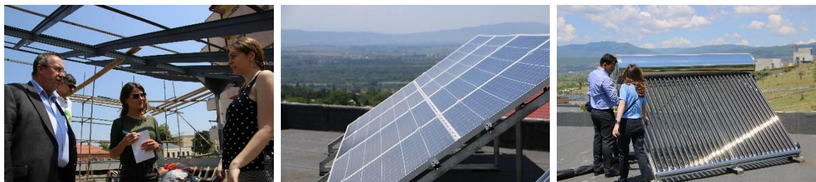
Rooftop Solar PV System in Telavi and Solar PV Water Heating System in Saguramo
