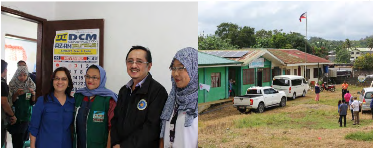
MinDA Secretary Alonto visits the solar rooftop installed at Sugod Health Station and interacts with barangay health workers. Photo credit by B-LEADERS.
