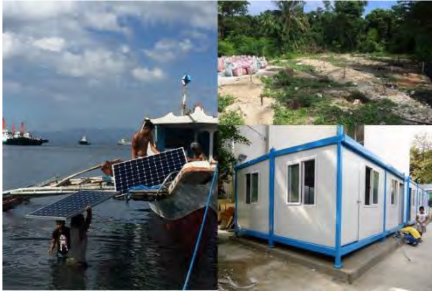
The solar PV micro-grid project in Isla Verde not only provided resilient and reliable power to a village of the island but also tested and defined requirements on logistics, business arrangements, regulatory approvals, and multisectoral implementation. Photo credit by B-LEADERS.
