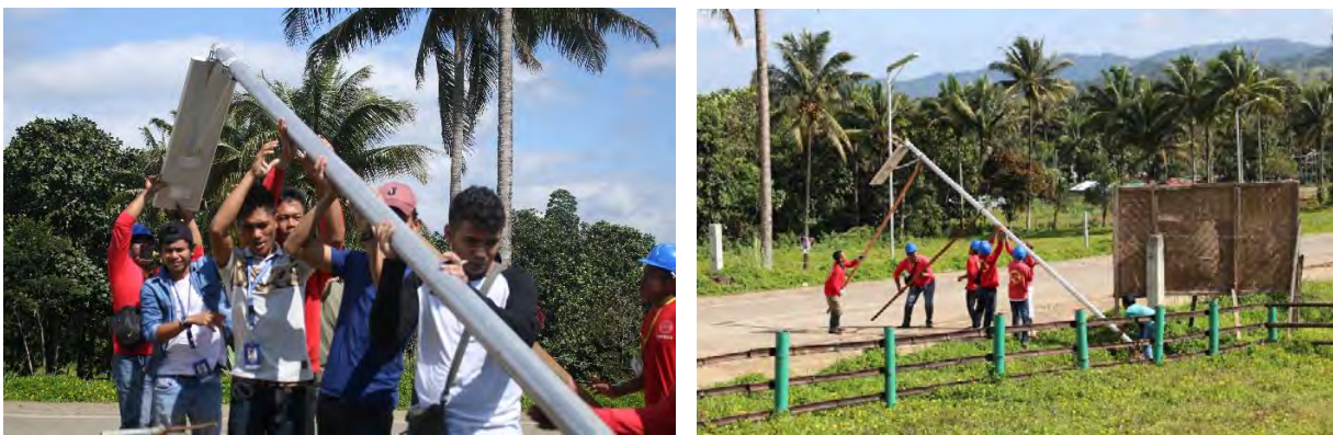
(Left) B-LEADERS’s installation crew demonstrates how to install a solar streetlight that OSY participants (Right) replicated during the trainings. Photo credit by B-LEADERS.
