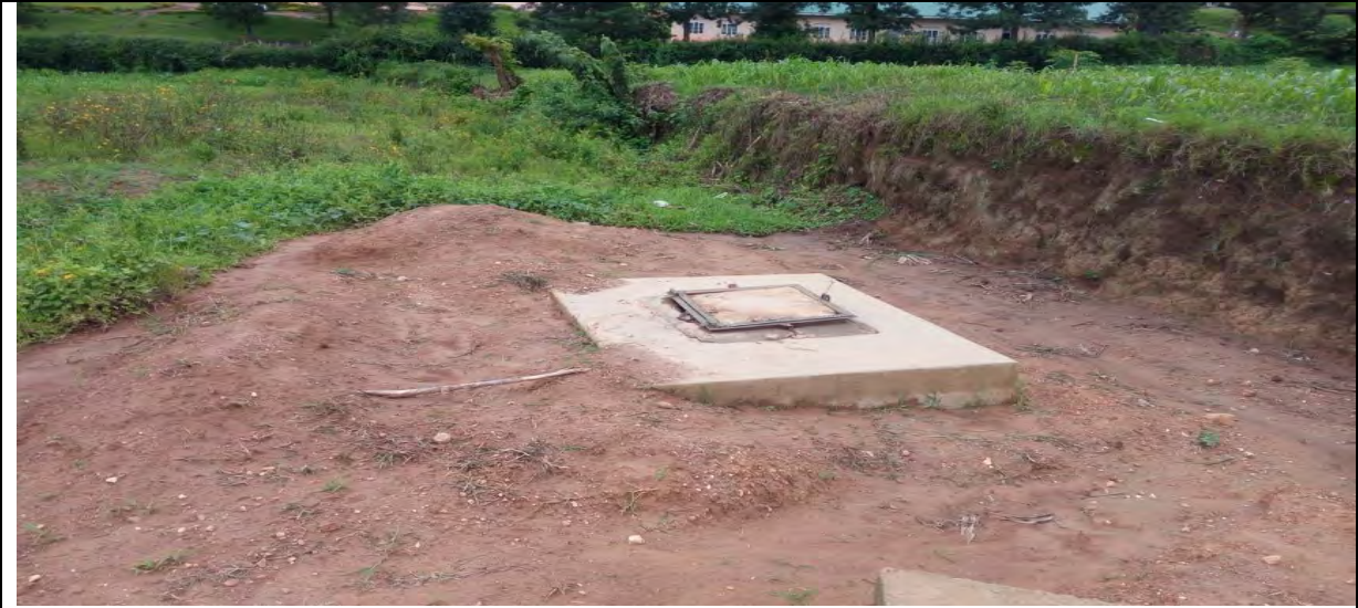
Figure 13: A septic tank at one of the health facilities
