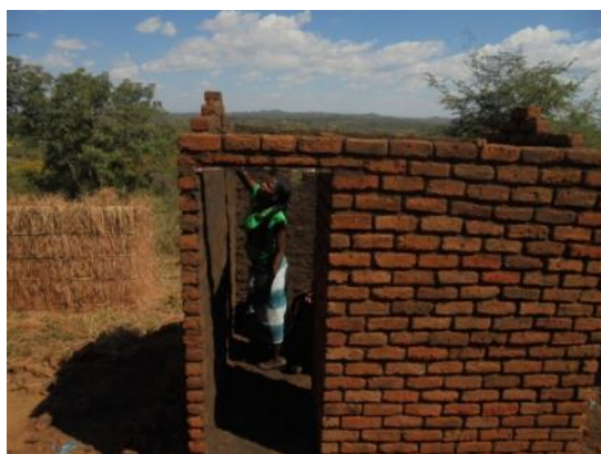
Jali community member putting finishes to one of the newly constructed pit latrines
