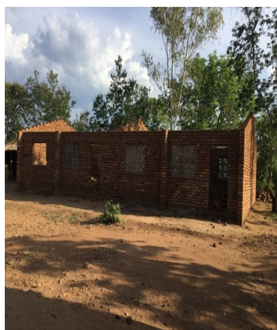
A two-block classroom structure that has been constructed by communities at Chisongwe Primary School in Balaka district.
