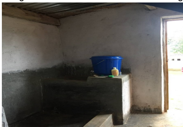
The newly constructed girls' changing room at Satema Primary school in Zomba district
