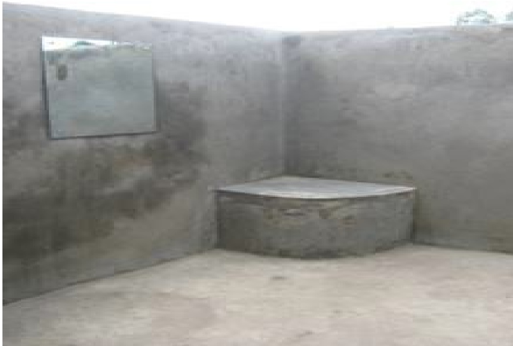
Figure 7.1: Inside the MHM Room—a stand for water bucket, a mirror for checking appearance and clothes after changing pads
