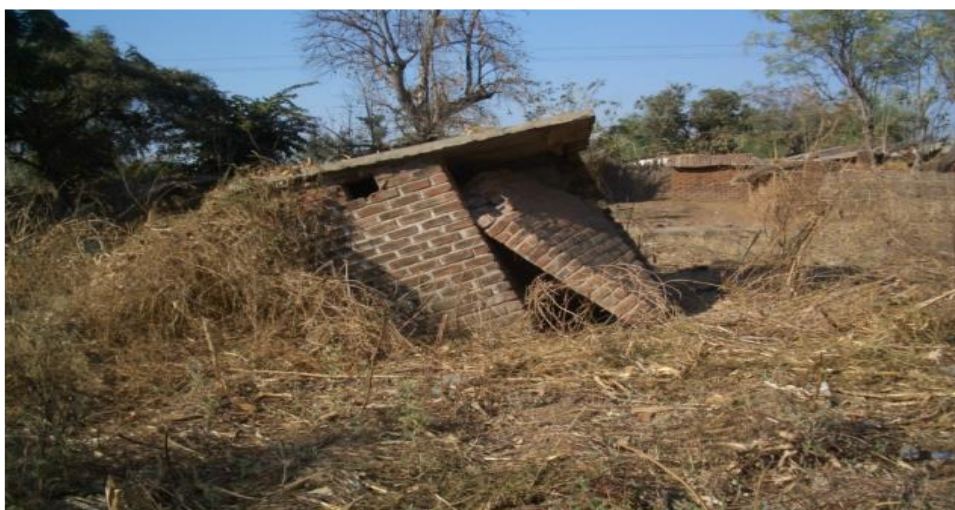
Figure 2:2: A collapsed latrine.
