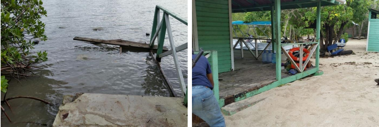
Photo 6. Damage from Hurricane Irma to infrastructure of the Marine Mammal Sanctuary of Estero Hondo, September 7, 2017.
