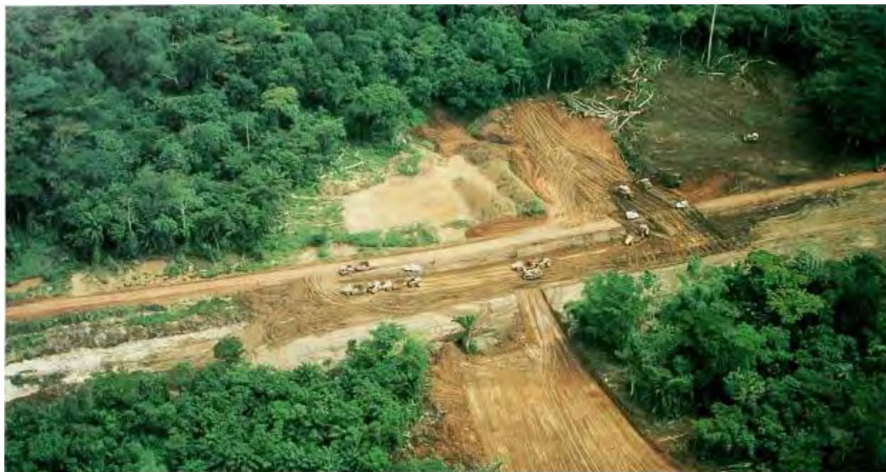
FIGURE 5. Road Construction Through a Forest in the Democratic Republic of the Congo
