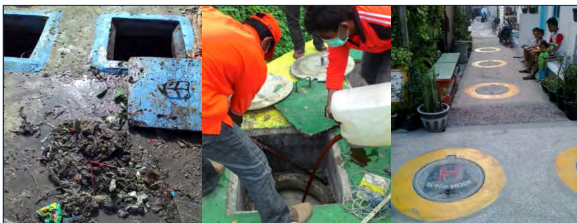
UPTD-PAL staff in Gresik assist a communal sanitation CBO in the maintenance of its infrastructure.
