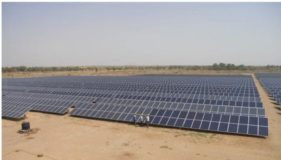
Figure 5: Utility-scale solar PV applications
