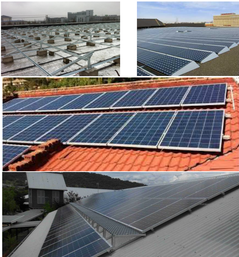
Figure 23: Different rooftop array mounting structures
