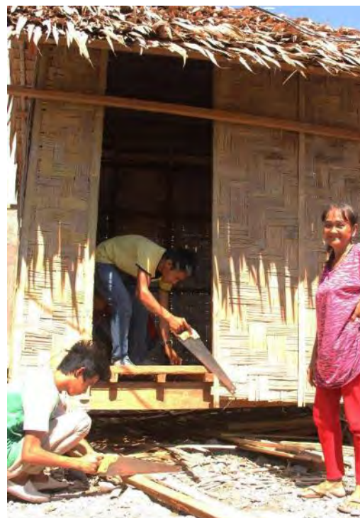
Herminia Sebastian (right), 58 years old, found her home leveled to the ground after the siege in Zamboanga in 2013. Without a home, she temporarily stayed in Brgy Guiwan with one of her children. But the MYDev trainees on carpentry built her a new home as part of their community service project.
