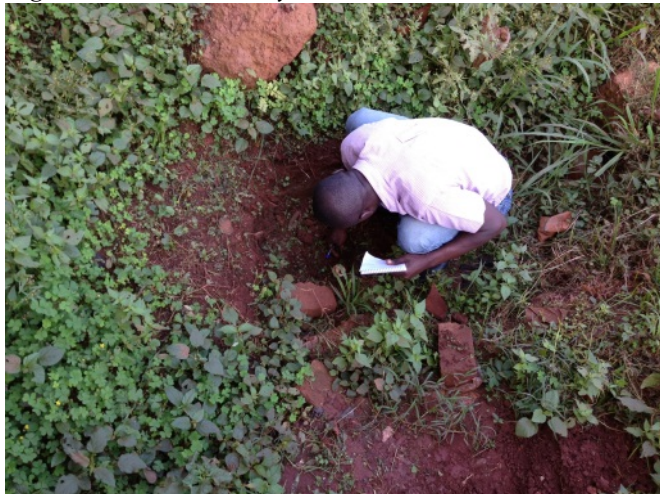
Figure 4.2.2 Meter nearly buried .
