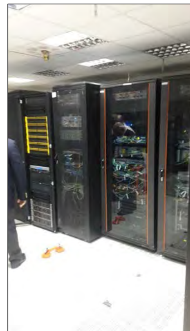
JCD server room
