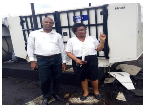
New generator purchased by facility management to support the PCR lab
