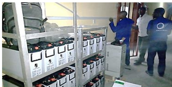
Inverter Installed at UCTH PCR Lab
