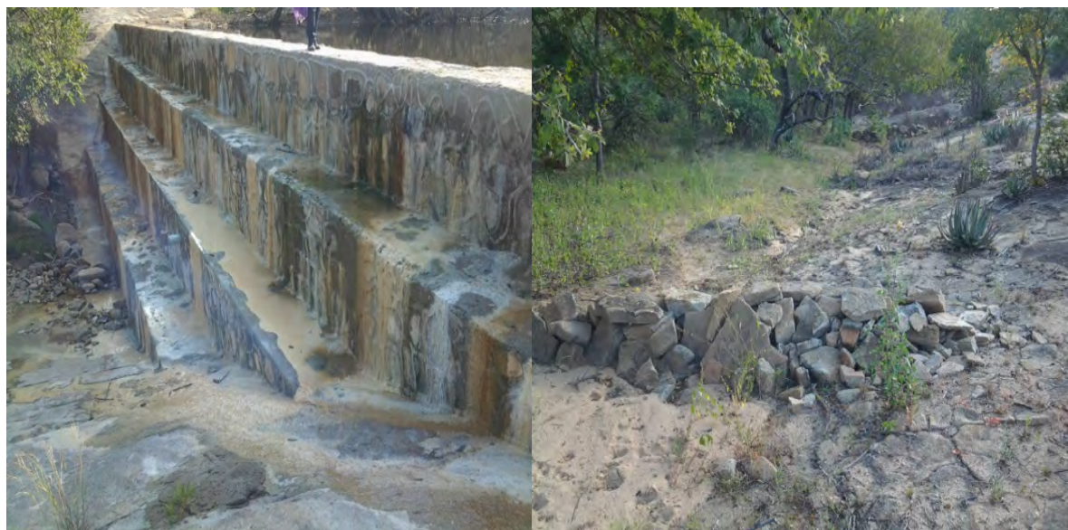
Photo 5: (Left) Mbuyaneweir dam wall, Gwanda. Photo 6: (Right) Silt trap in the catchment area of Mbuyane dam.
