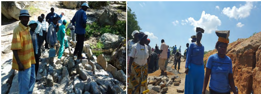
Photo 1: (Left) Weir dam wall under construction at Simbumbu ward, Chivi. Photo 2: (Right) Women carrying stones at dam site in ward 19, Buhera and others working in the background. Workers have no protective clothing in both cases.
