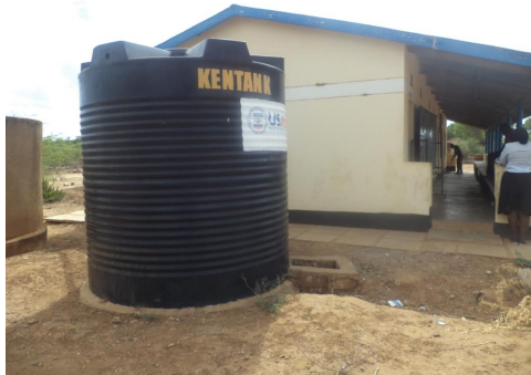
Water tank at Chewele Dispensary
