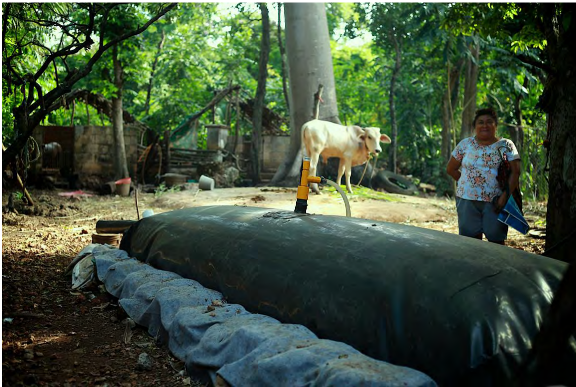
Image 1: Tubular modular polyethylene biodigester installed in a backyard farm by Sistema Biobolsa in partnership with the W.K. Kellogg Foundation and IRRI Mexico (2014).
