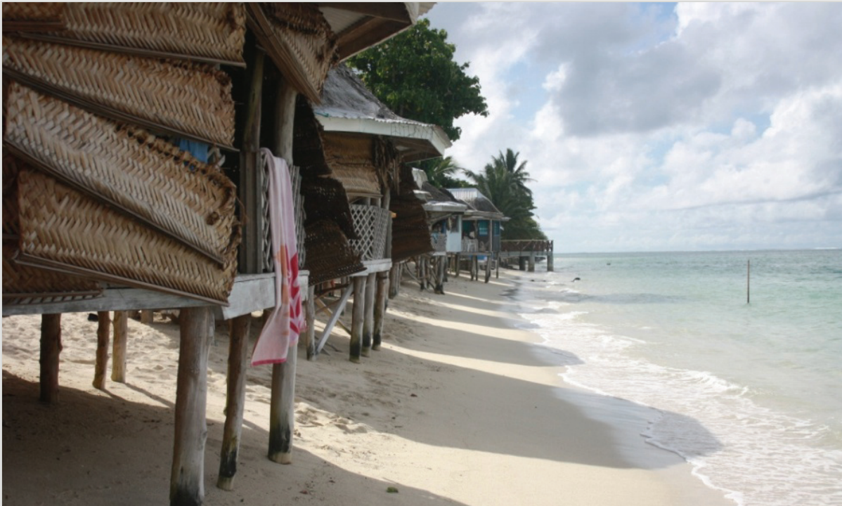
Samoa: Sea level rise is causing beaches to slowly become eroded, undermining the foundations of village huts foundations to be undermined. The only adaptation option is to relocate the villages inland.
