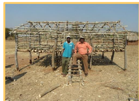
Figure 1: Benard Ngoma displays the goat housing established with field supervisors and lead farmers under Mawa Project. The previous open-air structure did not support animal husbandry practices nor promote livestock health.
