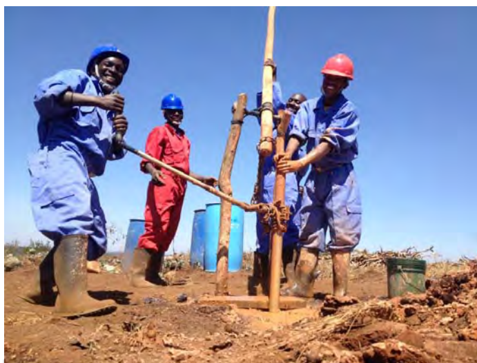
Photo by Fintrac Inc. SHIPO technicians drill to complete the construction of shallow wells under the USAID-TAPP partnership.
