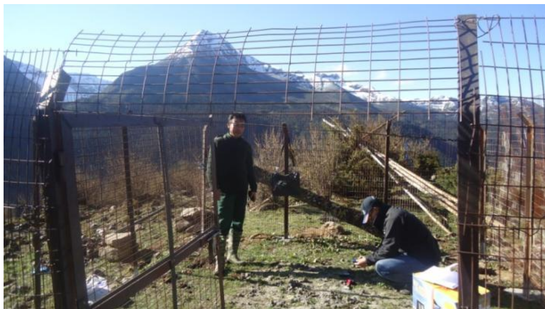
Activity 1.2.5: Installation of the first high-altitude (4033 m) hydro-meteorological station in Wangchuck Centennial Park at Khangdang, Bhutan.
