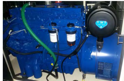
The new generator will power classrooms and computer lab at AMDCM. June 2015
