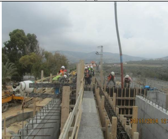
Photo Date- 24 th of November, 2014: Start and finish casting concrete for balance tank wall (Section E2).
