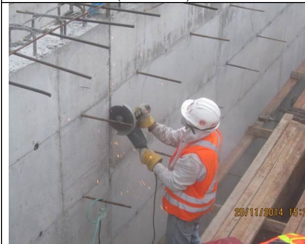
Photo Date- 25 th of November, 2014: Removing expansion joints and surface preparation for re-filling.
