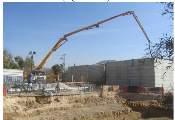
Photo date- 13 th of November, 2014: Start and finish casting concrete for balance tank wall (Section E1).
