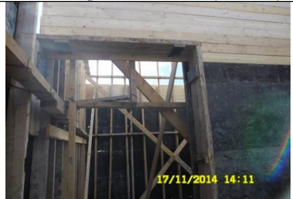
Photo date- 17 th of November, 2014: Continue formwork for living quarter building walls.
