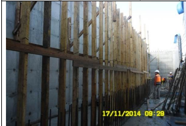
Photo date- 17 th of November, 2014: Start formwork for balance tank wall (Section E2).
