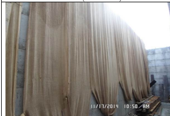
Photo date- 17 th of November, 2014: Continue concrete curing of balance tank wall (Section E2).
