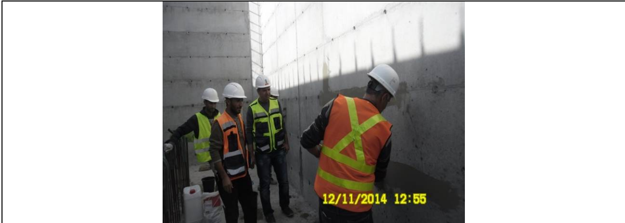
Sanur Well: Preparing a sample of balance tank wall surface repair with the present of FOSROC representative
