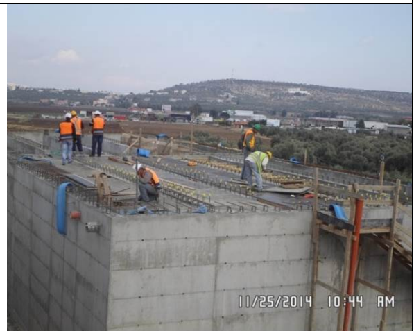
Photo Date- 25 th of November, 2014: Continue formwork for balance tank elevated slab.
