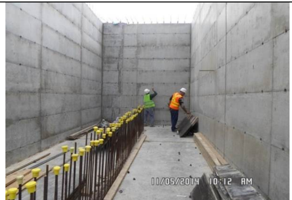
Photo Date- 5 th of November, 2014: Balance tank internal walls -tie rods holes repair.
