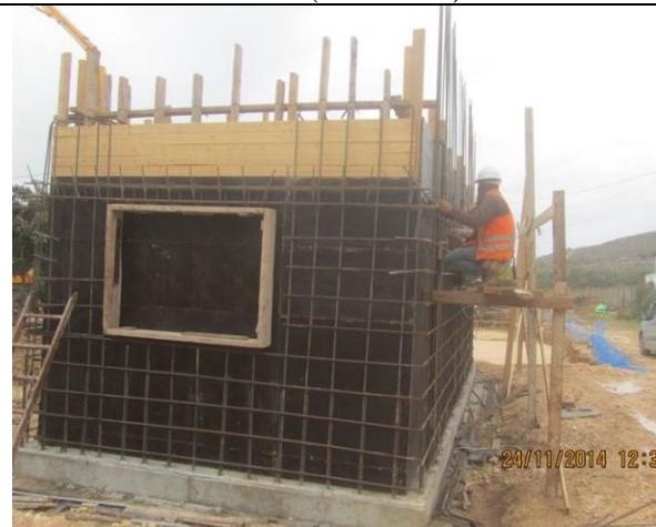
Photo Date- 24 th of November, 2014: Continue formwork and steel reinforcement steel for living quarter.
