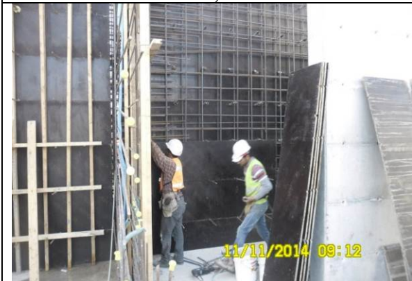
Photo date- 11 th of November, 2014: Continue steel reinforcement and formwork for balance tank wall (Section E1).
