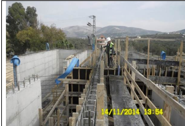
Photo date- 14 th of November, 2014: Start concrete curing of balance tank wall (Section E1).
