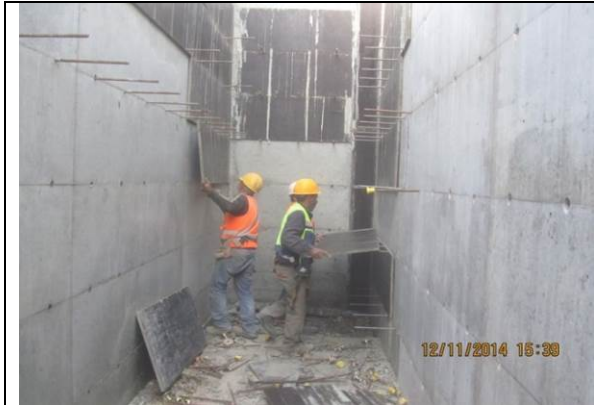
Photo date- 12 th of November, 2014: De-shuttering of formwork for balance tank wall (Section E2).
