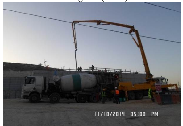
Photo date- 10 th of November, 2014: Casting concrete for balance tank wall (Section E2).
