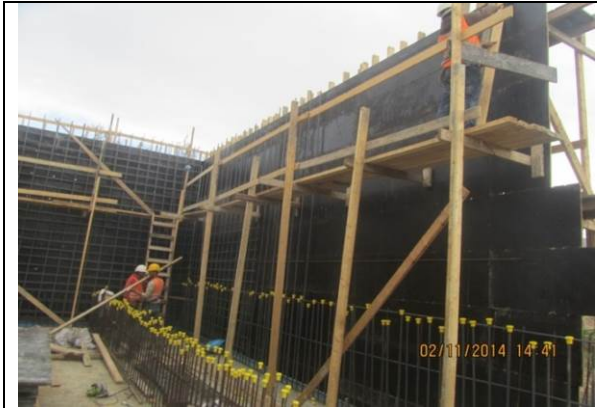
Photo Date- 2 nd of November, 2014: Continue formwork and steel reinforcement for balance tank wall (Section D).
