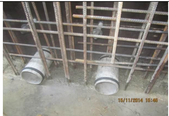
Photo date- 15 th of November, 2014: Installation of 6" stainless steel wash down opening on balance tank wall (Section E1).
