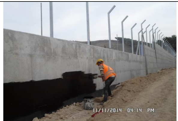
Photo date- 11 th of November, 2014: Applying damp-Proof (Nito-Proof 30) for the external side of the retaining wall.
