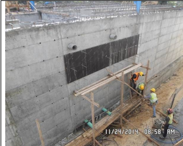
Photo Date- 24 th of November, 2014: Finish de-shuttering of formwork for balance tank wall (Section. E1).
