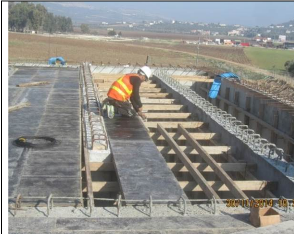
Photo Date- 30 th of November, 2014: Continue formwork for balance tank elevated slab.
