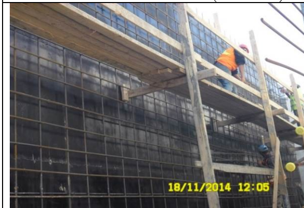
Photo date- 18 th of November, 2014: Continue formwork and steel reinforcement for balance tank wall (Section E2).
