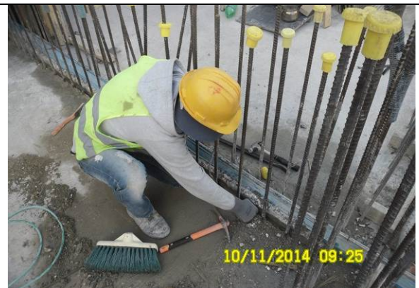
Photo date- 10 th of November, 2014: Repairing works of the kicker of balance tank wall (Section E1).
