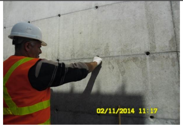
Photo Date- 2 nd of November, 2014: Balance tank internal walls-repairing tie rods holes.
