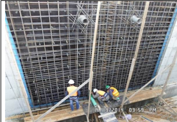
Photo date- 19 th of November, 2014: Fixing 8” thimbles for overflow pipes and 6” thimbles for equalization pipes for balance tank wall-(Section E1).
