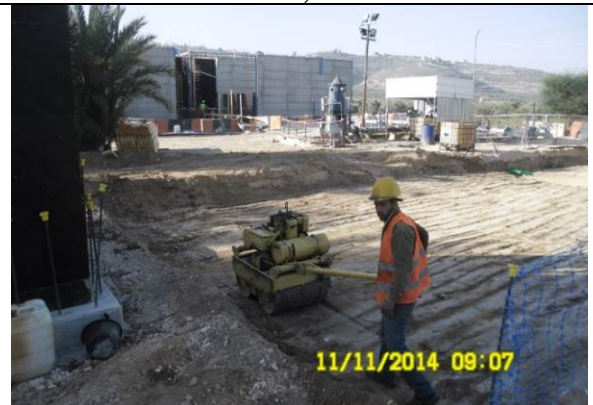
Photo date- 11 th of November, 2014: Start and finish compaction of substrata for chlorination room foundation.
