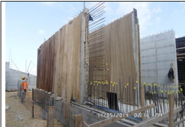
Photo Date- 5 th of November, 2014: Concrete curing of balance tank wall (Section C).
