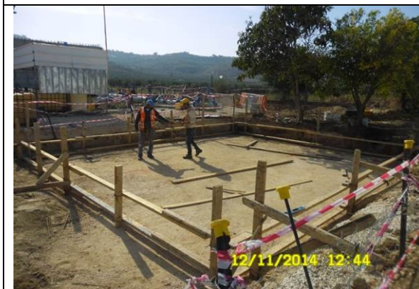
Photo date- 12 th of November, 2014: Start formwork for electrical metering room foundation.
