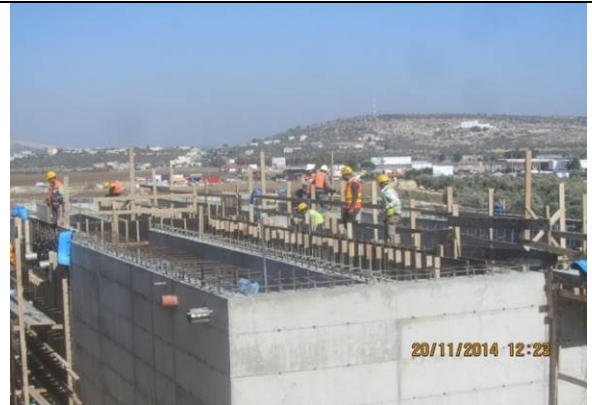
Photo date- 20 th of November, 2014: Finish formwork and steel reinforcement for balance tank wall (Section E1).
