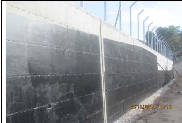
Photo date- 12 th of November, 2014: Finish applying damp-Proof (1st layer) on the external side of the retaining wall, from St.78+800 to St.140+200.
