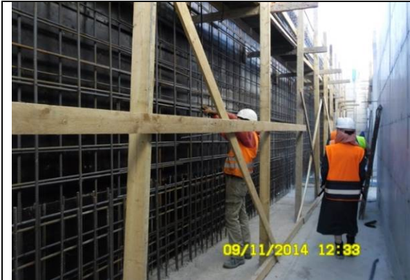
Photo Date- 9 th of November, 2014: Continue steel reinforcement and formwork for balance tank wall (Section E1).
