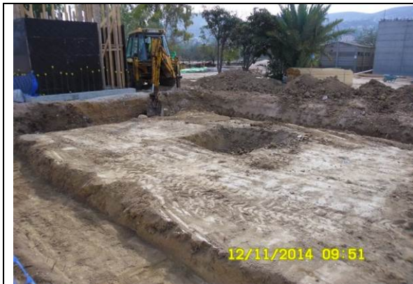
Photo date- 12 th of November, 2014: Start and finish excavation for chlorination room footing.
