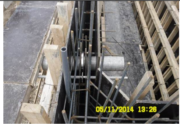
Photo Date- 5 th of November, 2014: Installation of stainless steel pipes for balance tank wall (Section D).
