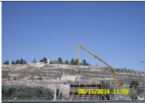
Photo Date- 6 th of November, 2014: Casting concrete for balance tank wall (Section D).
