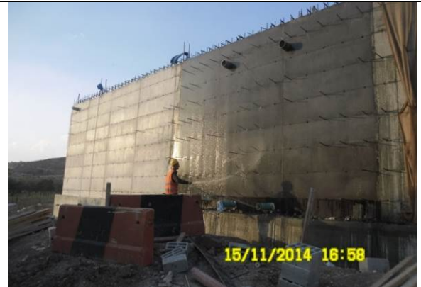
Photo date- 15 th of November, 2014: Continue concrete curing of balance tank wall (Section E1).
