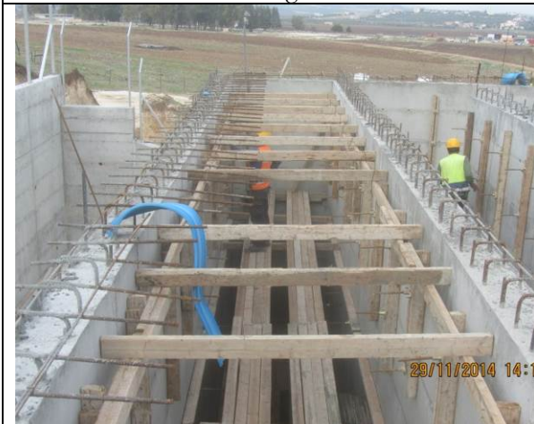
Photo Date- 29 th of November, 2014: Continue formwork for balance tank elevated slab.
