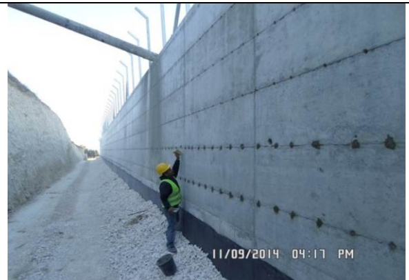
Photo date- 9 th of November, 2014: Continue repairing tie rods holes- external side of the retaining wall (2 nd lift).
