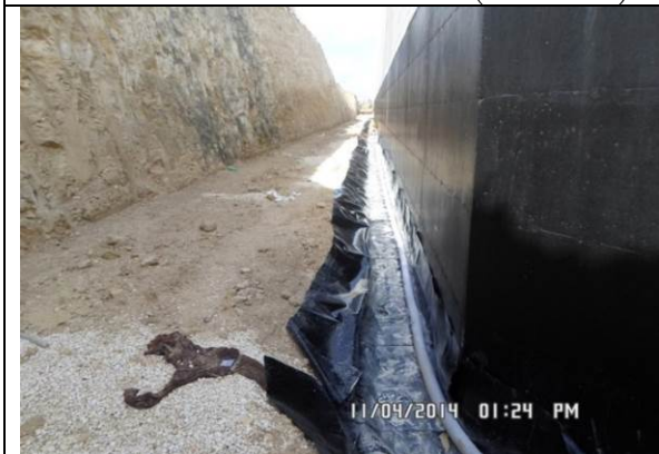
Photo Date- 4 th of November, 2014: Finishing installation of underdrain system behind retaining wall.
