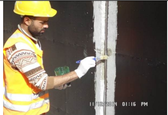
Photo date- 12 th of November, 2014: Start and finish filling Thoflex-600 in the expansion joints of the retaining wall.
