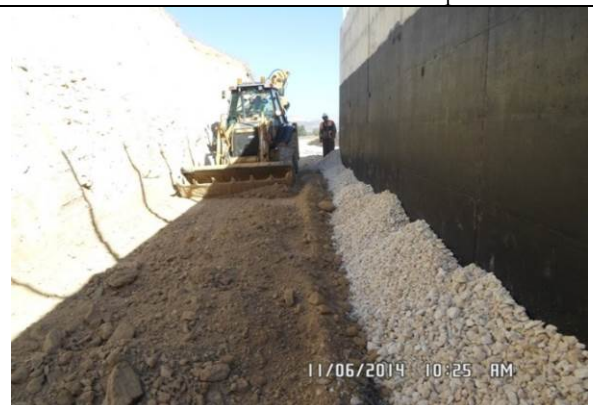
Photo Date- 6 th of November, 2014: Continue backfilling of drain rock behind retaining wall.
