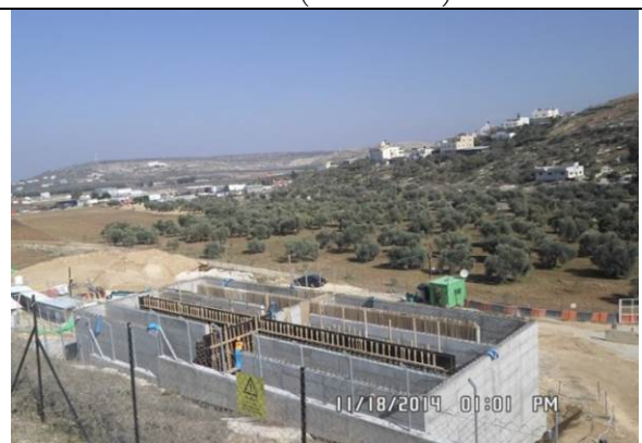
Photo date- 18 th of November, 2014: Continue formwork and steel reinforcement for balance tank wall (Section E1).
