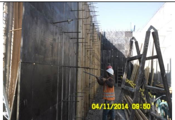
Photo Date- 4 th of November, 2014: Formwork de-shuttering of balance tank wall (Section C).
