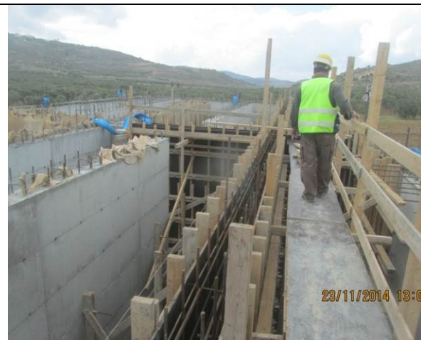
Photo Date- 22 nd of November, 2014: Continue formwork and steel reinforcement for balance tank wall (Section E2).
