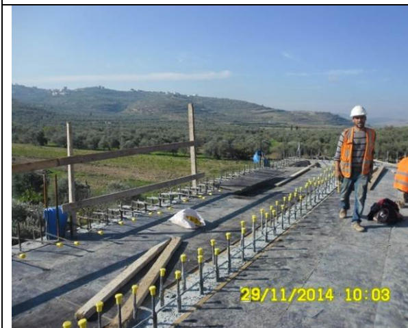
Photo Date- 29 th of November, 2014: Continue formwork for balance tank elevated slab.
