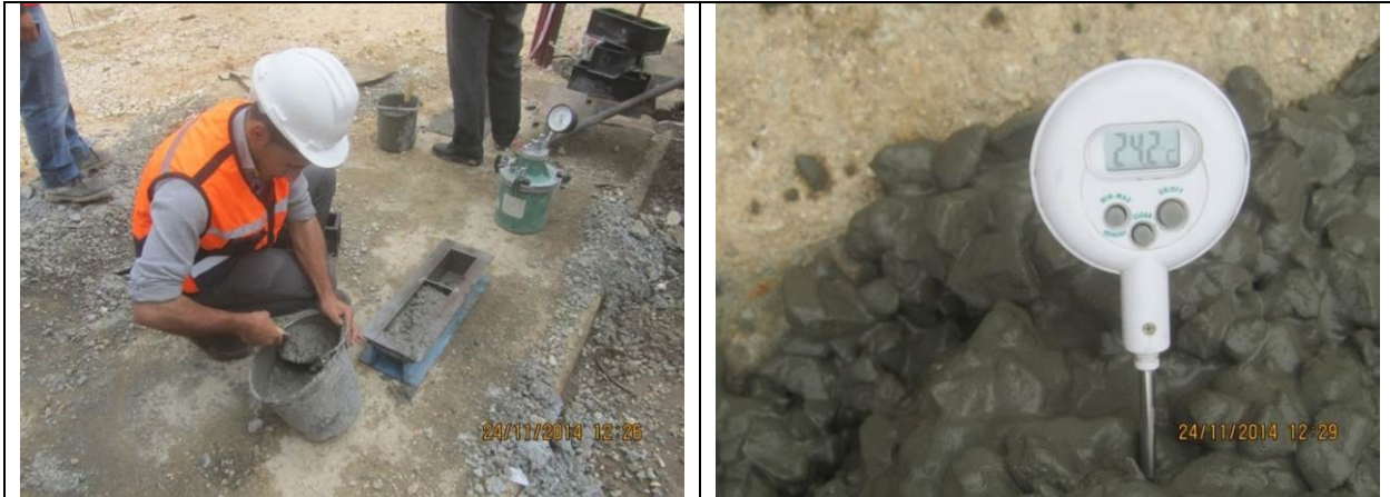
Sanur Well: Collecting concrete samples and field tests for balance tank wall (Section E2)
