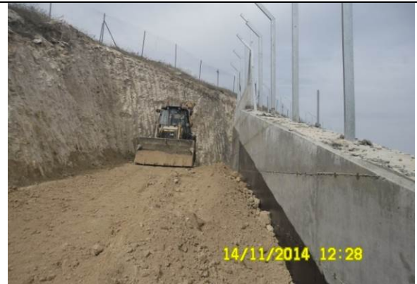
Photo date- 14 th of November, 2014: Continue backfilling and compaction behind retaining wall.
