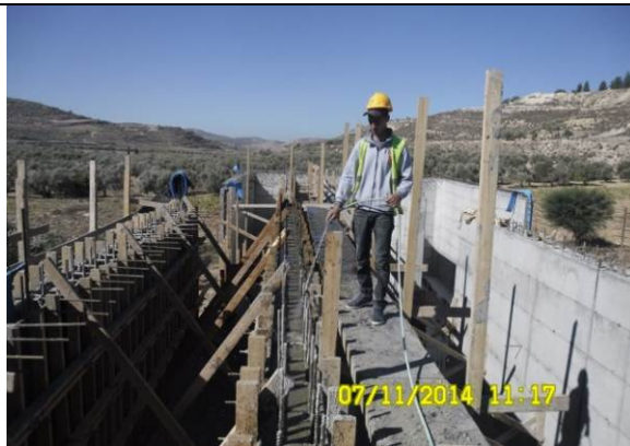
Photo Date- 7 th of November, 2014: Concrete curing of balance tank wall (Section D).
