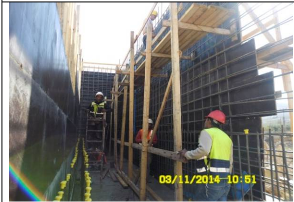
Photo Date- 3 rd of November, 2014: Continue formwork and steel reinforcement for balance tank wall (Section D).
