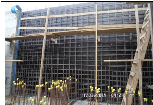
Photo Date- 3 rd of November, 2014: Starting steel reinforcement of balance tank wall (Section E2).
