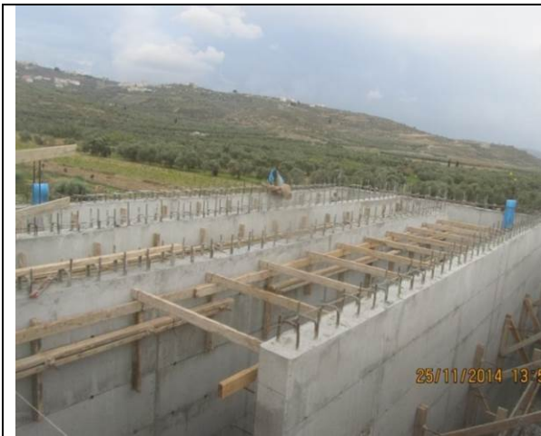
Photo Date- 25 th of November, 2014: Start formwork for balance tank elevated slab.
