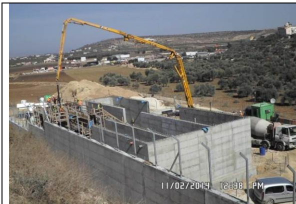
Photo Date- 2 nd of November, 2014: Casting concrete for balance tank wall (Section C).
