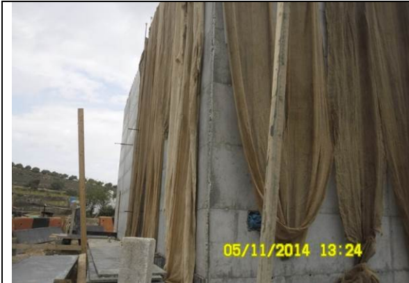
Photo Date- 5 th of November, 2014: Concrete curing of balance tank wall (Section C).
