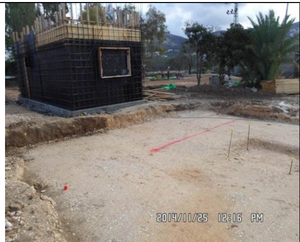
Photo Date- 25 th of November, 2014: Continue formwork and steel reinforcement steel for living quarter.
