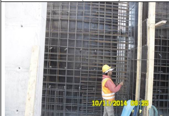
Photo date- 10 th of November, 2014: Continue steel reinforcement for balance tank wall (Section E1).
