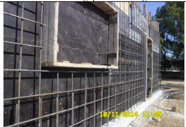
Photo date- 18 th of November, 2014: Continue formwork and steel reinforcement for living quarter building walls.
