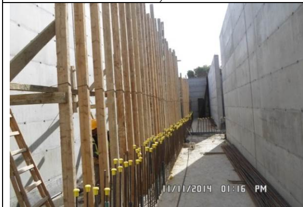
Photo date- 11 th of November, 2014: Formwork for balance tank wall (Section E1).
