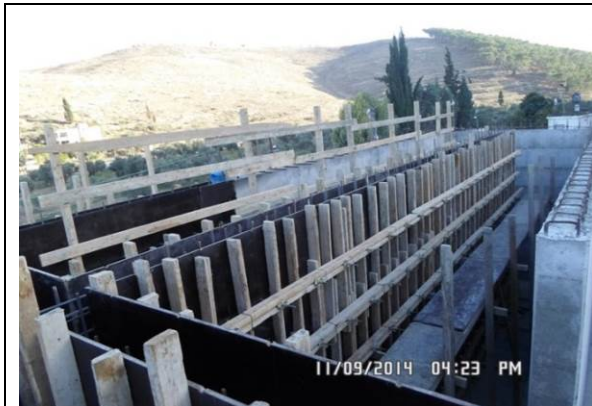
Photo Date- 9 th of November, 2014: Continue closing formwork of the balance tank wall (Section E2).
