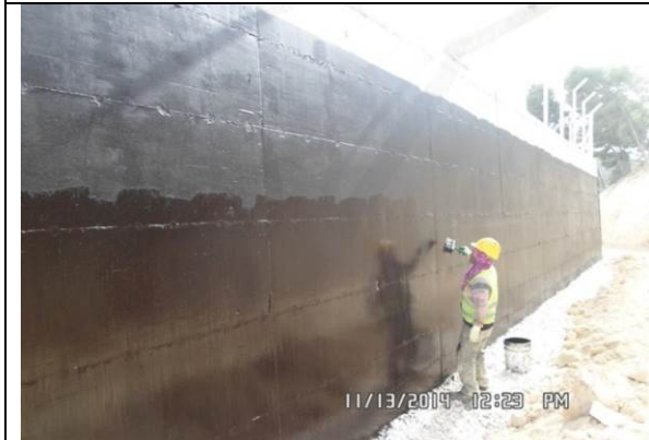
Photo date- 13 th of November, 2014: Start and finish applying damp-proof (2 nd layer) on the external side of the retaining wall, from St.78+800 to St.140+200.
