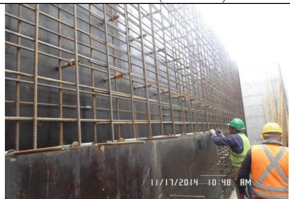
Photo date- 17 th of November, 2014: Continue formwork and steel reinforcement for balance tank wall (Section E1).
