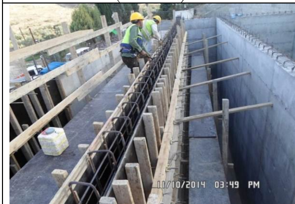
Photo date- 10 th of November, 2014: Finishing formwork closing for balance tank wall (Section E2).
