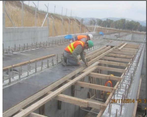
Photo Date- 24 th of November, 2014: Start formwork for balance tank elevated slab.
