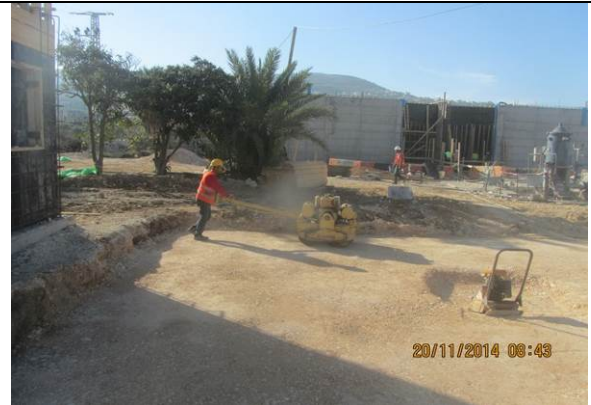
Photo date- 20 th of November, 2014: Finish spreading, leveling and compaction of base course layer under chlorination room foundation.
