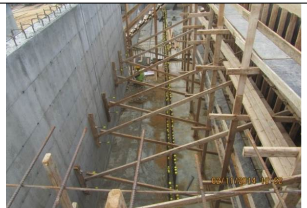
Photo Date- 2 nd of November, 2014: Starting formwork for balance tank wall (Section E2).
