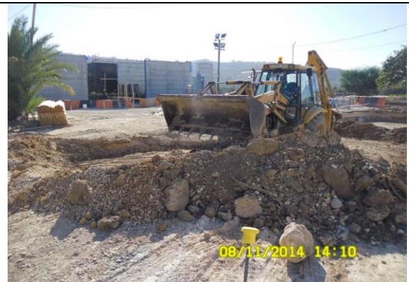
Photo Date- 8 th of November, 2014: Excavations of the chlorination room foundation to the required level.
