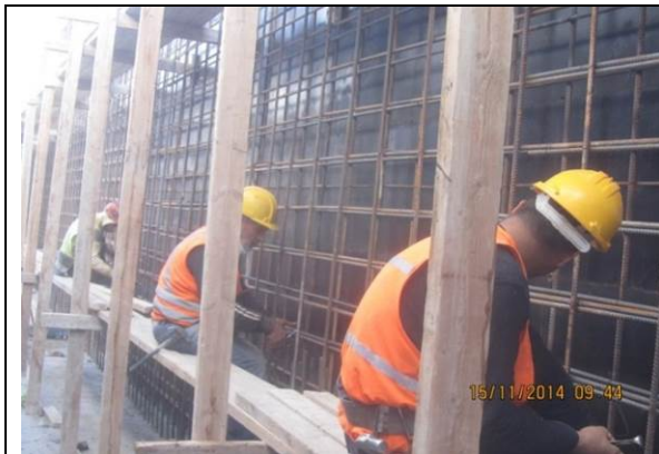
Photo date- 15 th of November, 2014: Continue formwork and steel reinforcement for balance tank wall (Section E1).
