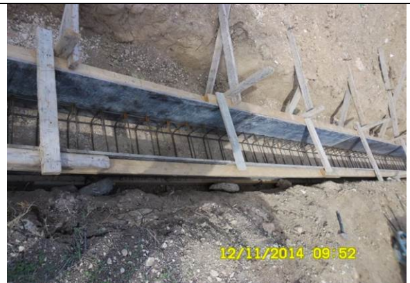
Photo date- 12 th of November, 2014: Continue steel reinforcement for fence wall foundation (Segment-AB).
