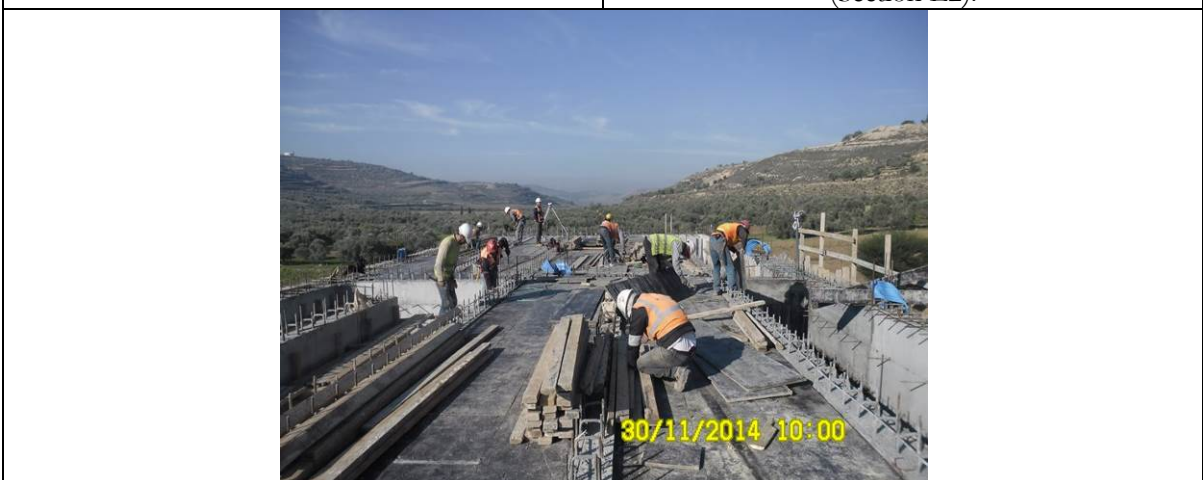
Photo Date- 30 th of November, 2014: Continue formwork for balance tank elevated slab.
