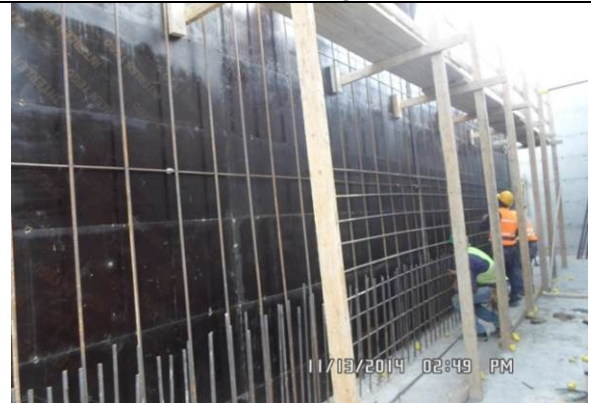
Photo date- 13 th of November, 2014: Continue formwork for balance tank wall (Section E1).
