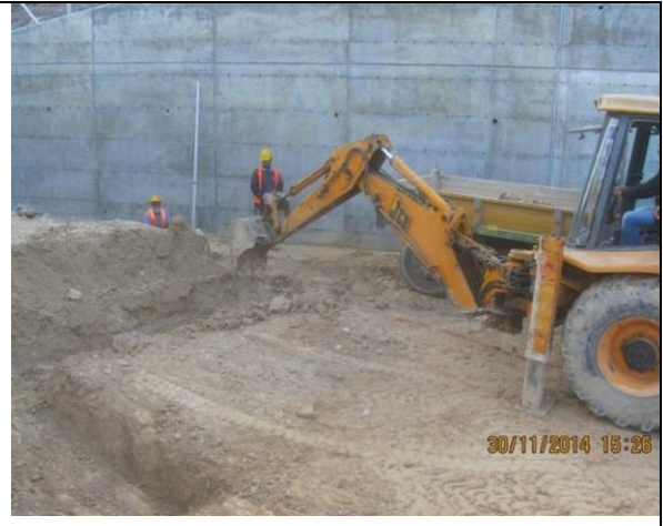
Photo Date- 30 th of November, 2014: Continue excavations for foundations of living quarter and electrical metering buildings.
