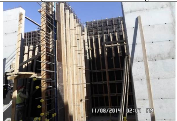
Photo Date- 8 th of November, 2014: Closing formwork of the balance tank wall (Section E2).
