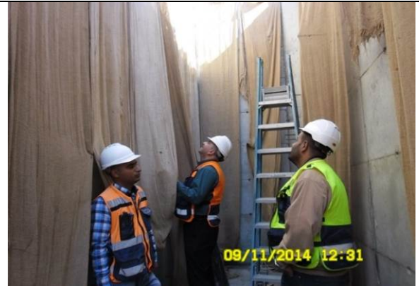
Photo date- 9 th of November, 2014: Continue concrete curing of balance tank wall (Section D).
