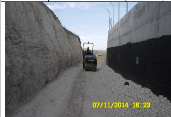
Photo Date- 7 th of November, 2014: Compaction of backfilled materials behind retaining wall.
