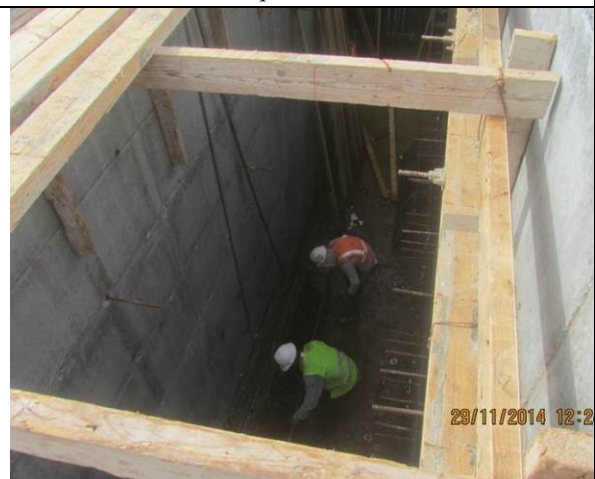
Photo Date- 29 th of November, 2014: Start formwork de-shuttering of balance tank wall (Section E2).
