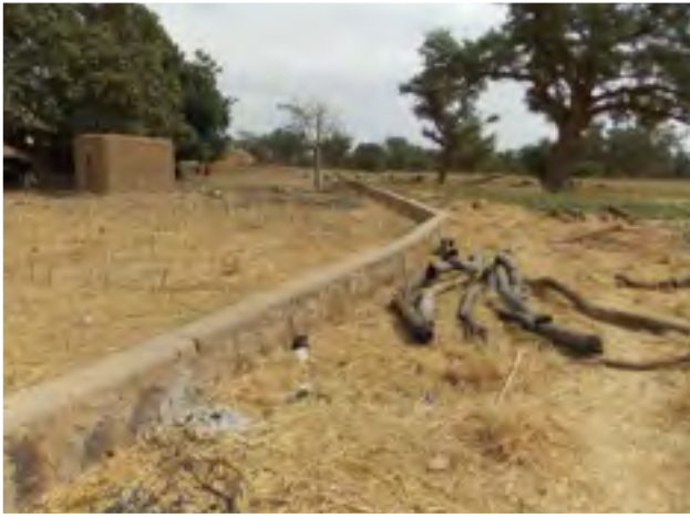
Digue (dike) created with Nema FFW that protects the village of Boumbam from seasonal flooding (Douentza) (November 2013) (Photographer: Isack Dolo).
