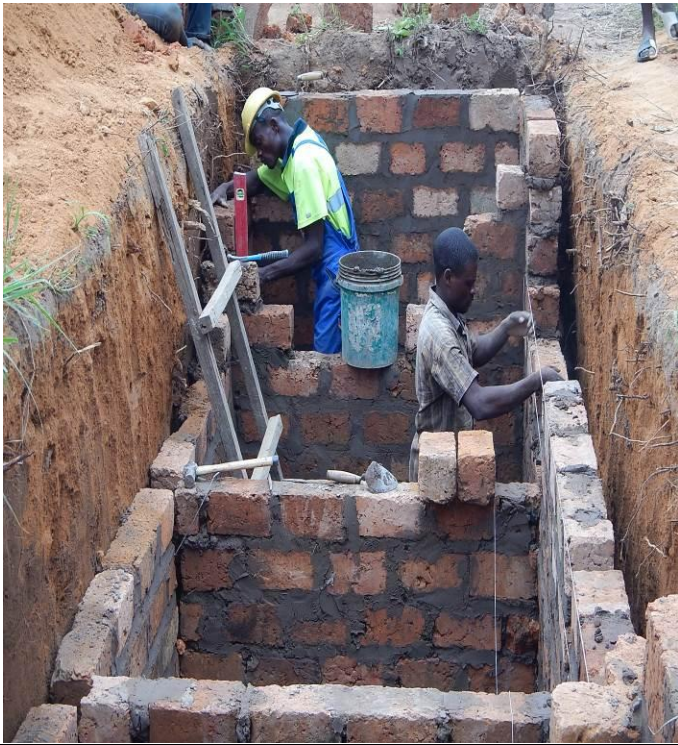
Photo of the site EP. PENSOLU (at the beginning of the construction)
