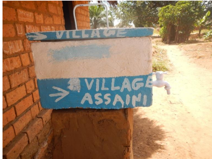
An installed hand wash system in the community
