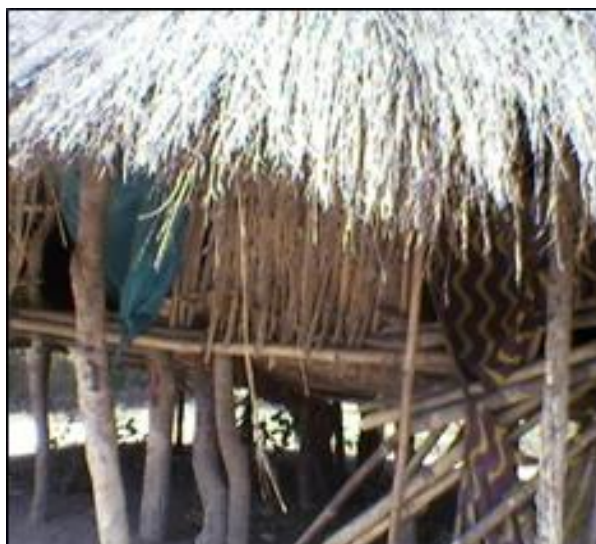
Caption: Magrete’s former house, in a state of major disrepair. Consent: Written consent was received from Magrete to use this photograph.
